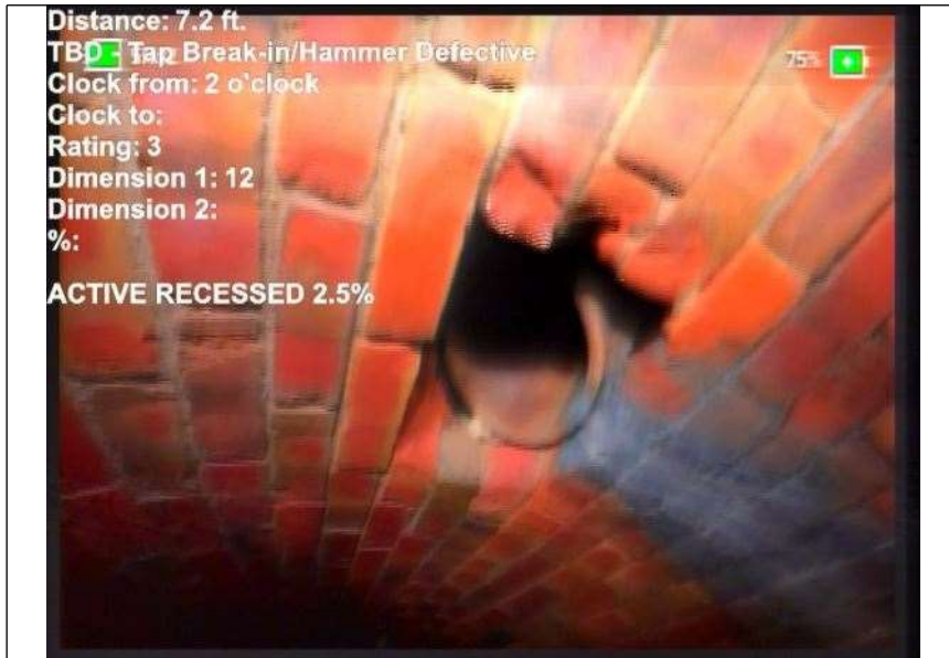
At: 7. TBD - Tap Break-in/Hammer Defective 1999998092 6514 ft. 2/. Joint: No ACTIVE RECESSED 2.5%
