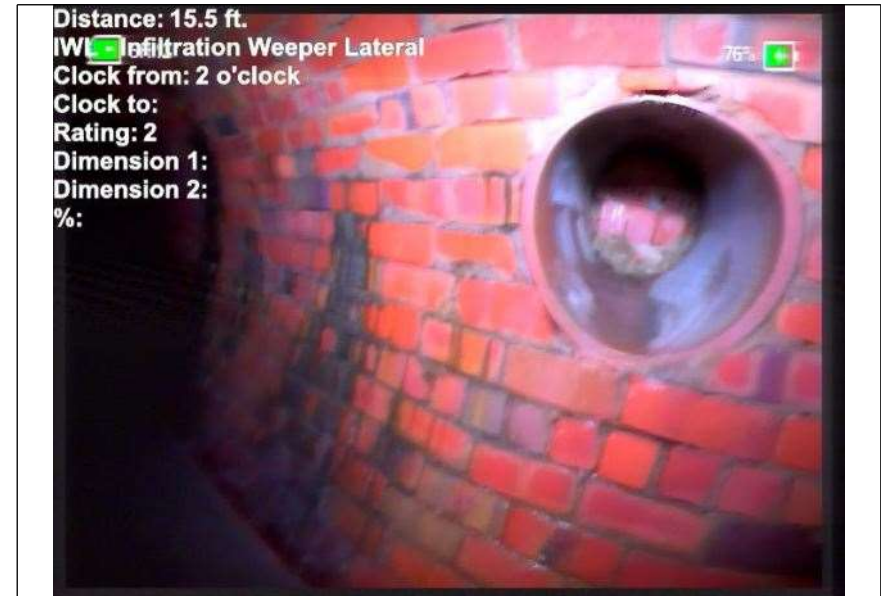
At: 15.5 ft. 2/. IWL - Infiltration Weeper Lateral Joint: No
