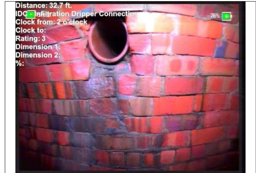
At: 32. IDC - Infiltration Dripper Connection 7000007629 395 ft. 2/.
