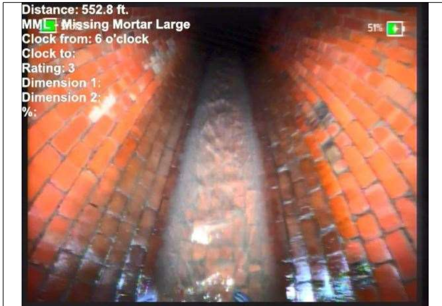
At: 552. 7999877929 MML - Missing Mortar Large 69 ft. 6/.
