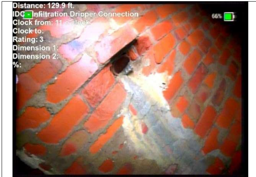
At: 129. IDC - Infiltration Dripper Connection 8999938964 84 ft. 11/.
