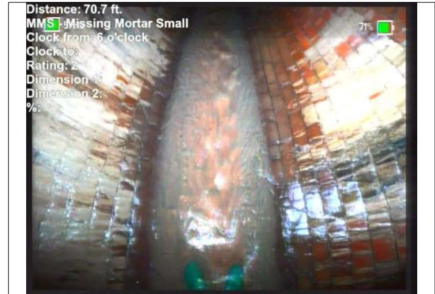
At: 70. 6999969482 MMS - Missing Mortar Small 422 ft. 6/. Joint: No
