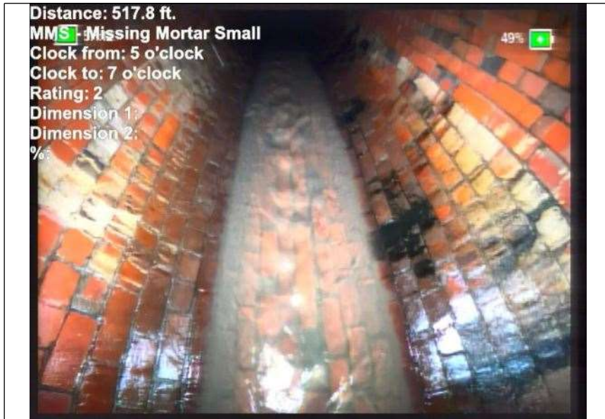
At: 517. MMS - Missing Mortar Small 7999877929 69 ft. 5/7
