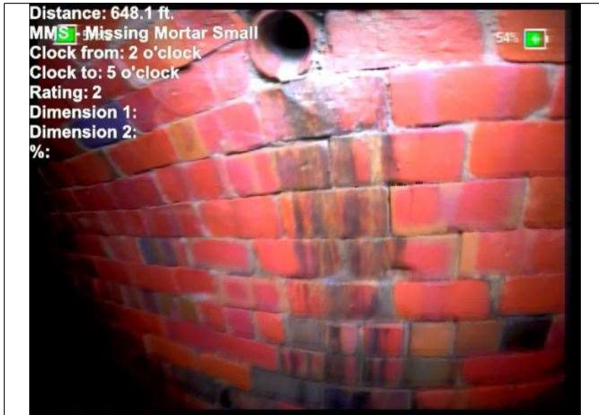
At: 648. MMS - Missing Mortar Small 0999755859 38 ft. 2/5
