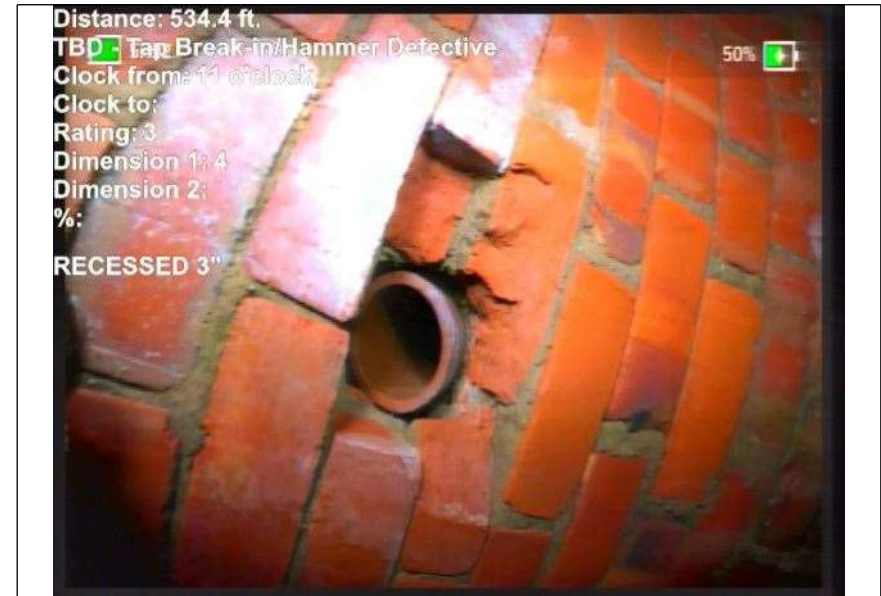
At: 534. TBD - Tap Break-in/Hammer Defective 400244140 63 ft. 11/.
