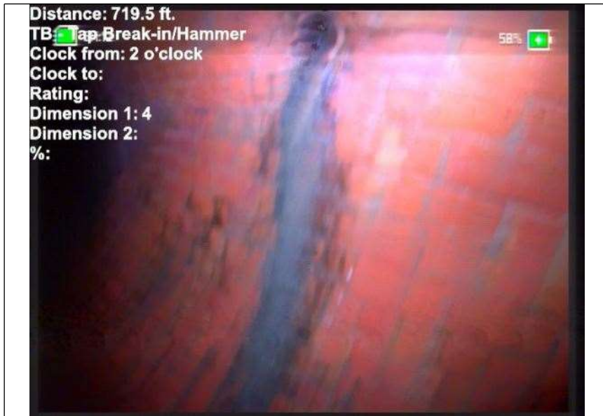
At: 719.5 ft. 2/. TB - Tap Break-in/Hammer
