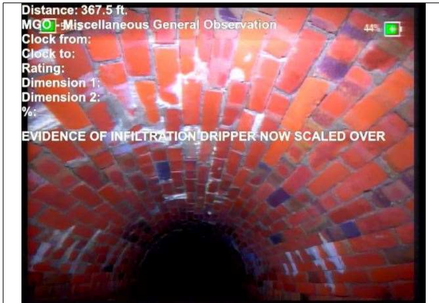
At: 367.5 ft. MGO - Miscellaneous General Observation Joint: No EVIDENCE OF INFILTRATION DRIPPER NOW SCALED OVER
