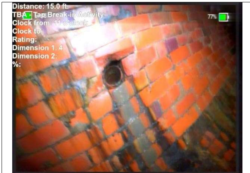
At: 15 ft. 11/. TBA - Tap Break-in Activity Joint: No
