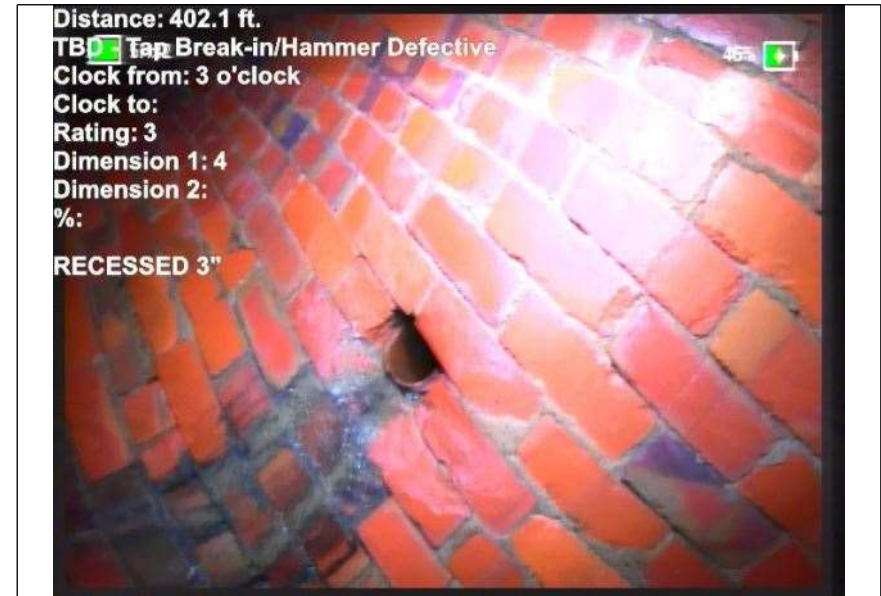
At: 402. TBD - Tap Break-in/Hammer Defective 1000061035 16 ft. 3/.
