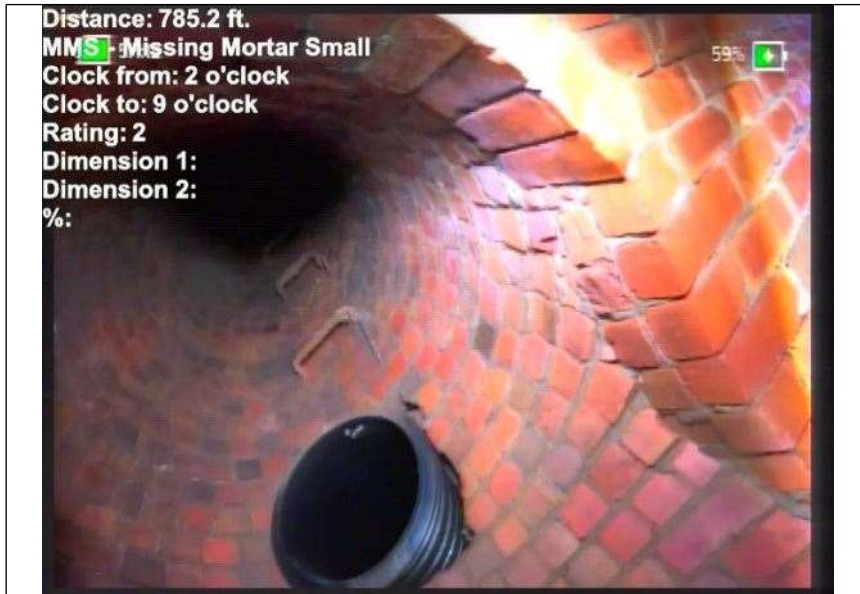
At: 785.1 ft. 2/9 MMS - Missing Mortar Small
