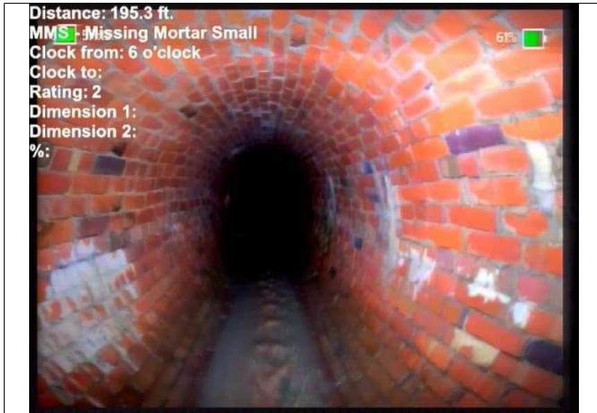
At: 195. MMS - Missing Mortar Small 3000030517 58 ft. 6/.
