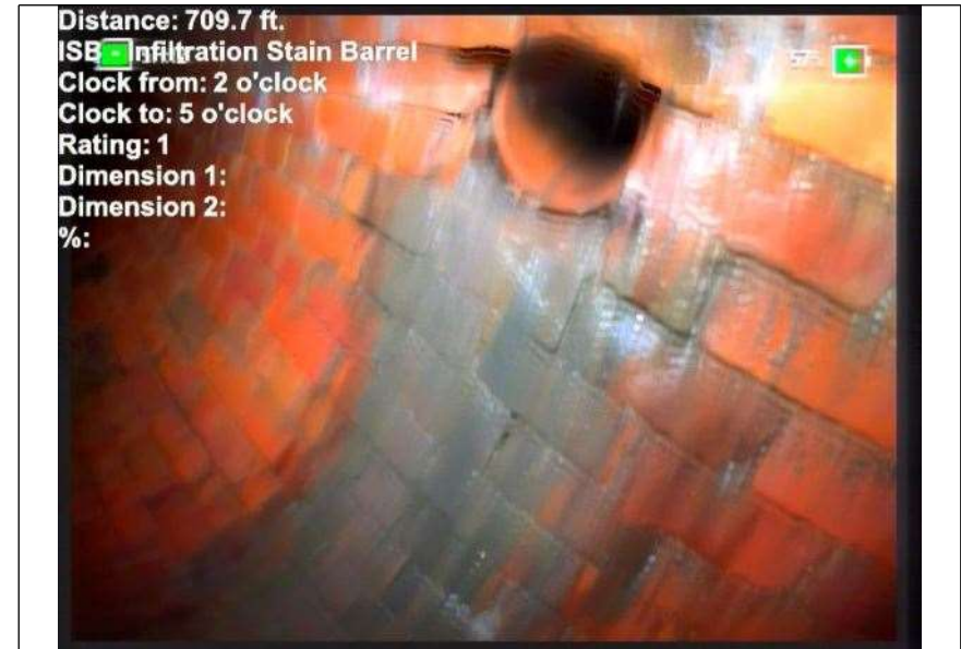
At: 709. 700122070 ISB - Infiltration Stain Barrel 31 ft. 2/5
