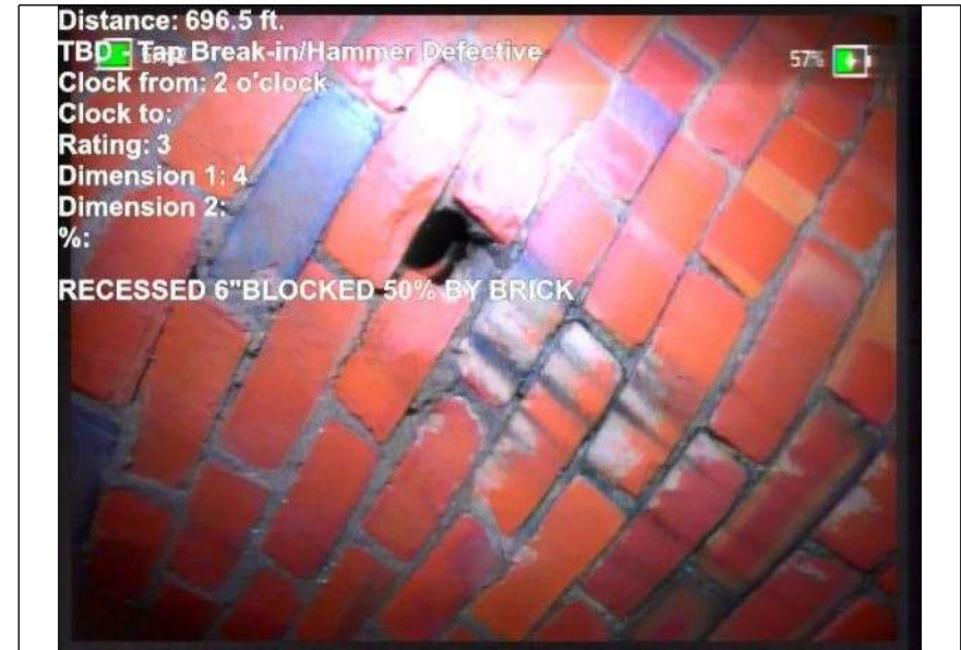
At: 696.5 ft. 2/. TBD - Tap Break-in/Hammer Defective Joint: No RECESSED 6"BLOCKED 50% BY BRICK
