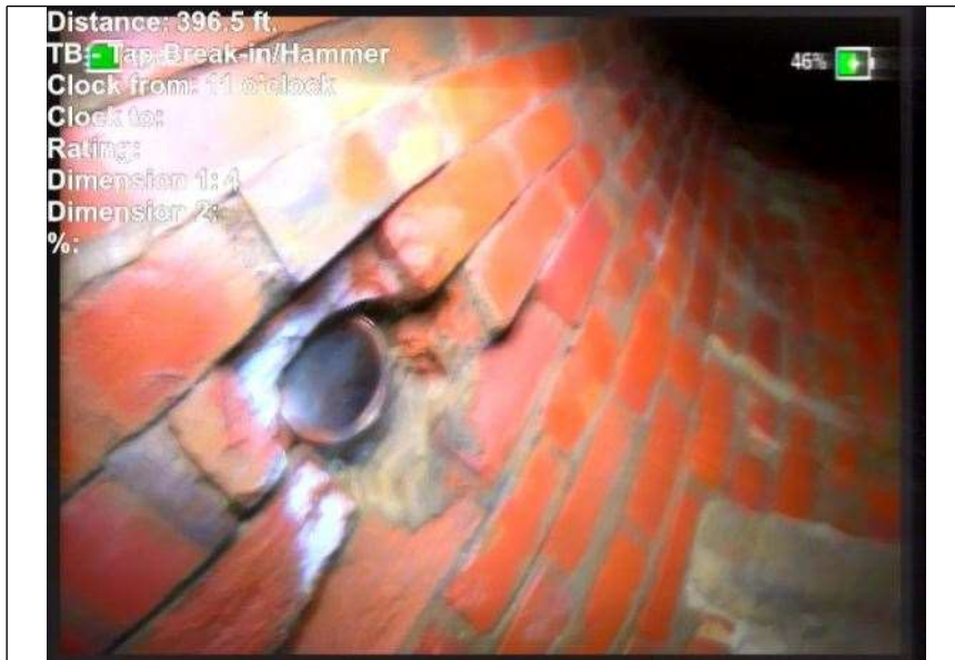
At: 396.5 ft. 11/. TB - Tap Break-in/Hammer
