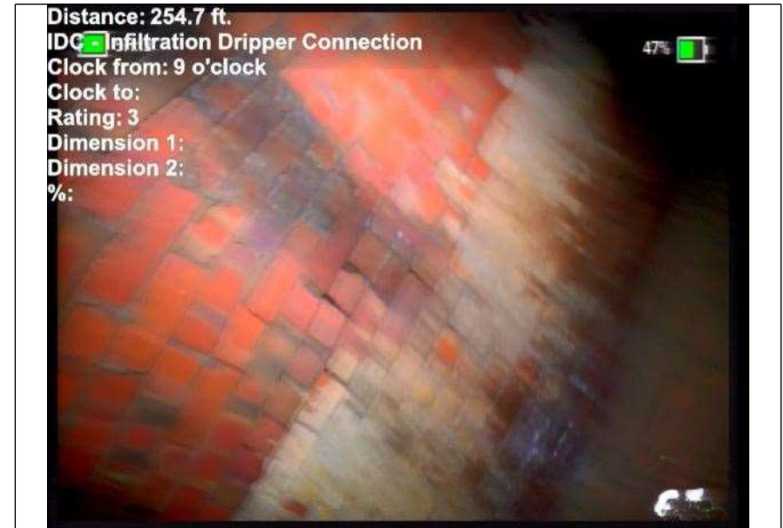
At: 254. IDC - Infiltration Dripper Connection 6999969482 42 ft. 9/.
