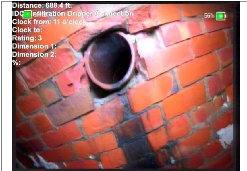
At: 688. IDC - Infiltration Drinker Connection 4000244140 63 ft. 11/.
