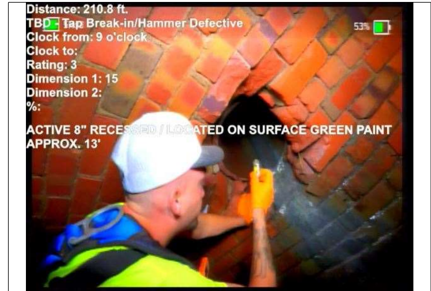
At: 210. TBD - Tap Break-in/Hammer Defective 8000030517 58 ft. 9/.
