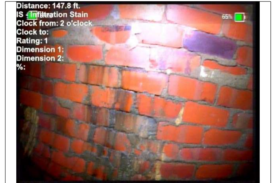
At: 147. IS - Infiltration Stain 8000030517 58 ft. 2/.
