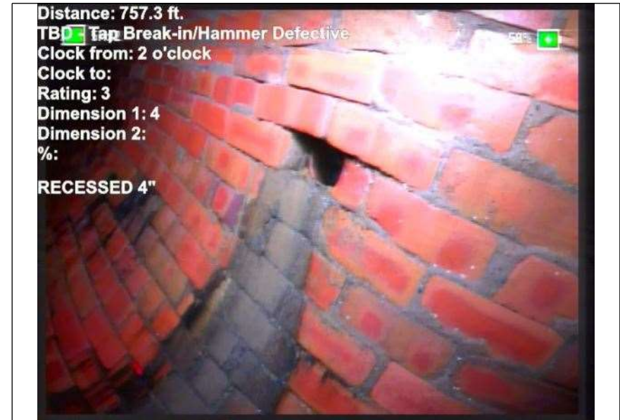
At: 757. TBD - Tap Break-in/Hammer Defective 2999877929 69 ft. 2/.
