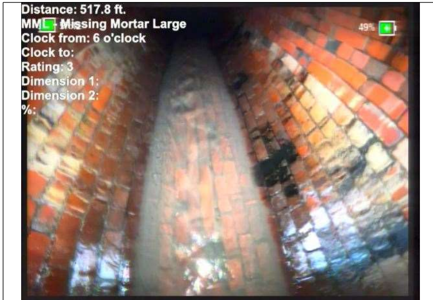
At: 517. MML - Missing Mortar Large 7999877929 69 ft. 6/.
