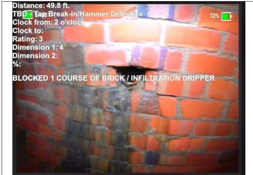
At: 49. 7999992370 TBD - Tap Break-in/Hammer Defective 605 ft. 2/. Joint: No BLOCKED 1 COURSE OF BRICK / INFILTRATION DRIPPER
