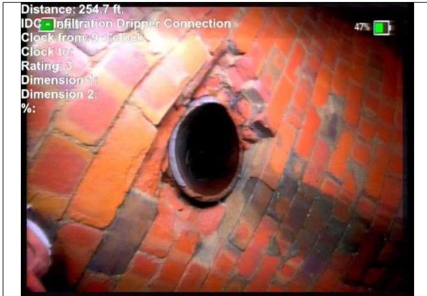
At: 254. IDC - Infiltration Dripper Connection 6999969482 42 ft. 9/.
