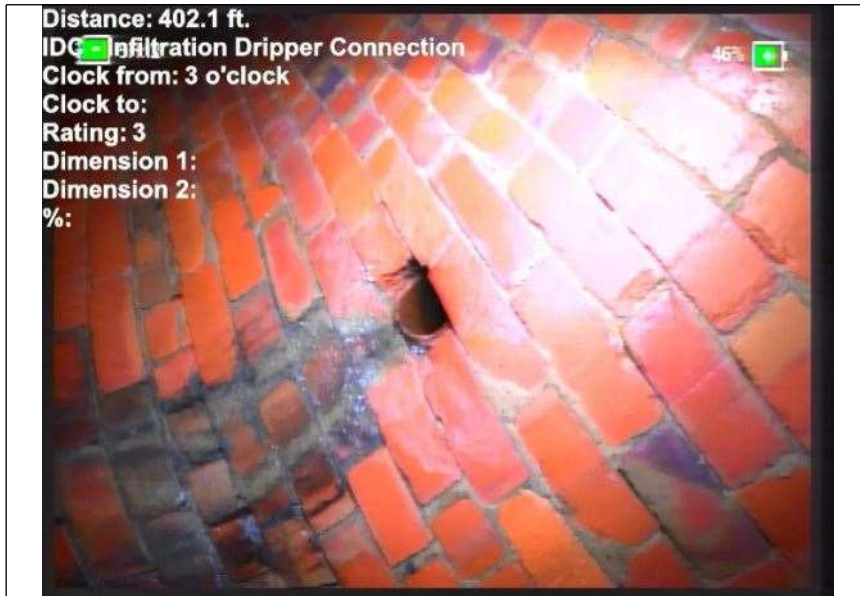
At: 402. IDC - Infiltration Drinker Connection 1000061035 16 ft. 3/.
