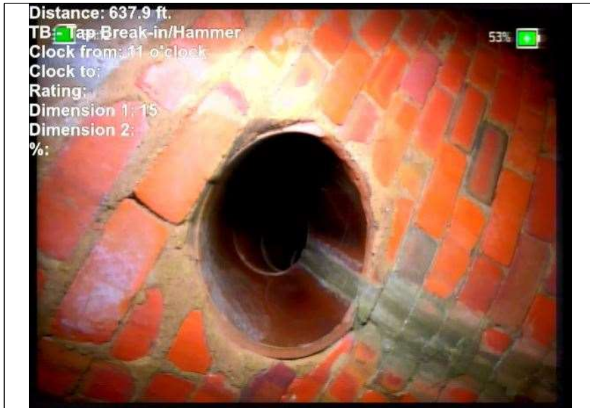
At: 637.9 ft. TB - Tap Break-in/Hammer 9000244140 63 ft. 11/.
