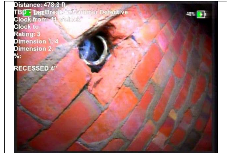
At: 478. TBD - Tap Break-in/Hammer Defective 2999877929 69 ft. 11/.
