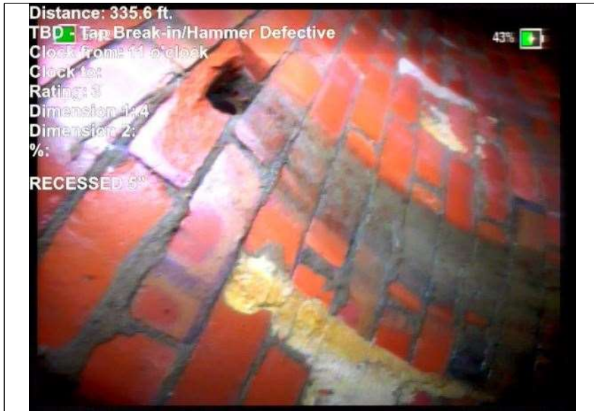
At: 335. TBD - Tap Break-in/Hammer Defective 6000061035 16 ft. 11/.
