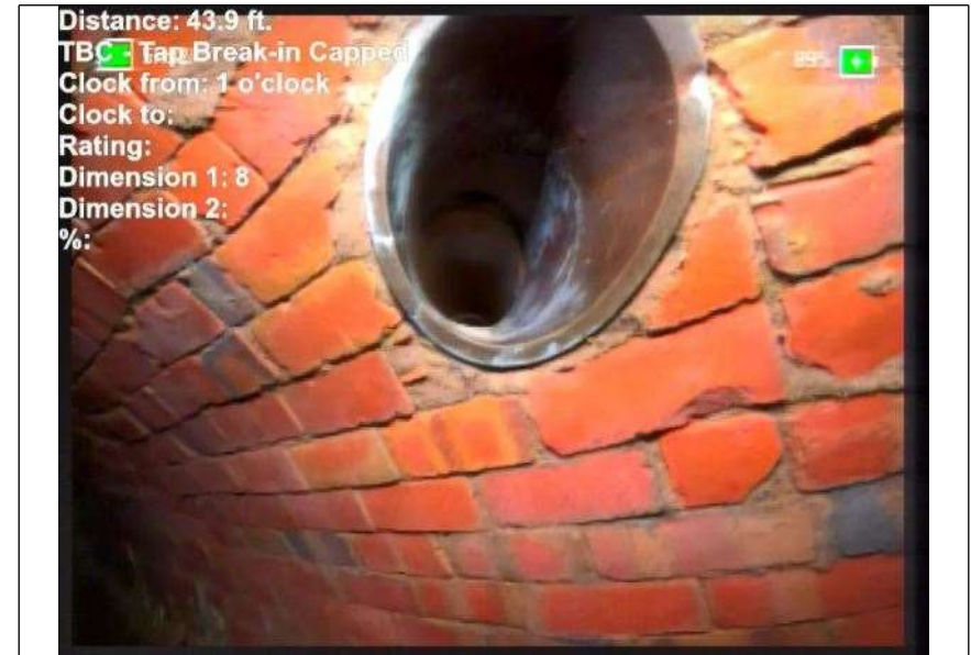
At: 43. TBC - Tap Break-in Capped 9000015258 789 ft. 1/. Joint: No
