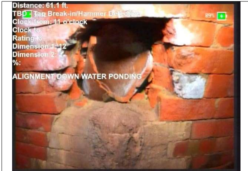
At: 61. TBD - Tap Break-in/Hammer Defective 0999984741 211 ft. 11/. Joint: No ALIGNMENT DOWN WATER PONDING
