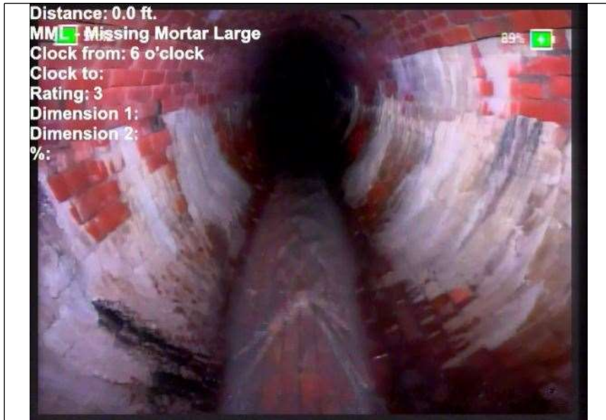
At: 0 ft. 6/. MML - Missing Mortar Large Joint: No
