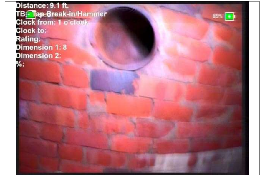
At: 9. TB - Tap Break-in/Hammer 1000003814 6973 ft. 1/. Joint: No
