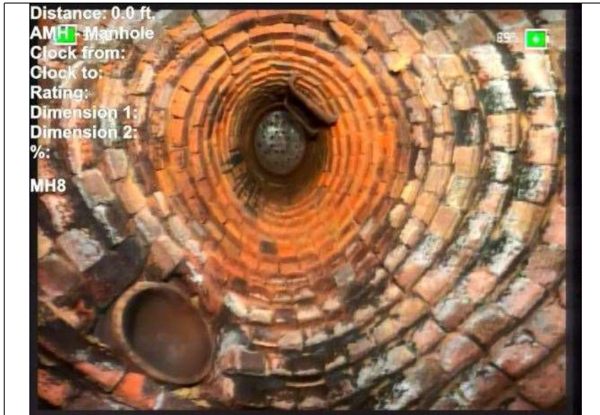
At: 0 ft. AMH - Manhole Joint: No MH8
