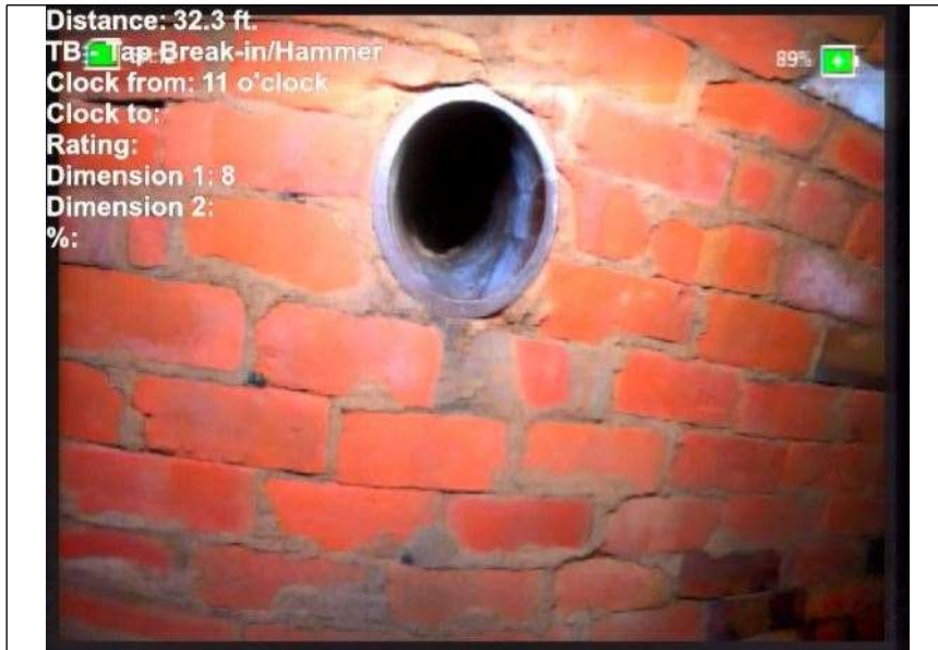
At: 32. TB - Tap Break-in/Hammer 2999992370 605 ft. 11/. Joint: No
