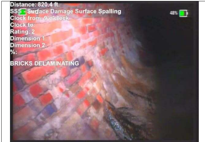
At: 820. 820.4 ft. SSS - Surface Damage Surface Spalling 4000244140 63 ft. 9/.
