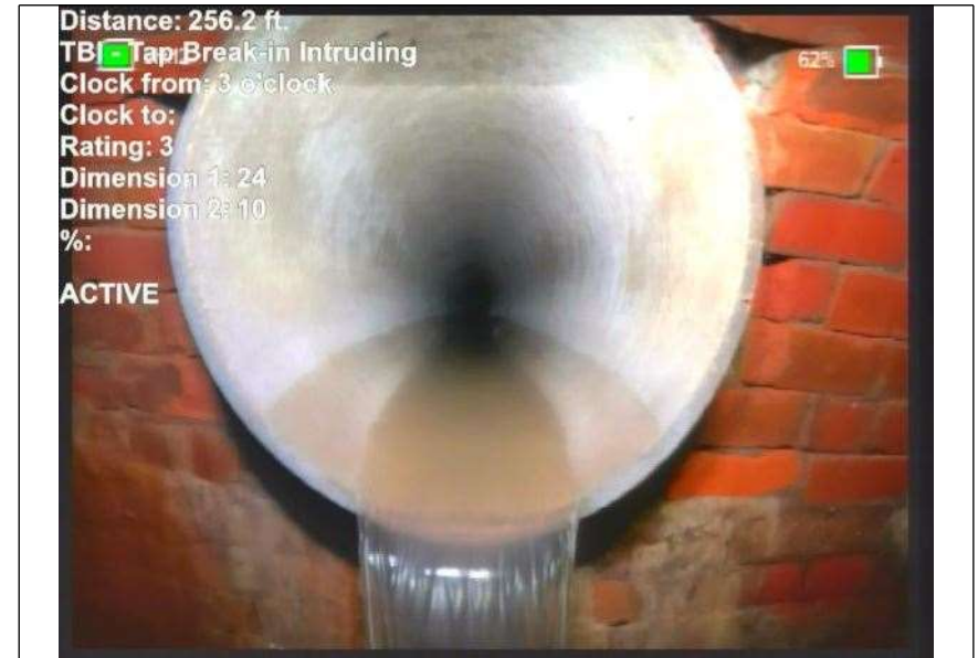
At: 256. TBI - Tap Break-in Intruding 2000122070 31 ft. 3/.
