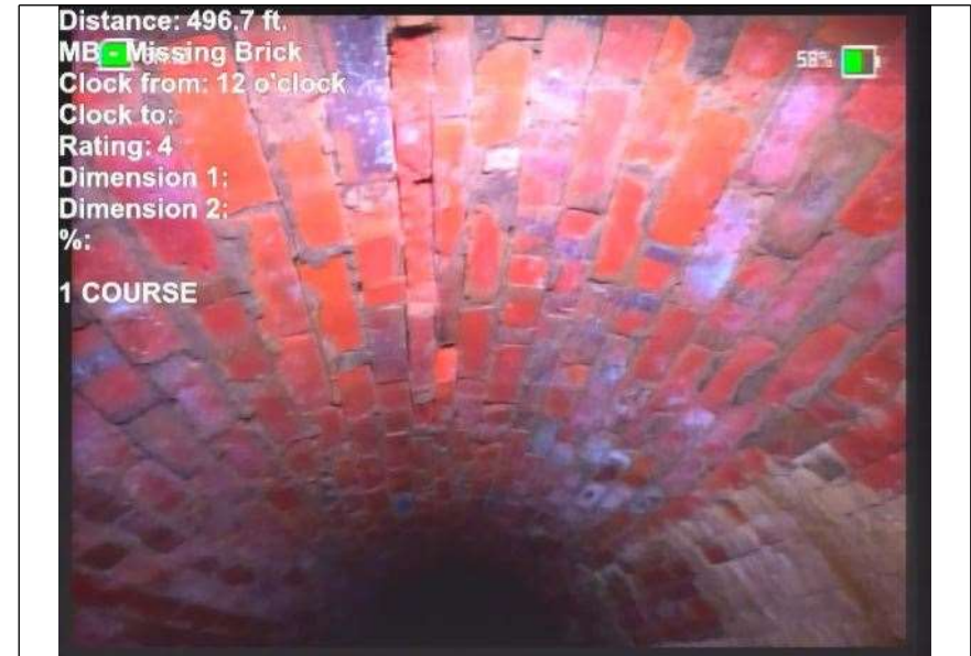
At: 496. MB - Missing Brick 7000122070 31 ft. 12/.
