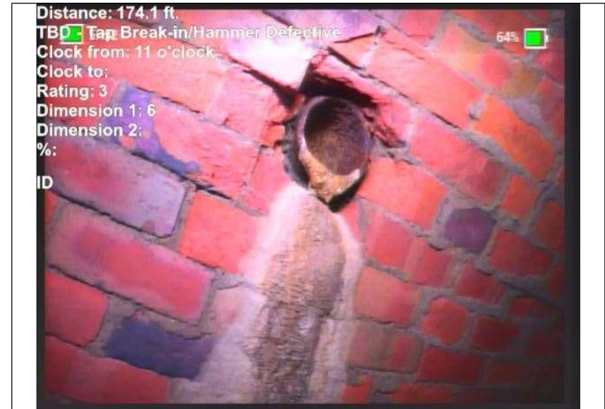
At: 174. TBD - Tap Break-in/Hammer Defective 1000061035 16 ft. 11/.
