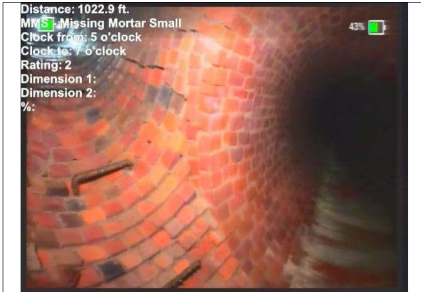
At: 1022. MMS - Missing Mortar Small 9000244140 6 ft. 5/7
