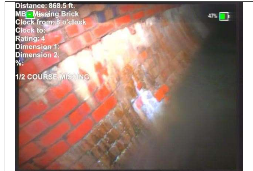
At: 868.5 ft. 8/. MB - Missing Brick
