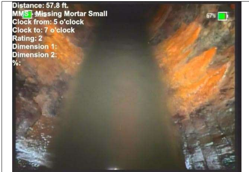
At: 57. MMS - Missing Mortar Small 7999992370 605 ft. 5/7
