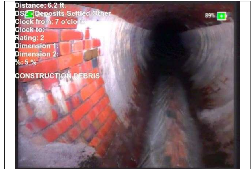
At: 6. 199998092 6514 ft. 7/. DSZ - Deposits Settled Other Joint: No 5 % CONSTRUCTION DEBRIS
