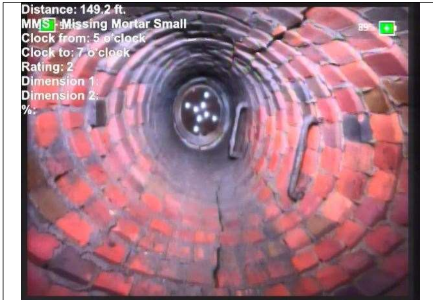
At: 149. MMS - Missing Mortar Small 1999969482 42 ft. 5/7
