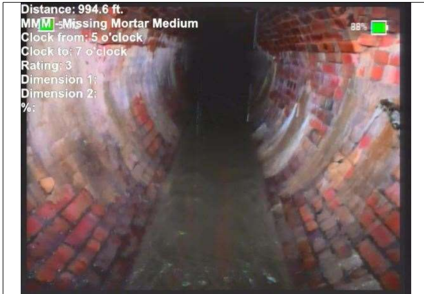
At: 994. 5999755859 MMM - Missing Mortar Medium 38 ft. 5/7
