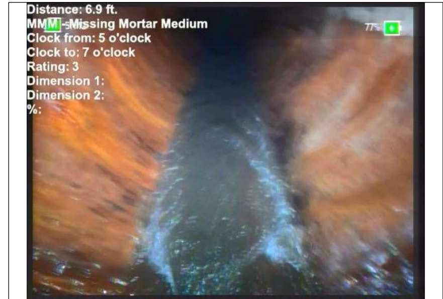
At: 6. MMM - Missing Mortar Medium 9000000953 6743 ft. 5/7 Joint: No
