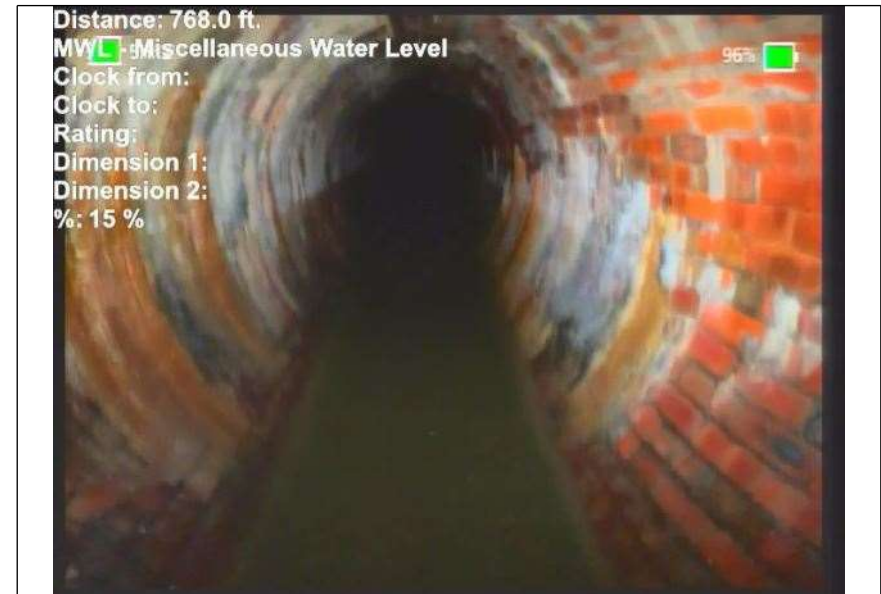
At: 768 ft. MWLS - Miscellaneous Water Level Sag Joint: No 15 %
