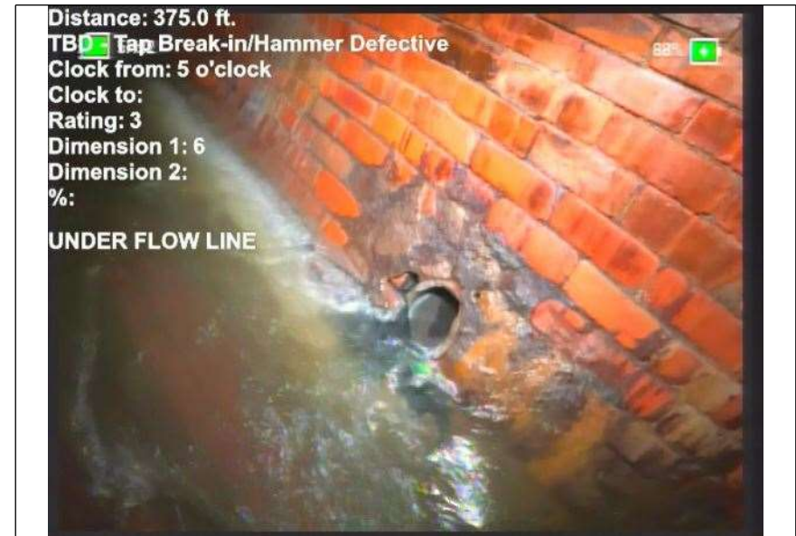
At: 375 ft. 5/. TBD - Tap Break-in/Hammer Defective Joint: No UNDER FLOW LINE
