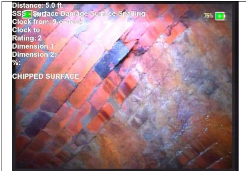
At: 5 ft. 9/ SSS - Surface Damage Surface Spalling Joint: No CHIPPED SURFACE
