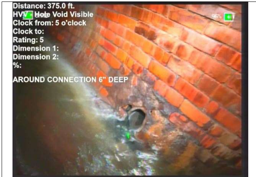
At: 375 ft. 5/. HVV - Hole Void Visible Joint: No AROUND CONNECTION 6" DEEP
