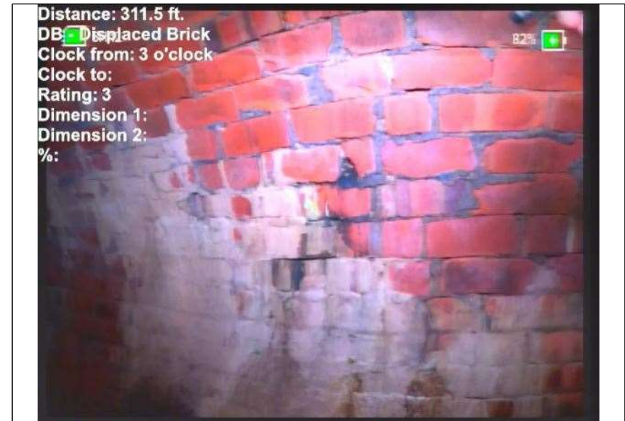
At: 311.5 ft. 3/. DB - Displaced Brick Joint: No
