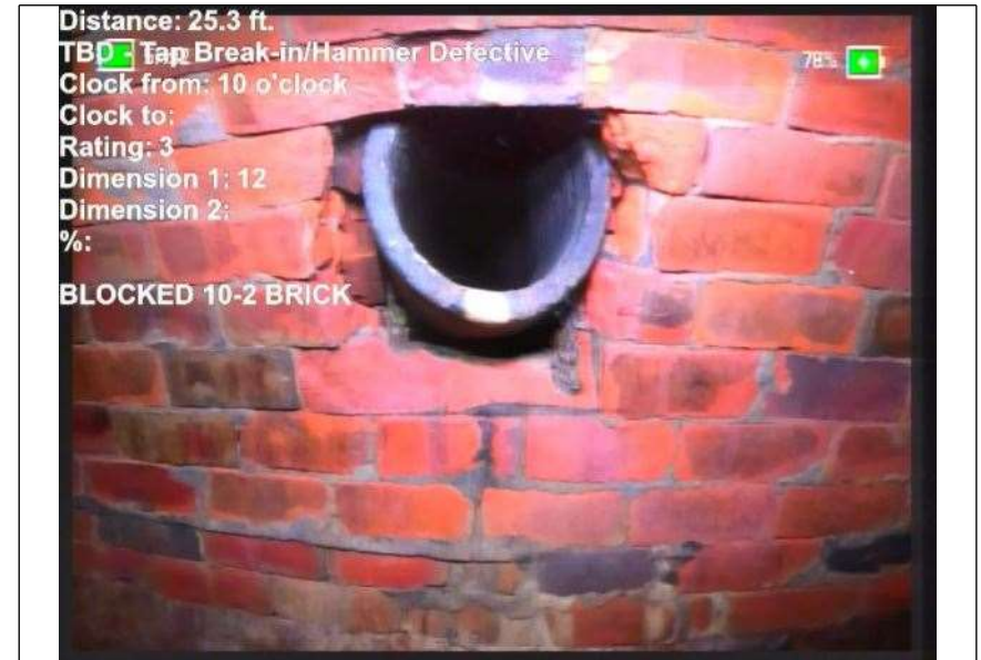
At: 25. TBD - Tap Break-in/Hammer Defective 2999992370 605 ft. 10/.
