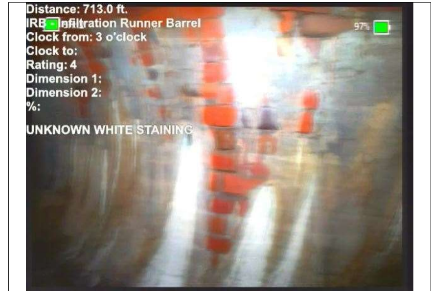
At: 713 ft. 3/. IRB - Infiltration Runner Barrel Joint: No UNKNOWN WHITE STAINING
