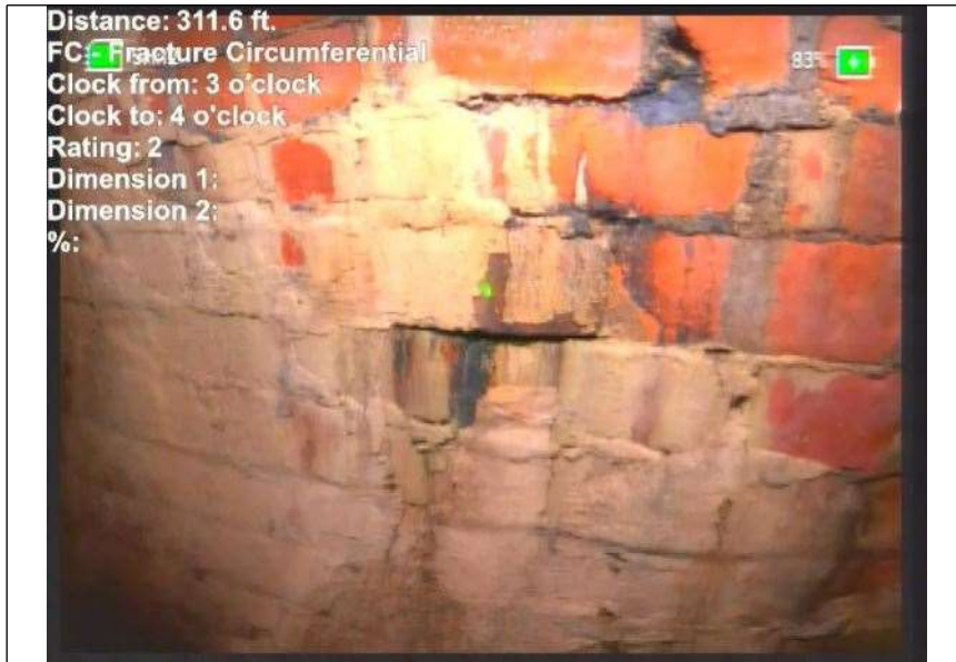
At: 311. FC - Fracture Circumferential 6000061035 16 ft. 3/4 Joint: No
