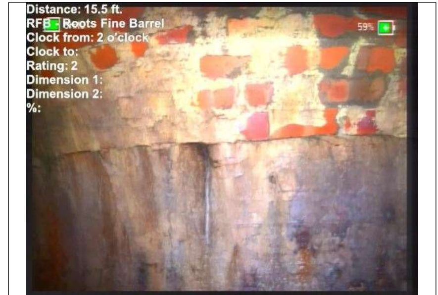
At: 15.5 ft. 2/. RFB - Roots Fine Barrel Joint: No
