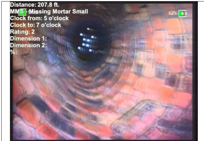
At: 207.7 ft. 5/7 MMS - Missing Mortar Small
