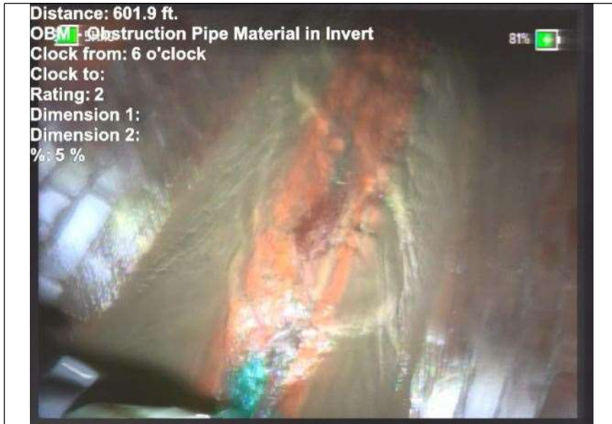
At: 601.9 ft. OBM - Obstruction Pipe Material in Invert 9000244140 63 ft. 6/. Joint: Yes 5 %
