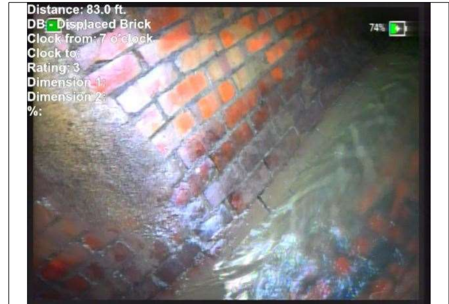
At: 83 ft. 7/. DB - Displaced Brick
