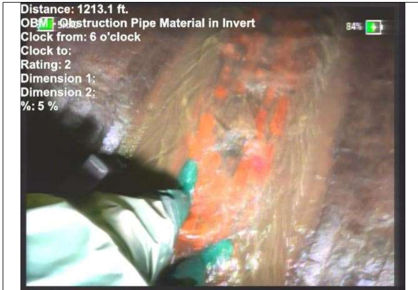
At: 1213. OBM - Obstruction Pipe Material in Invert 0999755859 4 ft. 6/.
