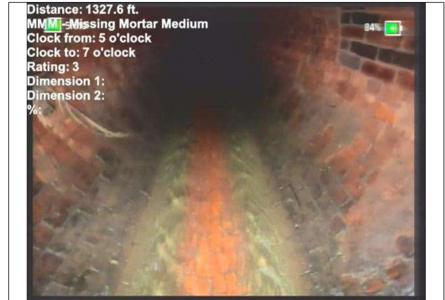
At: 1327. MMM - Missing Mortar Medium 5999755859 4 ft. 5/7
