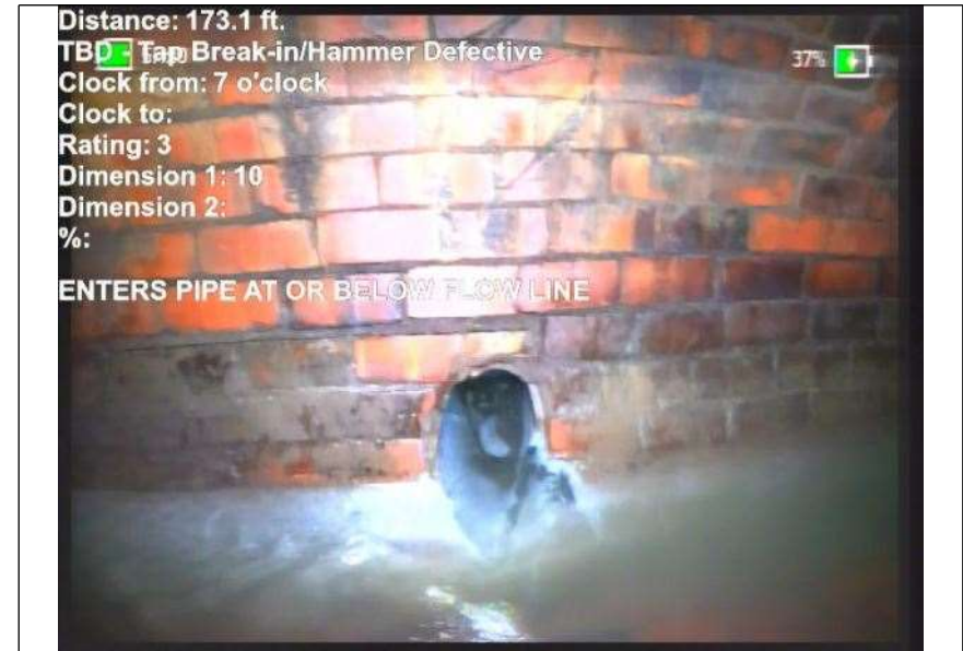
At: 173. TBD - Tap Break-in/Hammer Defective 1000061035 16 ft. 7/.
