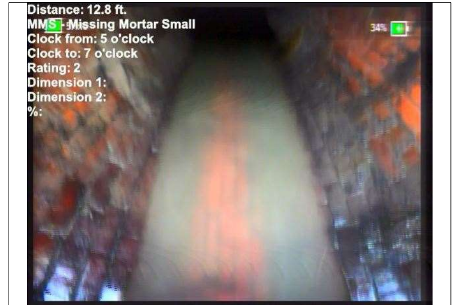
At: 12. MMS - Missing Mortar Small 8000001907 349 ft. 5/7 Joint: No
