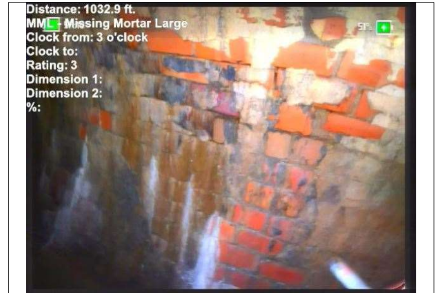
At: 1032. MML - Missing Mortar Large 9000244140 6 ft. 3/. Joint: No
