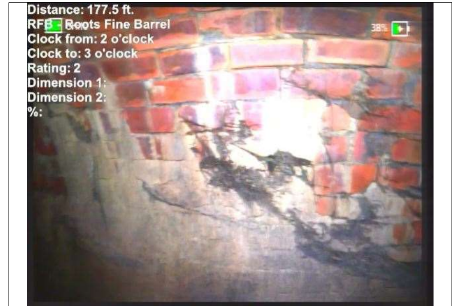
At: 177.5 ft. 2/3 RFB - Roots Fine Barrel Joint: No
