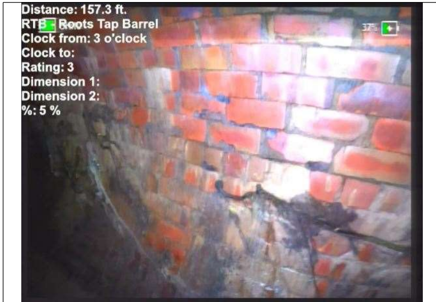
At: 157. RTB - Roots Tap Barrel 3000030517 58 ft. 3/. Joint: No 5 %
