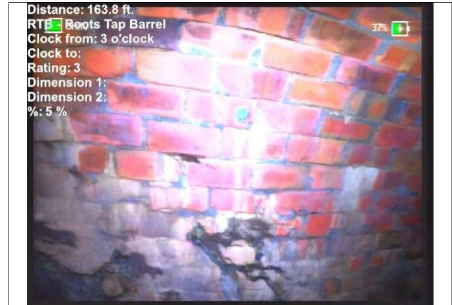
At: 163. RTB - Roots Tap Barrel 8000030517 58 ft. 3/. Joint: No 5 %
