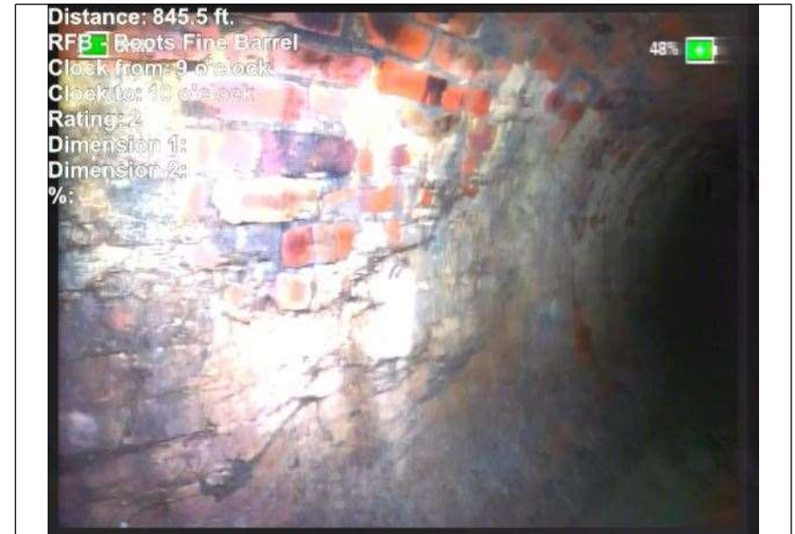
At: 845.5 ft. RFB - Roots Fine Barrel 9/10 Joint: No
