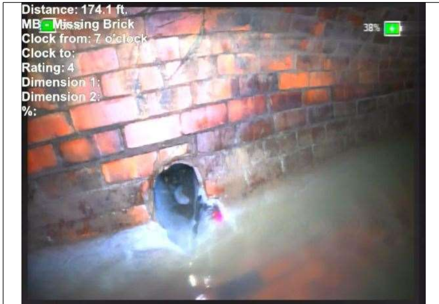
At: 174. MB - Missing Brick 1000061035 16 ft. 7/.
