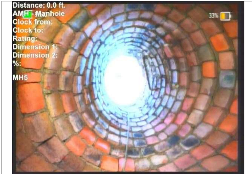
At: 0 ft. AMH - Manhole Joint: No MH4
