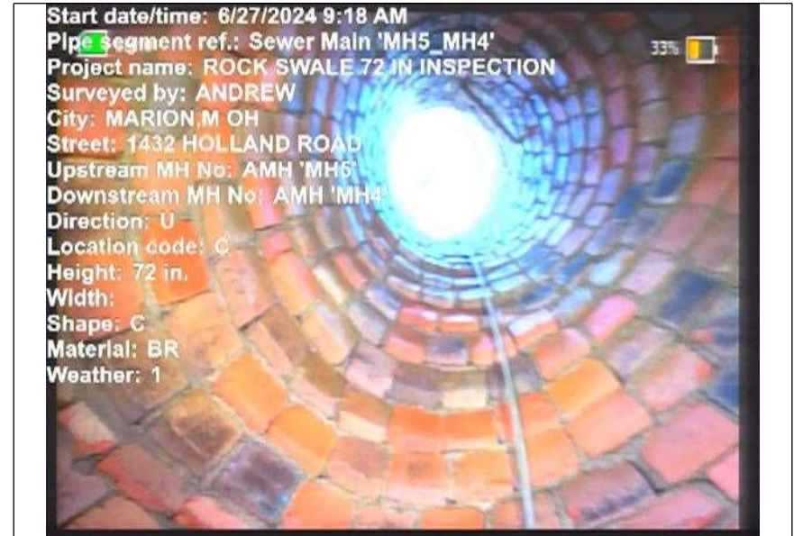
At: 0 ft. AMH - Manhole Joint: No MH4
