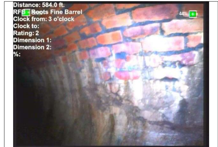
At: 584 ft. 3/. RFB - Roots Fine Barrel Joint: No
