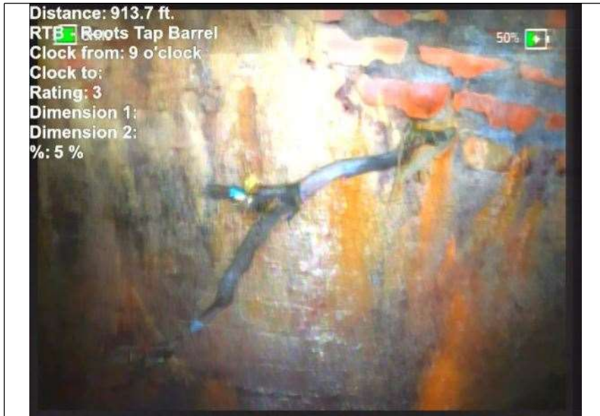
At: 913. RTB - Roots Tap Barrel 7000122070 31 ft. 9/. Joint: No 5 %
