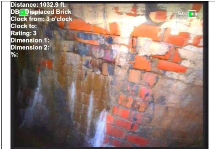
At: 1032. DB - Displaced Brick 9000244140 6 ft. 3/.
