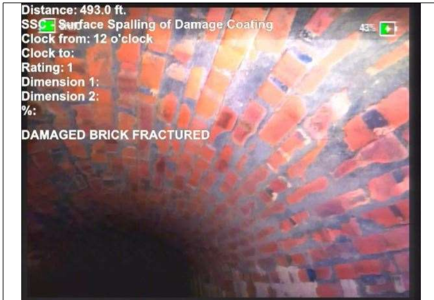
At: 493 ft. 12/. SSC - Surface Spalling of Damage Coating Joint: No DAMAGED BRICK FRACTURED
