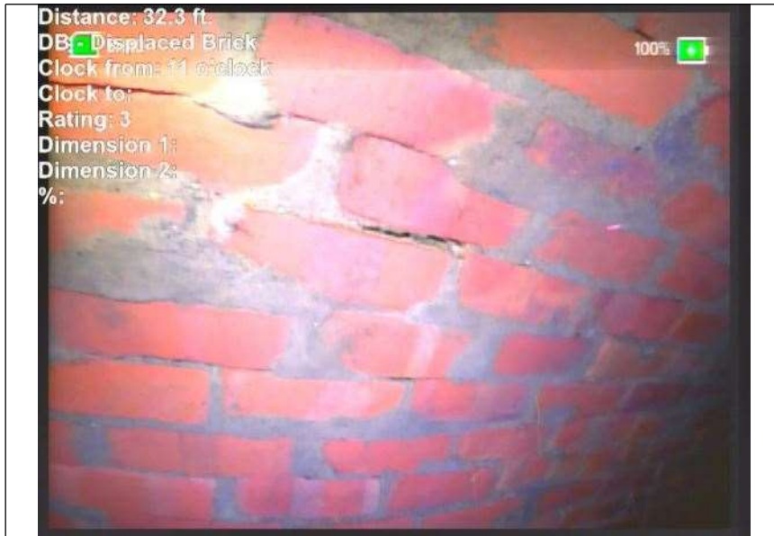
At: 32. DB - Displaced Brick 2999992370 605 ft. 11/.
