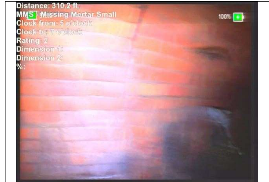
At: 310. MMS - Missing Mortar Small 2000122070 31 ft. 5/7
