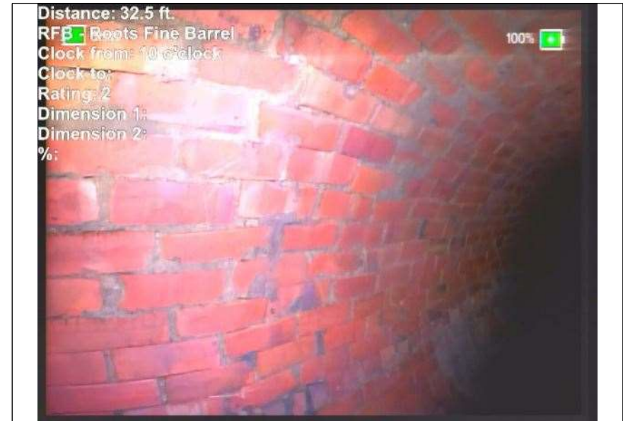
At: 32.5 ft. 10/. RFB - Roots Fine Barrel Joint: No
