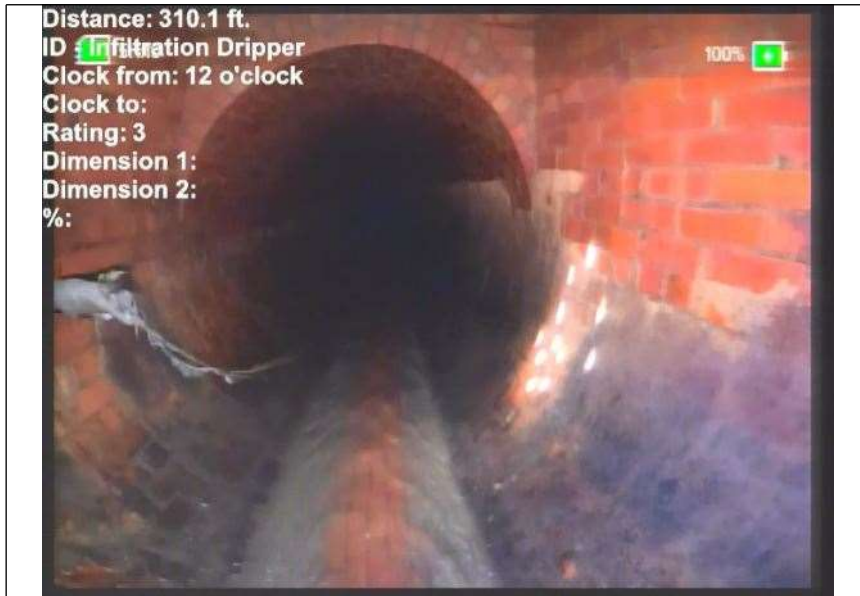
At: 310. ID - Infiltration Dripper 1000061035 16 ft. 12/.
