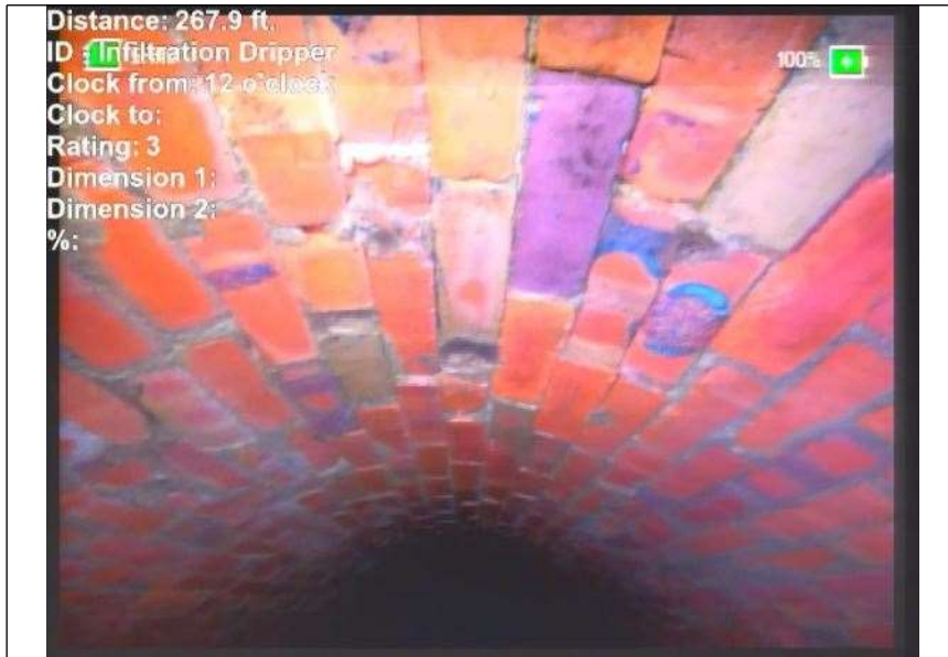
At: 267. ID - Infiltration Dripper 8999938964 84 ft. 12/.
