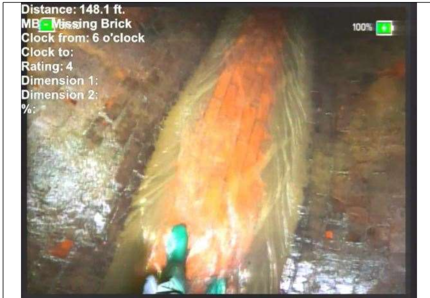
At: 148. MB - Missing Brick 1000061035 16 ft. 6/.
