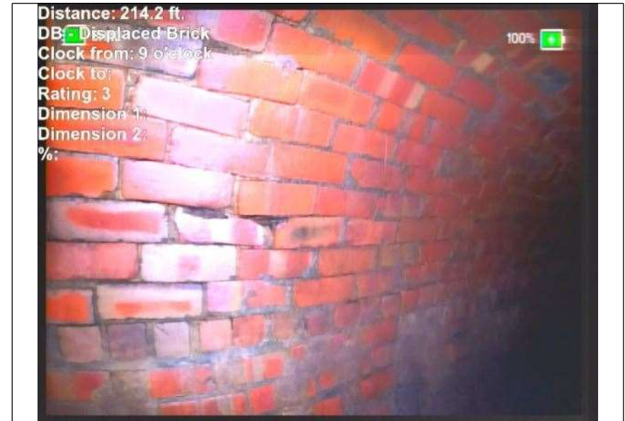
At: 214. DB - Displaced Brick 1999969482 42 ft. 9/.
