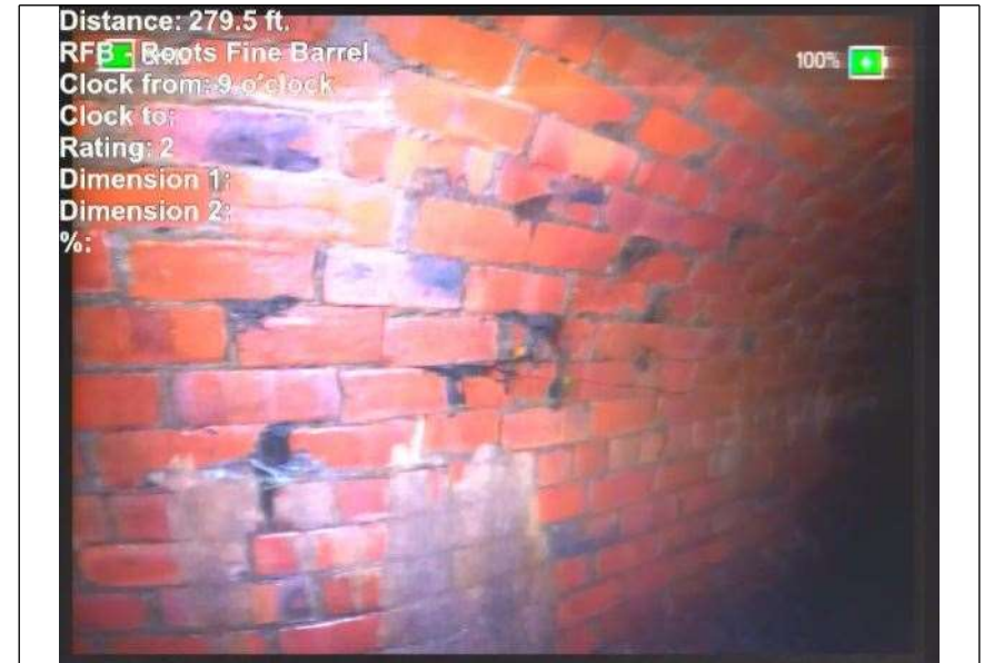
At: 279.5 ft. 9/. RFB - Roots Fine Barrel Joint: No
