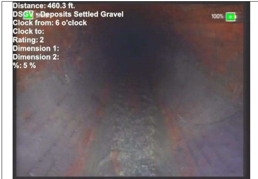
At: 460. DSGV - Deposits Settled Gravel 2999877929 69 ft. 6/. Joint: No 5 %
