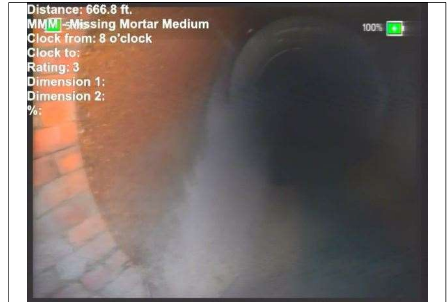
At: 666. MMM - Missing Mortar Medium 7999877929 69 ft. 8/. Joint: No
