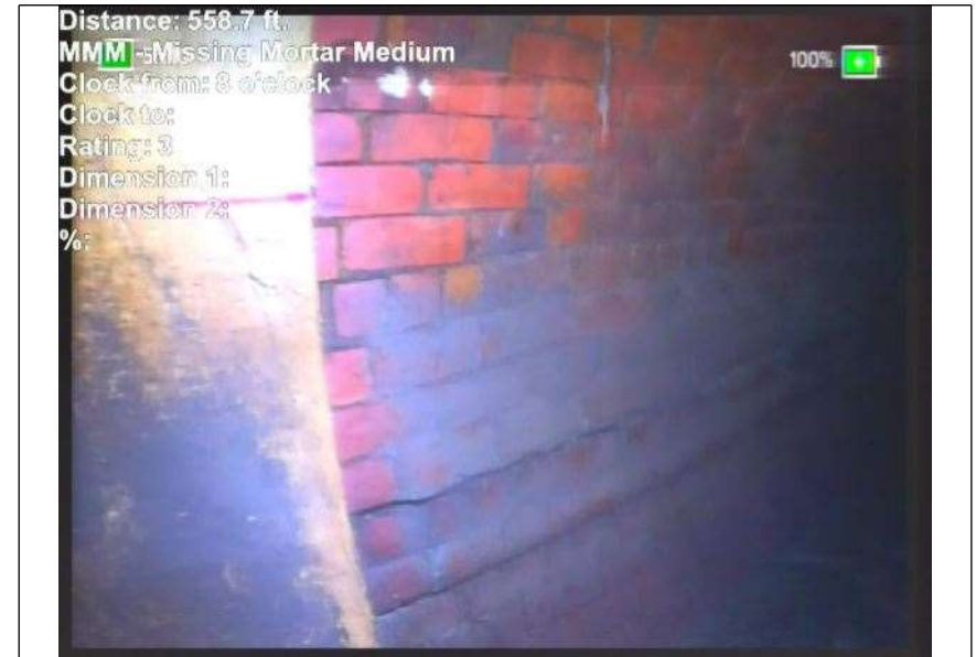
At: 558. 7000122070 MMM - Missing Mortar Medium 31 ft. 8/.
