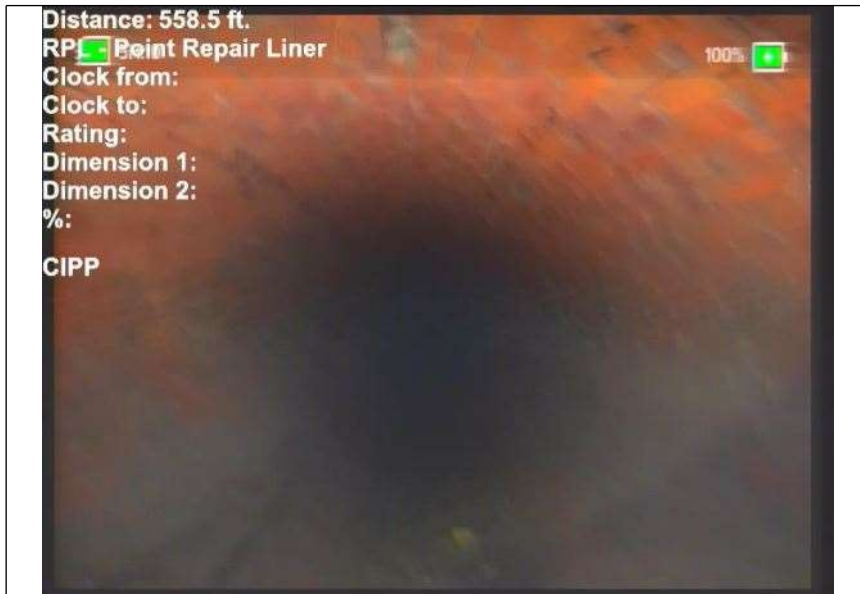
At: 558.5 ft. RPL - Point Repair Liner Joint: No CIPP
