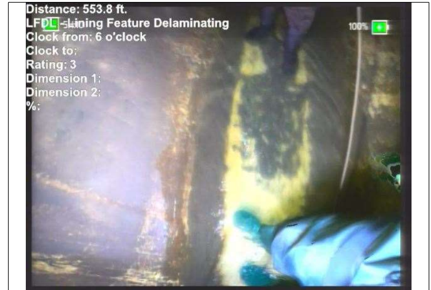
At: 553. LFDL - Lining Feature Delaminating 7999877929 69 ft. 6/.
