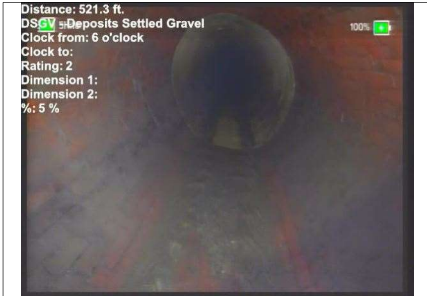
At: 521. DSGV - Deposits Settled Gravel 2999877929 69 ft. 6/. Joint: No 5 %
