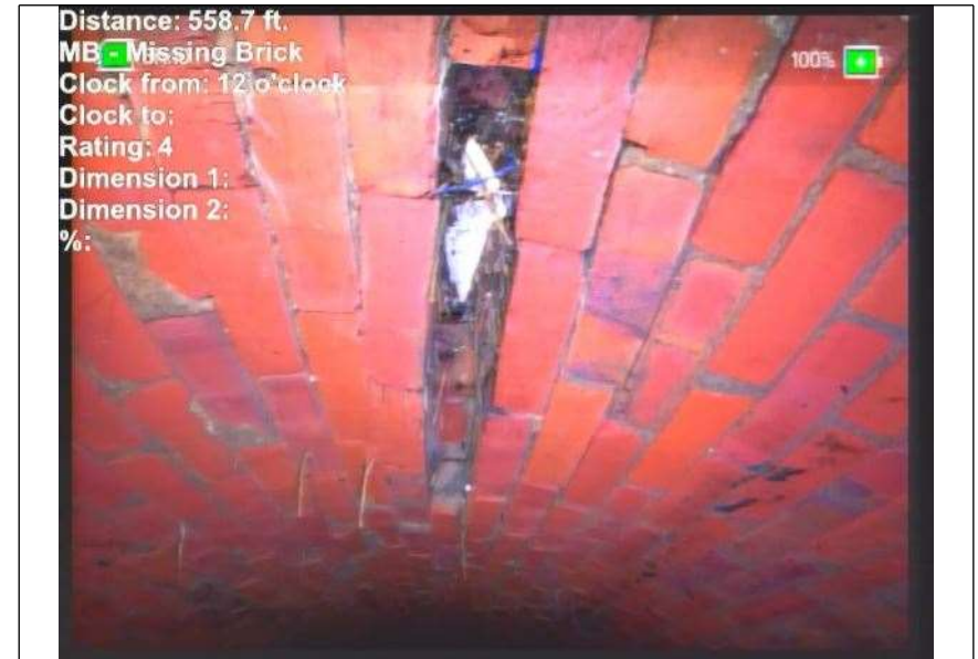
At: 558. MB - Missing Brick 7000122070 31 ft. 12/.
