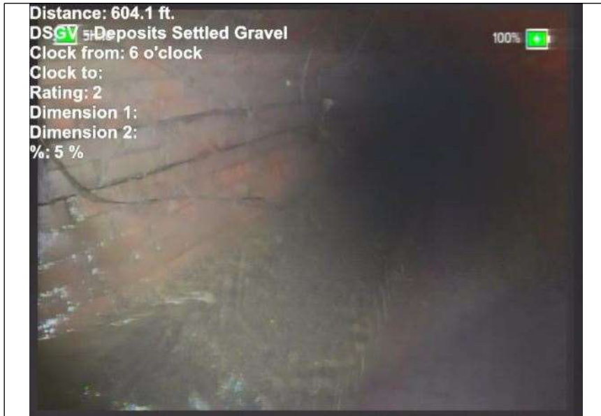
At: 604. DSGV - Deposits Settled Gravel 0999755859 38 ft. 6/. Joint: No 5 %
