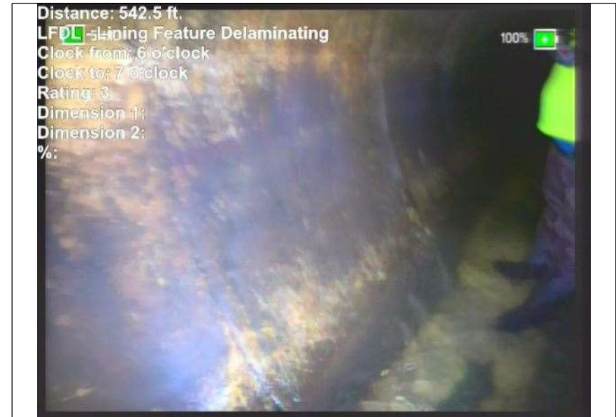
At: 542.5 ft. 6/7 LFDL - Lining Feature Delaminating Joint: No
