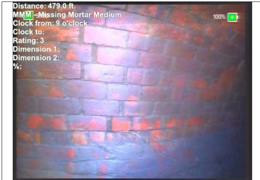
At: 479 ft. 9/. MMM - Missing Mortar Medium
