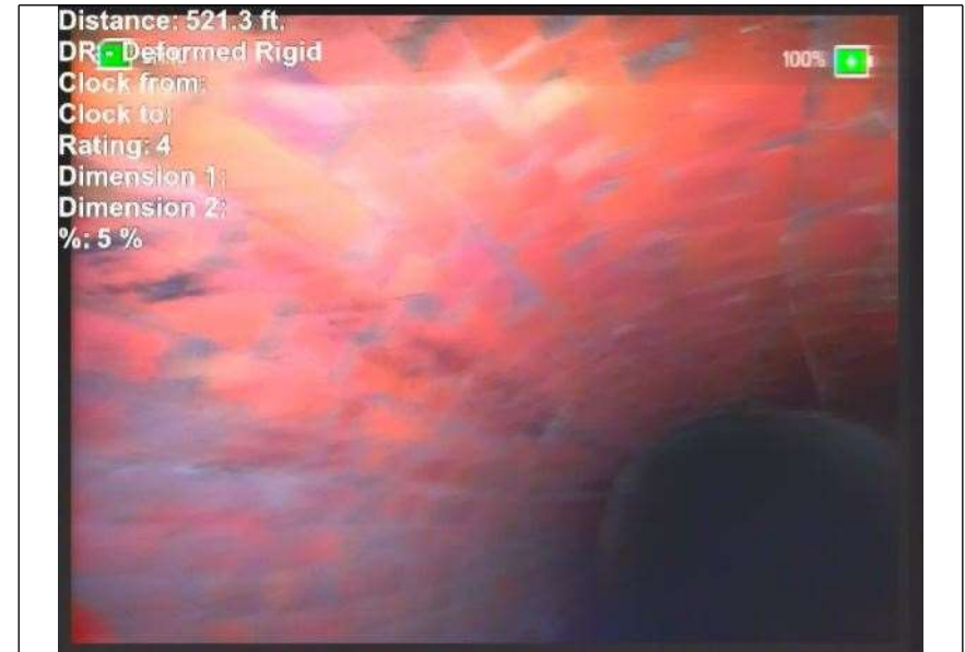
At: 521. DR - Deformed Rigid 2999877929 69 ft. Joint: No 5 %
