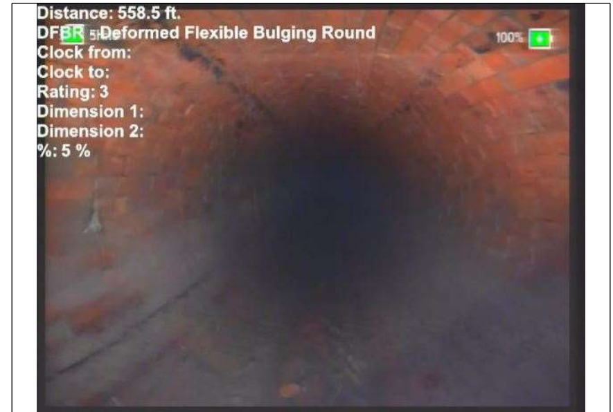
At: 558.5 ft. DFBR - Deformed Flexible Bulging Round Joint: No 5 %
