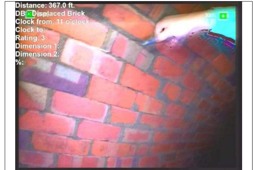
At: 367 ft. 11/. DB - Displaced Brick Joint: No
