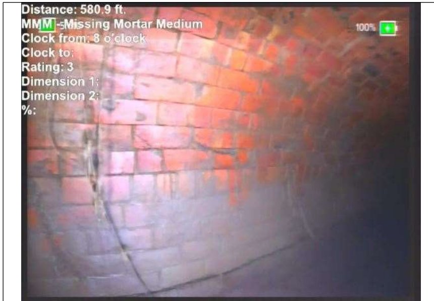
At: 580. MMM - Missing Mortar Medium 9000244140 63 ft. 8/.
