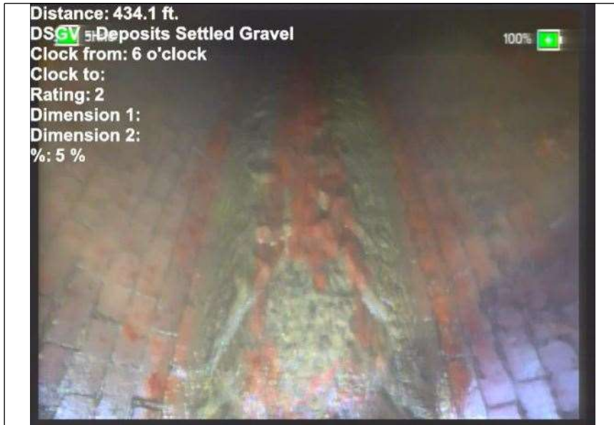
At: 434. DSGV - Deposits Settled Gravel 1000061035 16 ft. 6/. Joint: No 5 %
