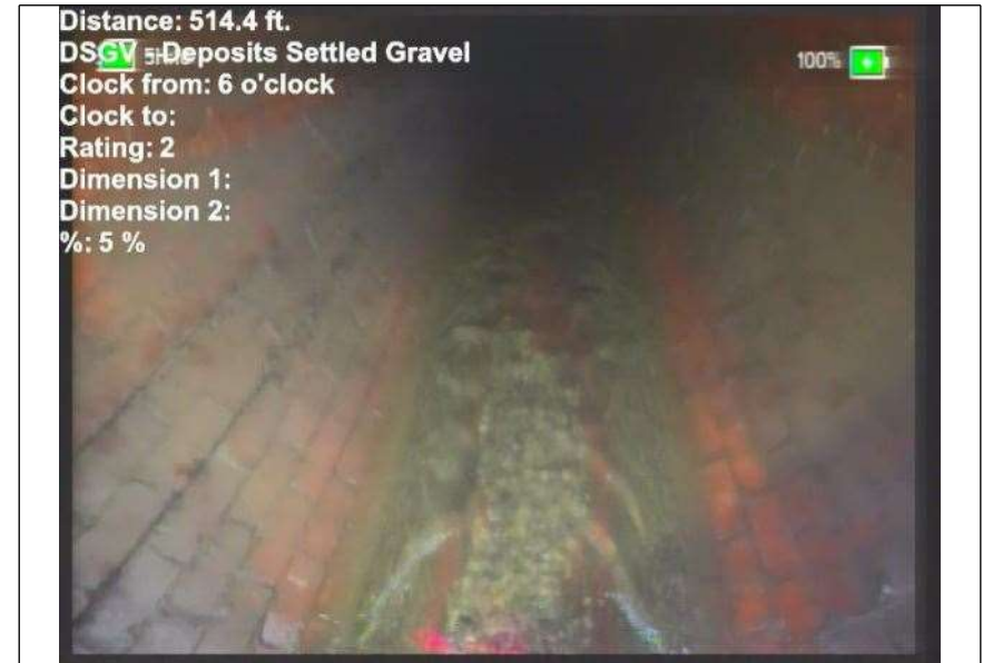
At: 514. DSGV - Deposits Settled Gravel 4000244140 63 ft. 6/. Joint: No 5 %
