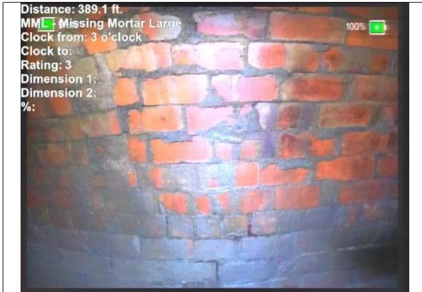
At: 389. MML - Missing Mortar Large 1000061035 16 ft. 3/.
