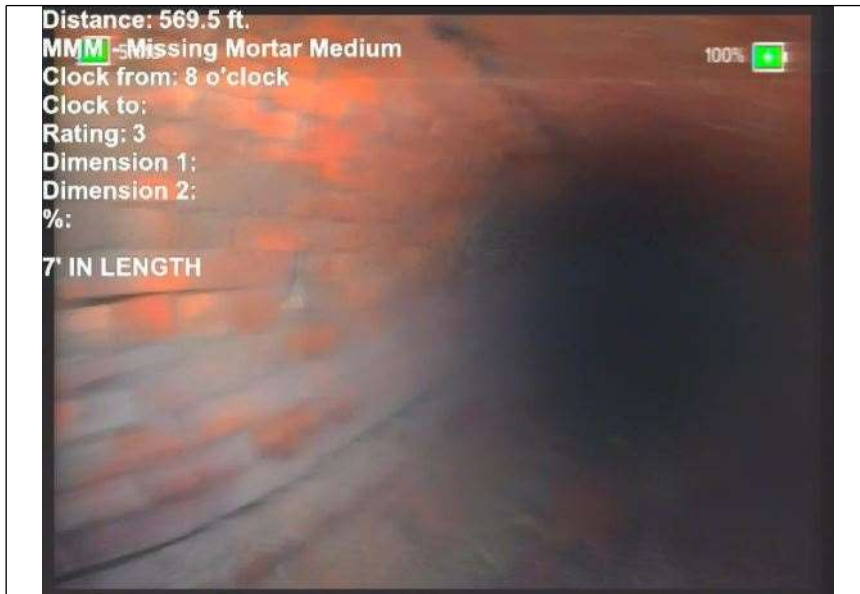
At: 569.5 ft. 8/. 7000122070 MMM - Missing Mortar Medium
