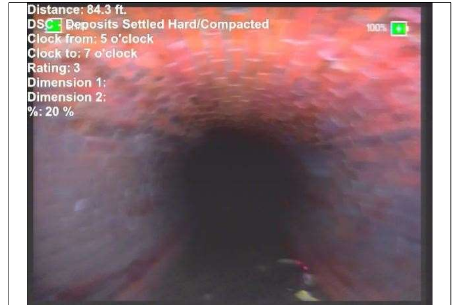
At: 84. DSC - Deposits Settled Hard/Compacted 3000030517 578 ft. 5/7 Joint: No 20 %
