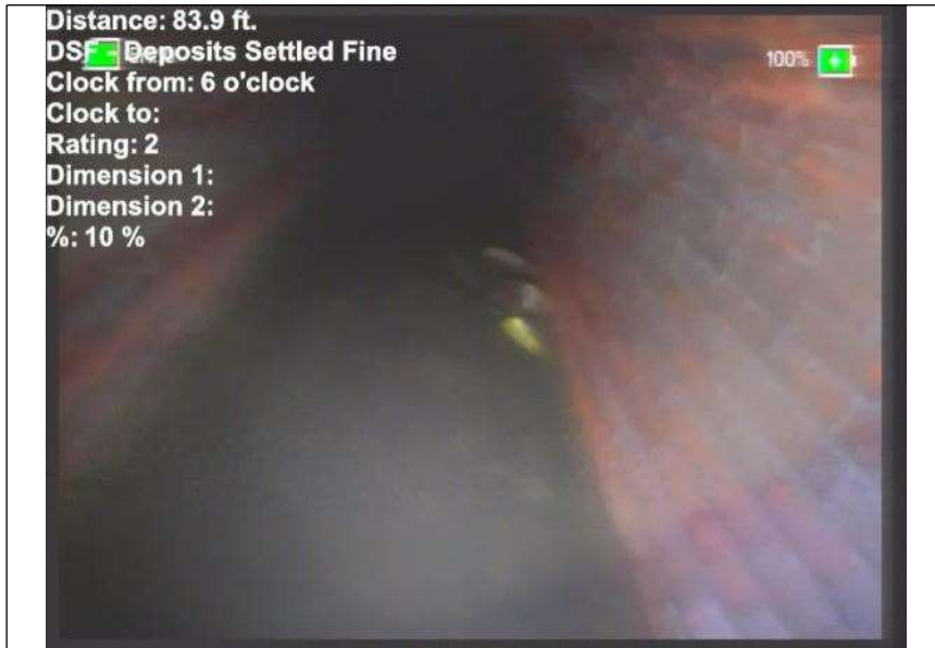
At: 83. DSF - Deposits Settled Fine 9000015258 789 ft. 6/. Joint: No 10 %
