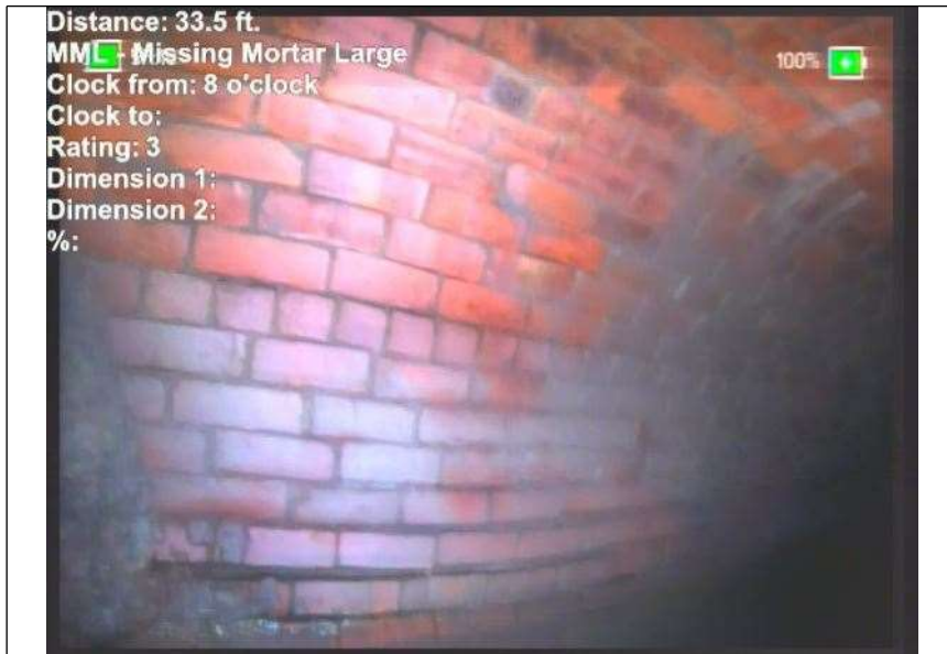
At: 33.5 ft. 8/. MML - Missing Mortar Large
