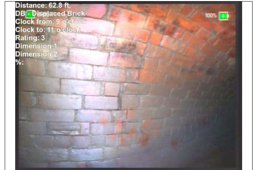
At: 62. 7999992370 DB - Displaced Brick 605 ft. 9/11 Joint: No
