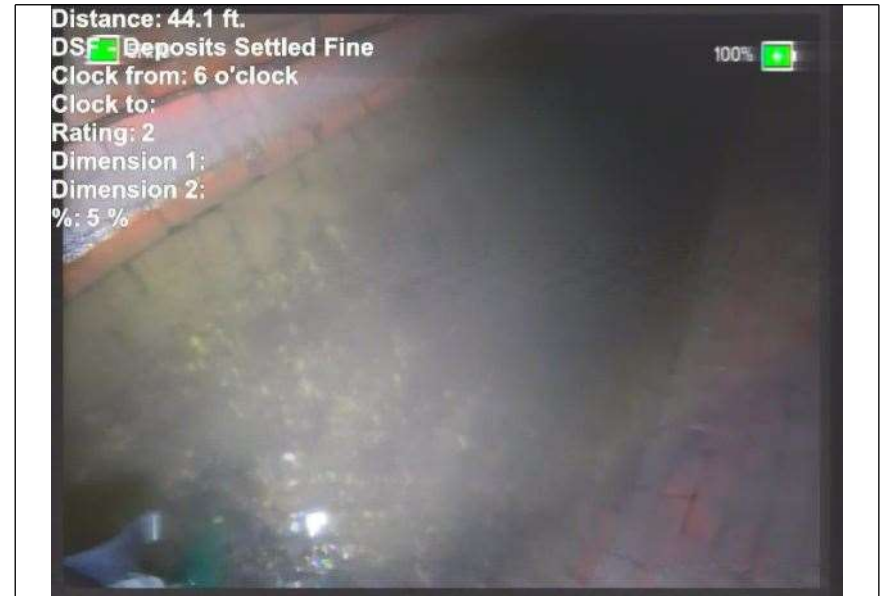
At: 44. DSF - Deposits Settled Fine 0999984741 211 ft. 6/ Joint: No 5 %
