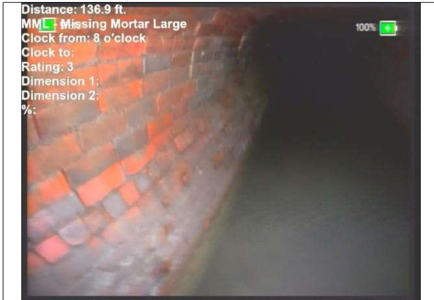
At: 136. MML - Missing Mortar Large 8999938964 84 ft. 8/.
