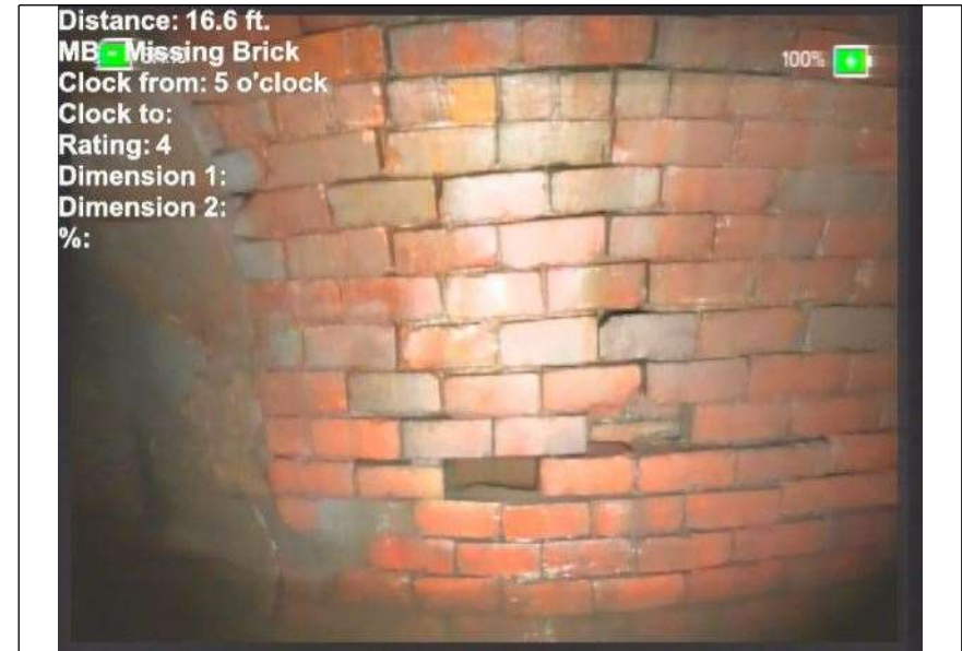
At: 16. MB - Missing Brick 6000003814 697 ft. 5/.
