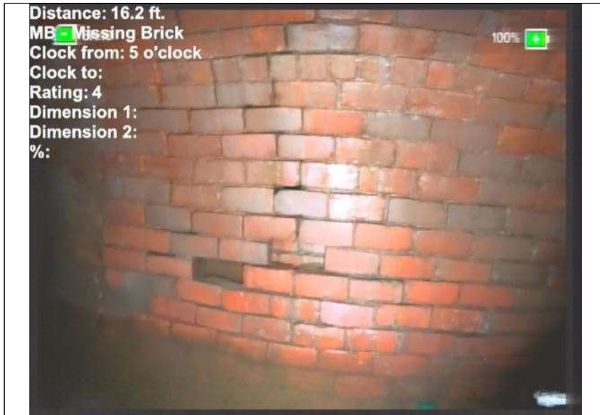
At: 16. MB - Missing Brick 2000007629 395 ft. 5/.
