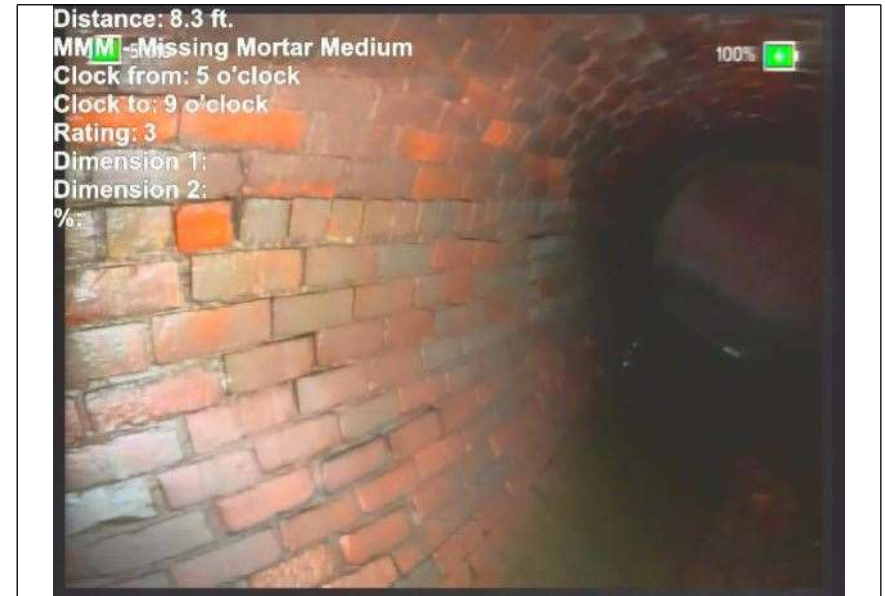
At: 8. MMM - Missing Mortar Medium 3000001907 3486 ft. 5/9 Joint: No
