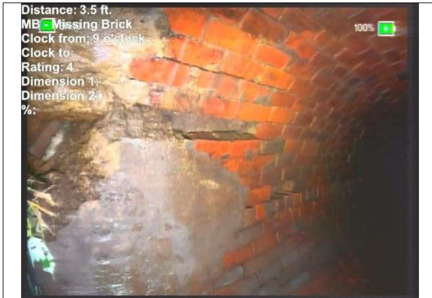
At: 3.5 ft. 9/. MB - Missing Brick
