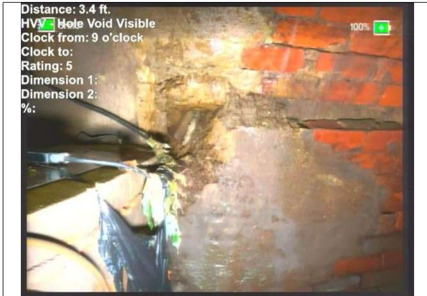
At: 3. HVV - Hole Void Visible 4000000953 6743 ft. 9/.
