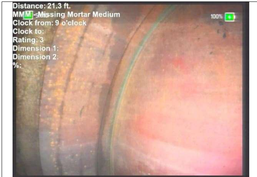
At: 21.2 ft. 5/9 MMM - Missing Mortar Medium
