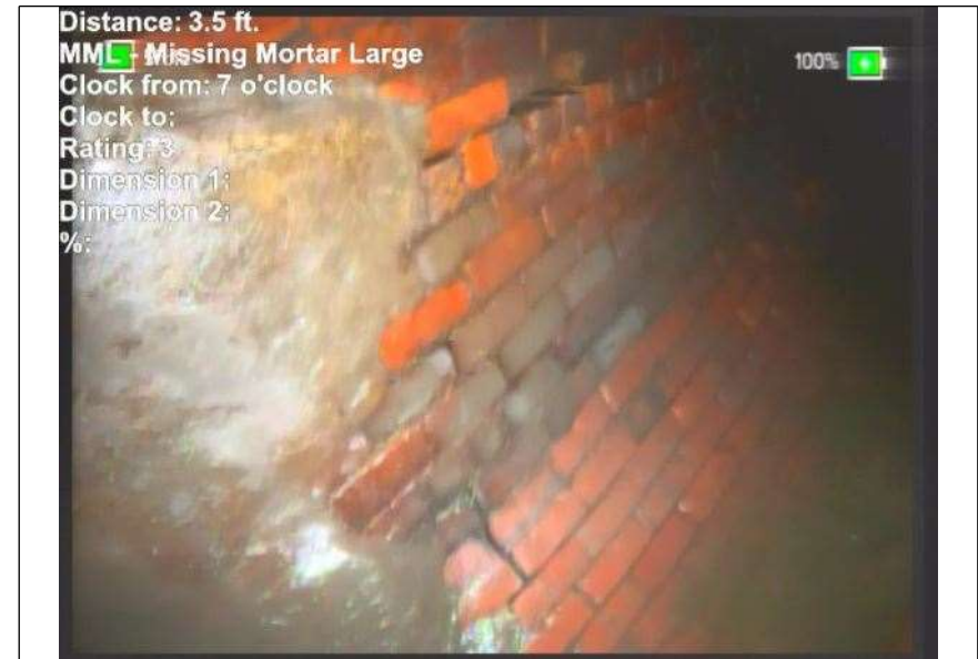
At: 3.5 ft. 7/. MML - Missing Mortar Large
