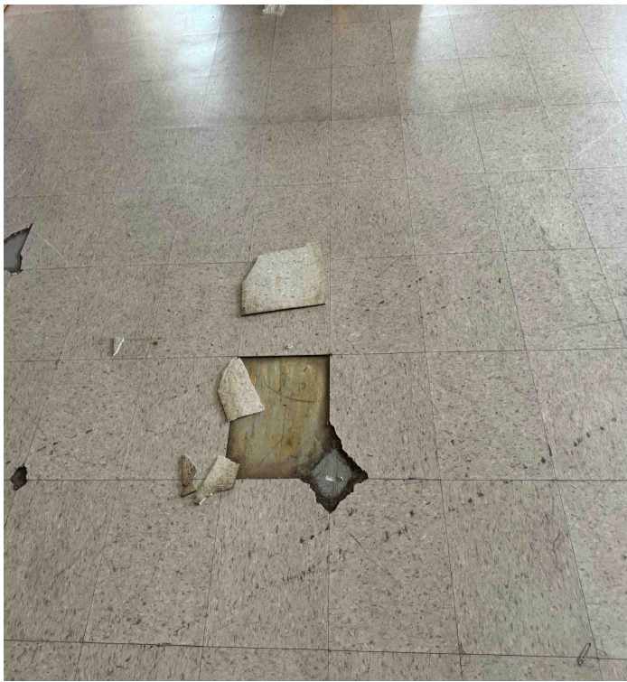
HA #02 (12x12) 2nd Story Floor Tile with Mastic
