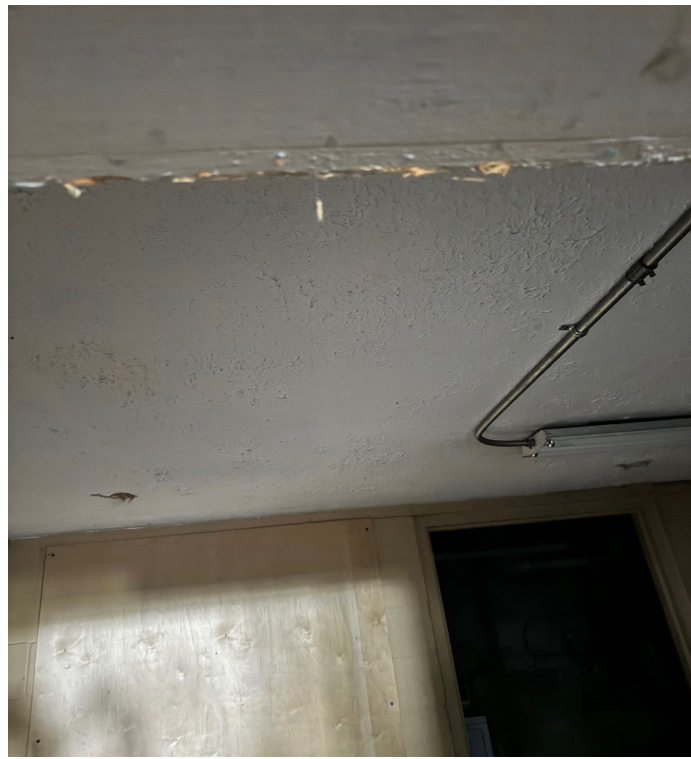
HA #05/#10 2nd Story Restroom & 1st Floor Laundry Room Ceiling Texture
