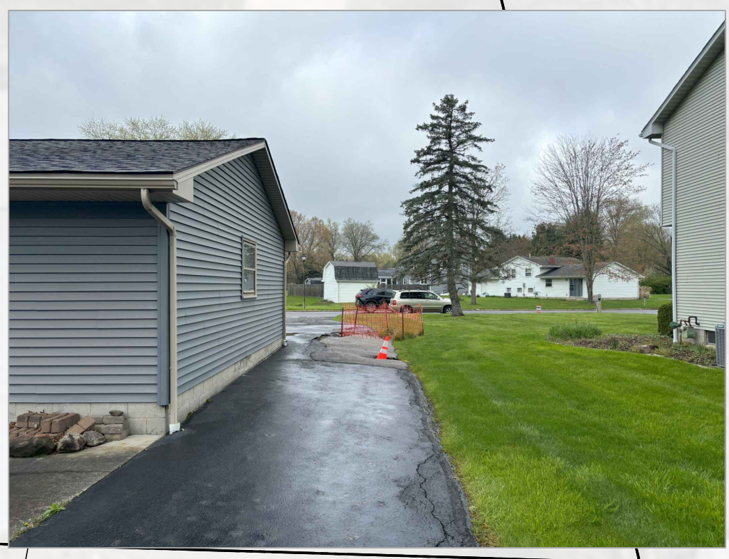
EXISTING FAILING DRIVEWAY - 6817 COLLEEN DR (FACING WEST)
