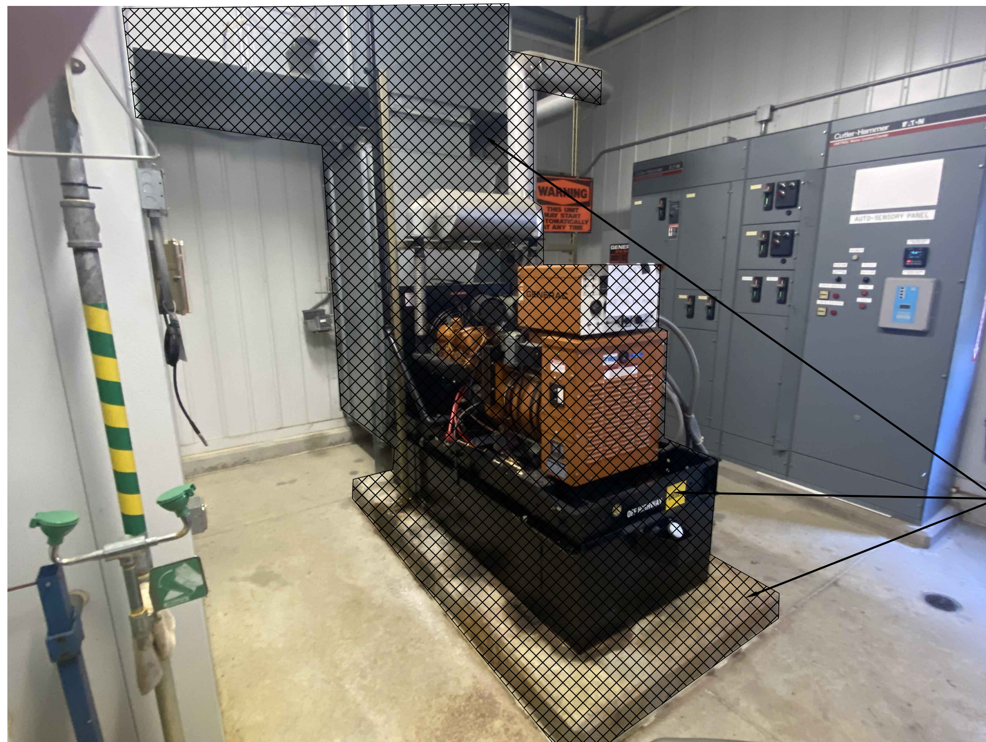
PHOTO 9 - PALMER AVE. TANK EXISTING GENERATOR
