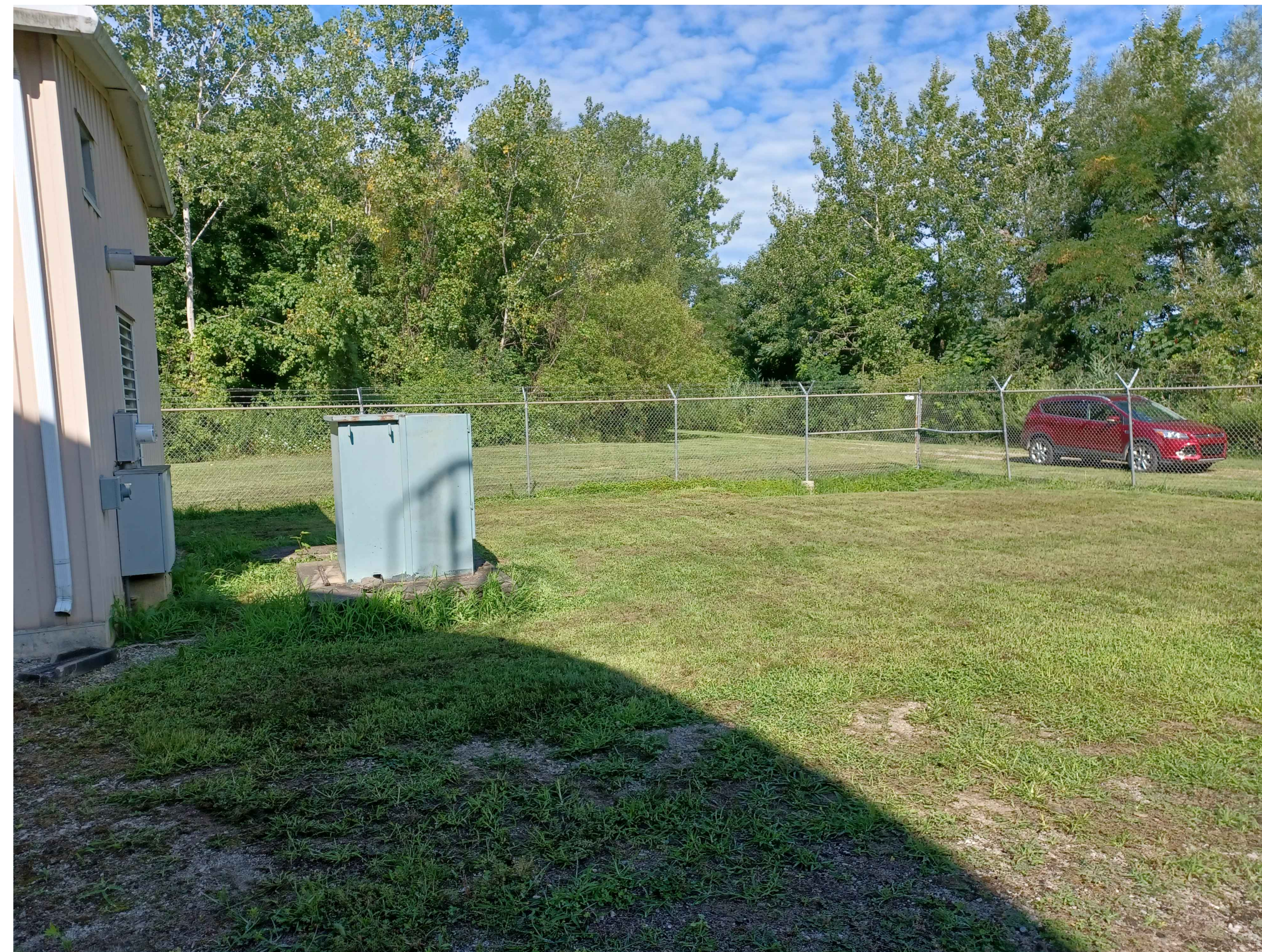
PHOTO 12 - PALMER AVE. TANK PROP. GENERATOR SITE
