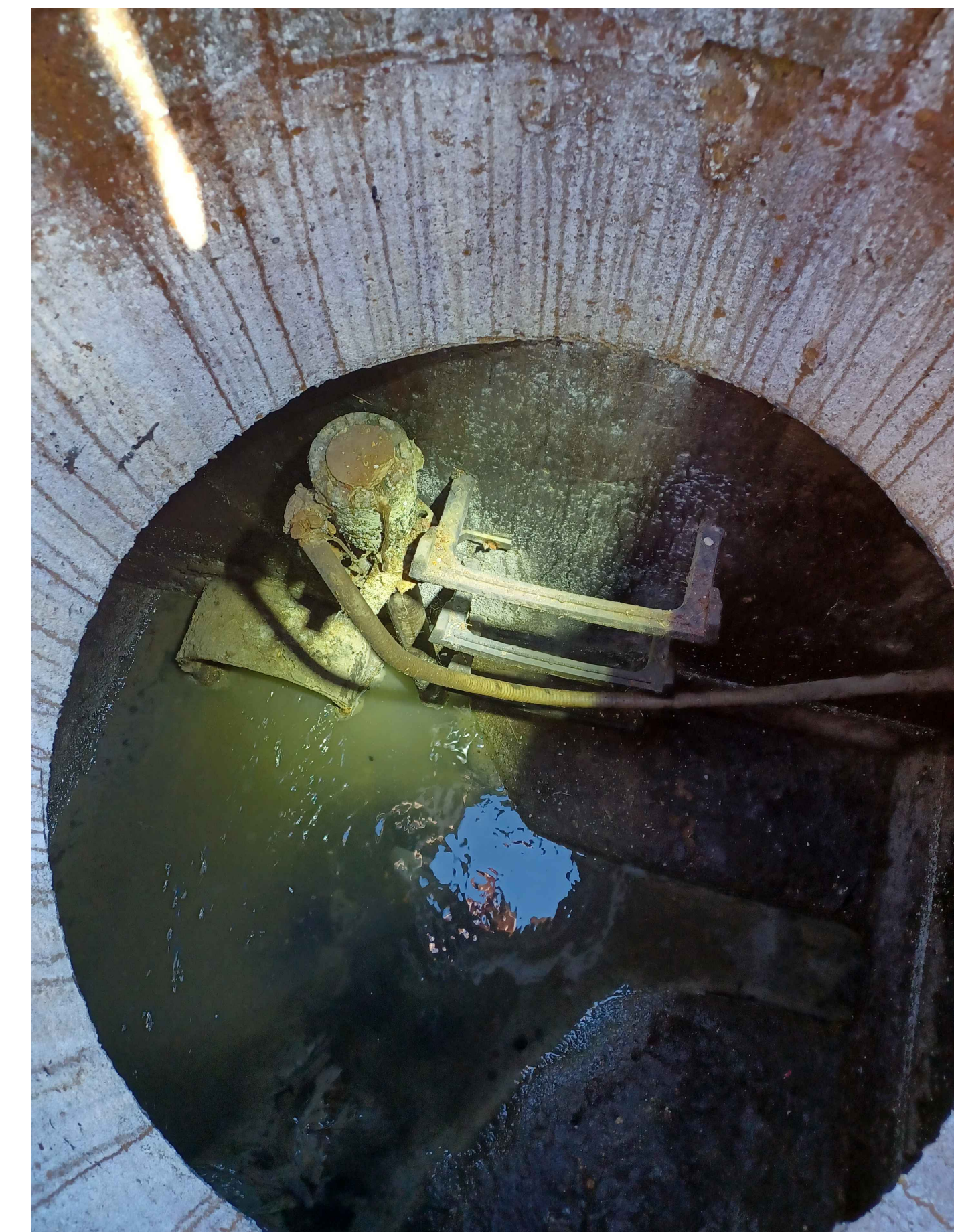
PHOTO 8 - PALMER AVE. TANK DIVERSION CHAMBER LEVEL SENSOR
