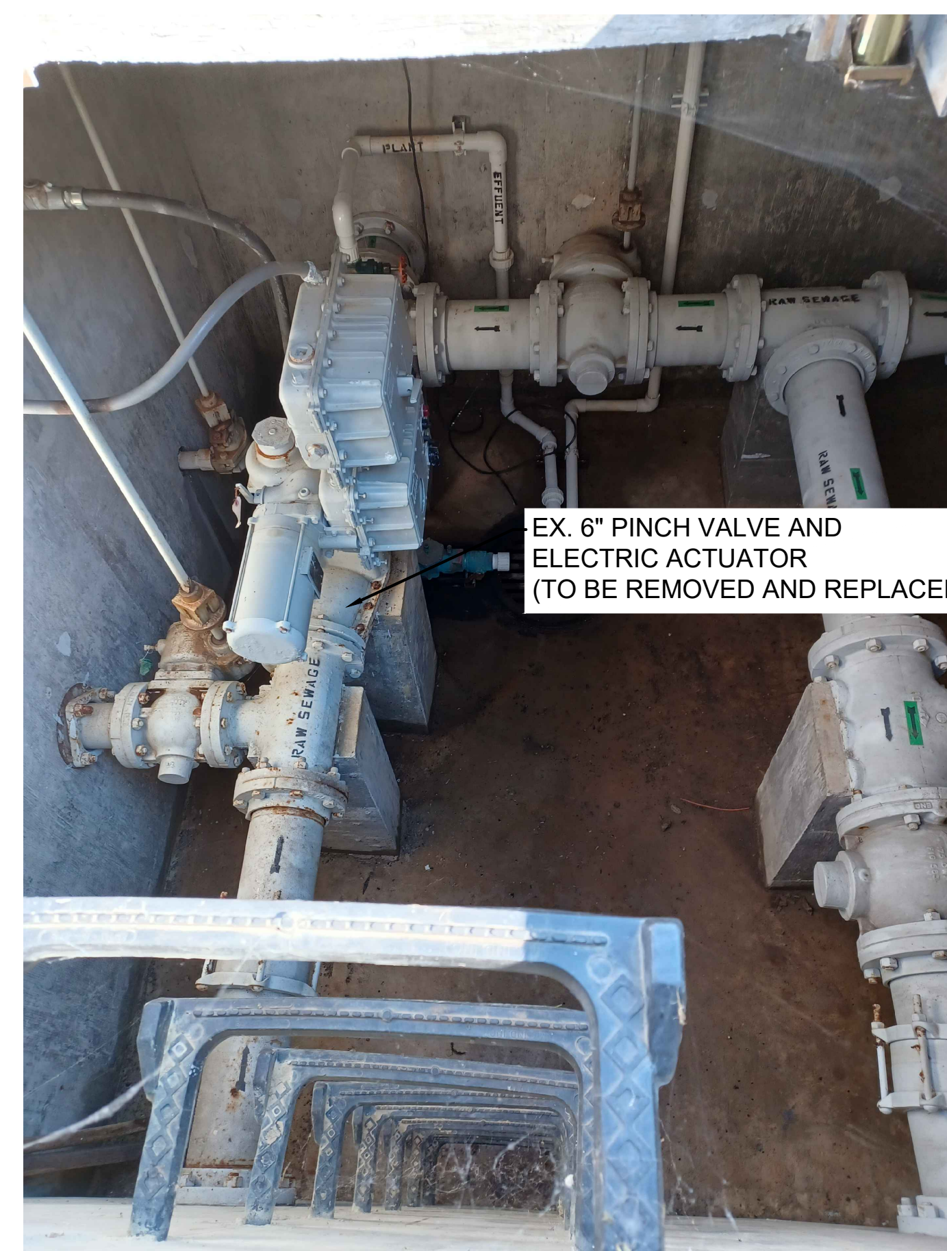
PHOTO 5 - PALMER AVE. TANK VALVE VAULT
