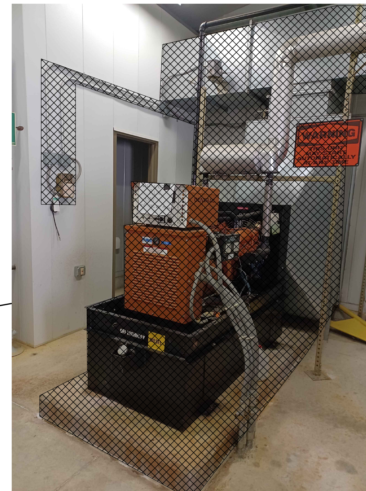
PHOTO 10 - PALMER AVE. TANK EXISTING GENERATOR
