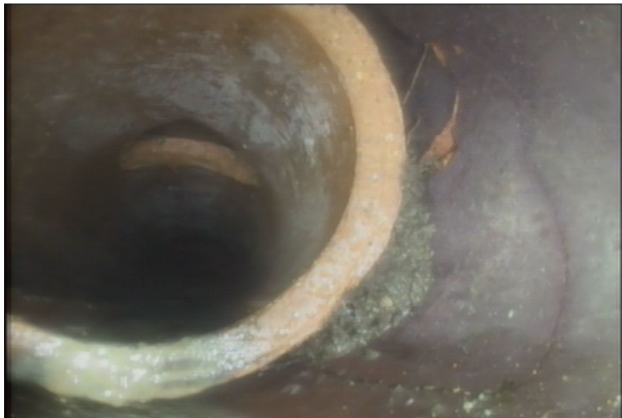
2, 00:04:02, 74.50ft Tap Factory Made, at 09 o'clock, -, within 8 inches of joint: YES, 6" / HOUSE NUMBER 186
