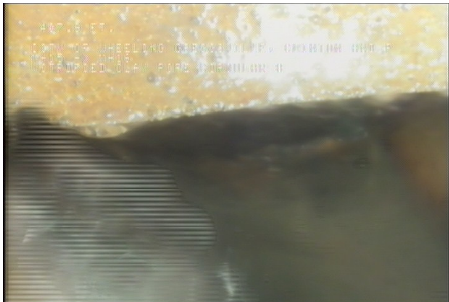
10, 00:25:58, 407.90ft Tap Factory Made, at 09 o'clock, -, within 8 inches of joint: YES, 6"
