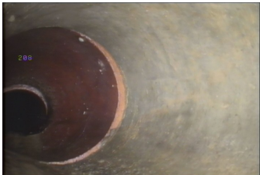
2, 00:02:29, 25.80ft Tap Factory Made, at 09 o'clock, -, within 8 inches of joint: YES, 6" / HOUSE NUMBER 208
