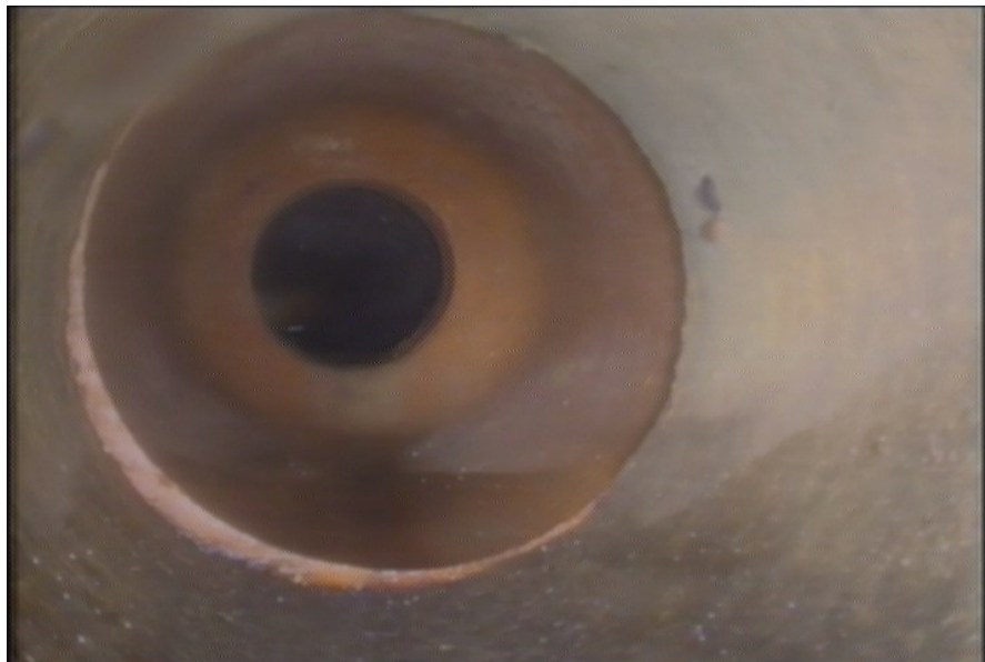
6, 00:15:25, 302.20ft Tap Factory Made, at 09 o'clock, -, within 8 inches of joint: YES, 6" / HOUSE NUMBER 228
