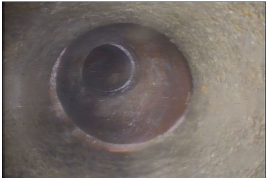
4, 00:08:59, 143.80ft Tap Factory Made, at 11 o'clock, -, within 8 inches of joint: YES, 6"
