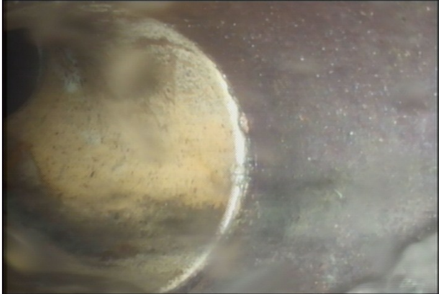
3, 00:08:53, 96.80ft Tap Factory Made, at 09 o'clock, -, within 8 inches of joint: YES, 6" / HOUSE NUMBER 156
