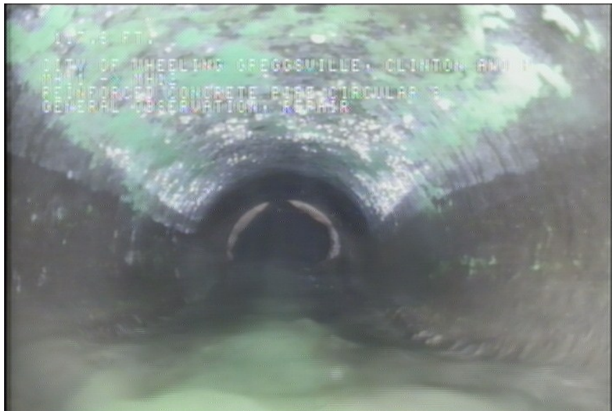
4, 00:08:02, 117.60ft General Observation / REPAIR
