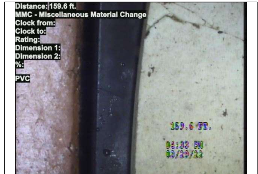
At: 159.6 ft. MMC - Miscellaneous Material Change Joint: No PVC
