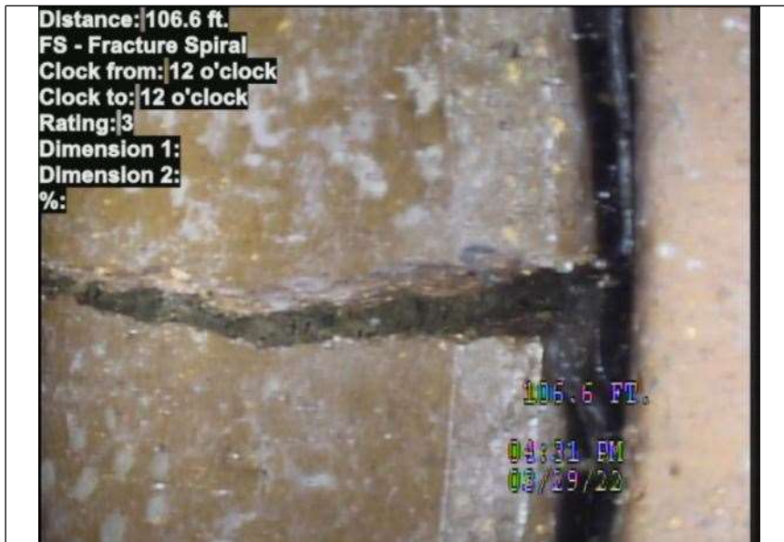
At: 106.6 ft. FS - Fracture Spiral 12/12 Joint: No
