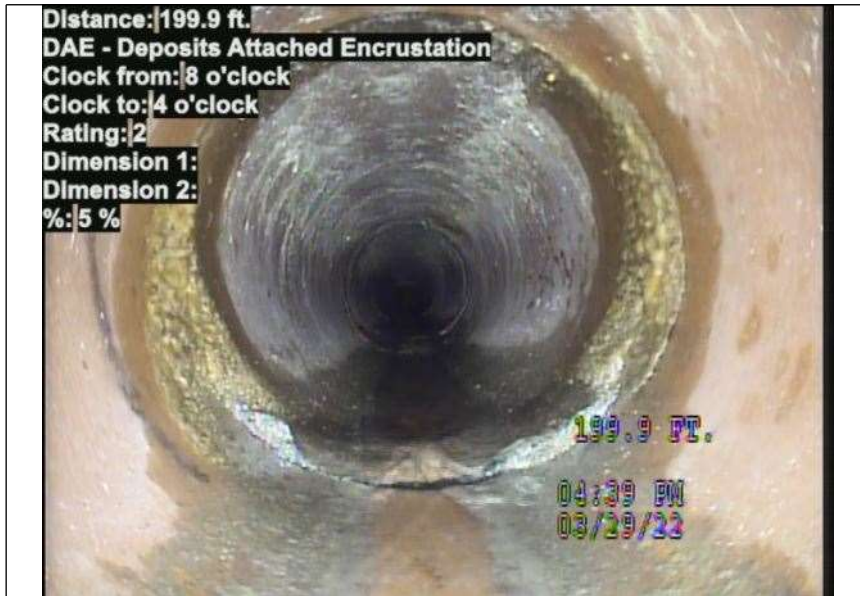
At: 199.9 ft. 8/4 DAE - Deposits Attached Encrustation Joint: No 5 %
