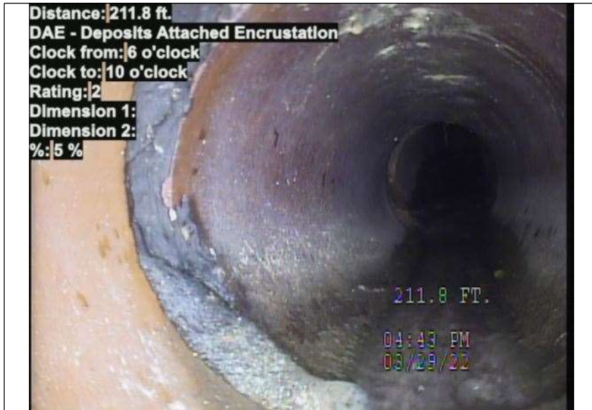
At: 211.8 ft. DAE - Deposits Attached Encrustation 6/10
