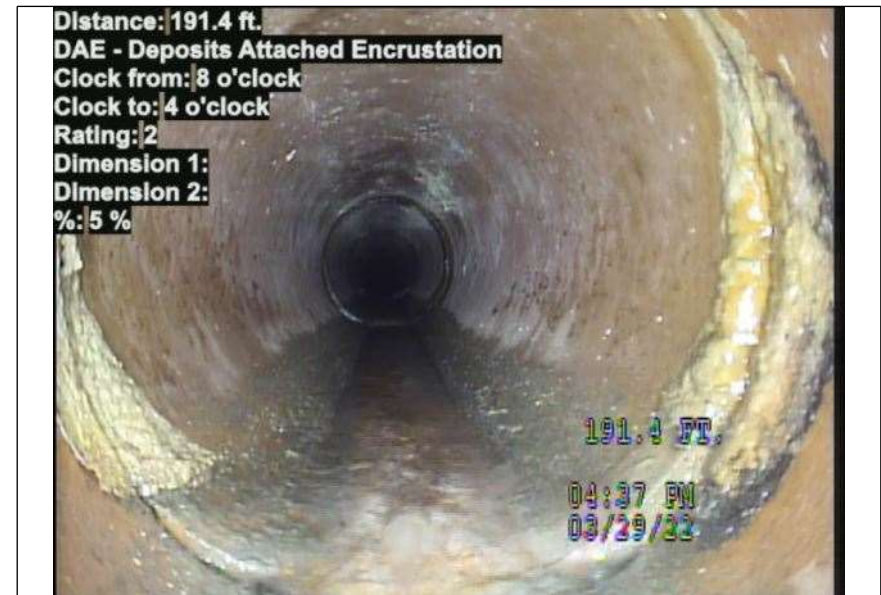
At: 191.4 ft. 8/4 DAE - Deposits Attached Encrustation Joint: No 5 %
