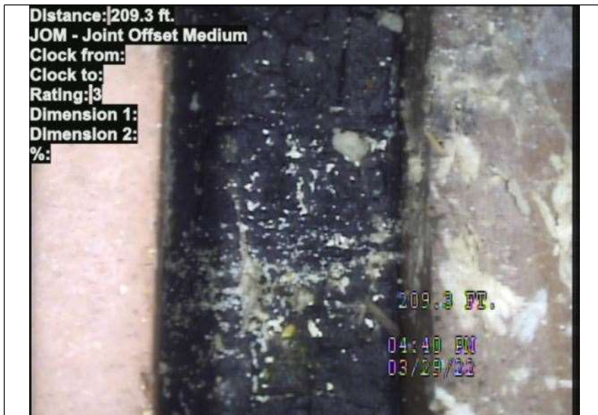
At: 209.3 ft. JOM - Joint Offset Medium Joint: No
