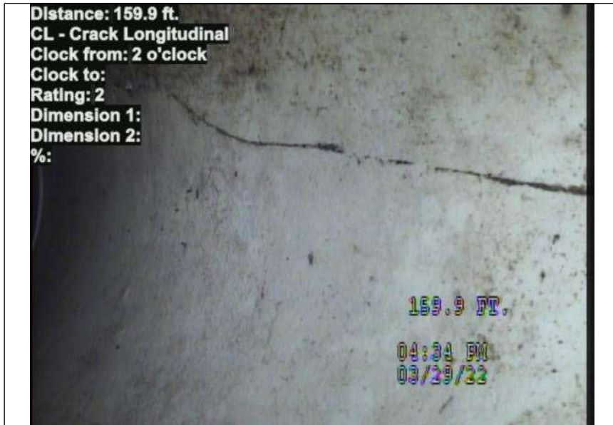
At: 159.9 ft. 2/. CL - Crack Longitudinal Joint: No
