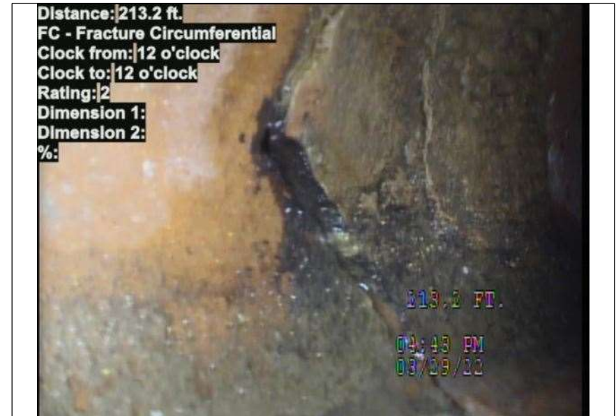
At: 213.2 ft. FC - Fracture Circumferential 12/12
