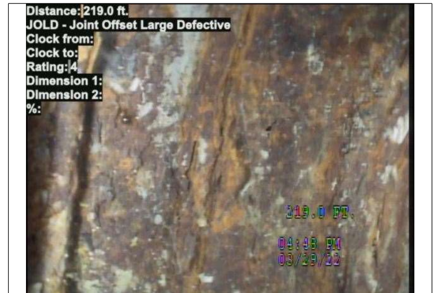
At: 219 ft. JOLD - Joint Offset Large Defective
