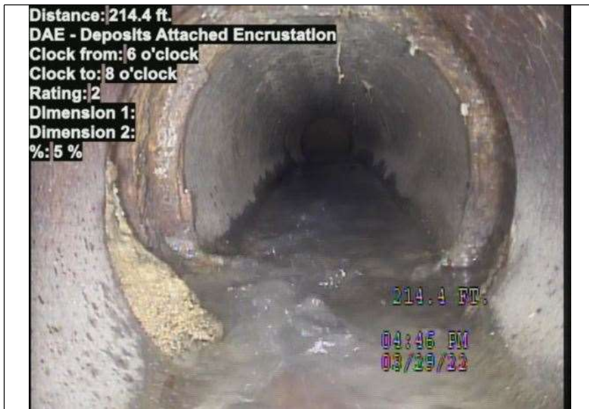
At: 214.4 ft. 6/8 DAE - Deposits Attached Encrustation
