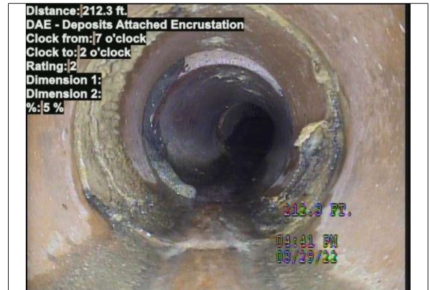
At: 211 ft. 7/2 DAE - Deposits Attached Encrustation Joint: No 5 %
