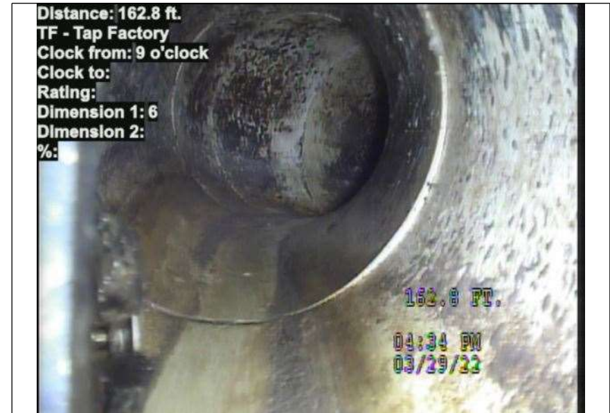
At: 162.8 ft. 9/. TF - Tap Factory Joint: No
