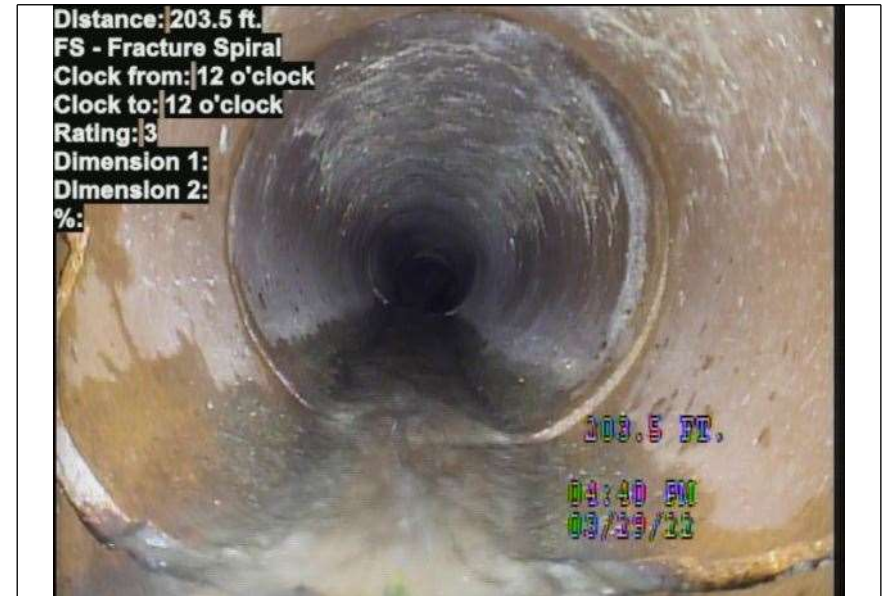
At: 203.5 ft. FC - Fracture Circumferential 12/12 Joint: No
