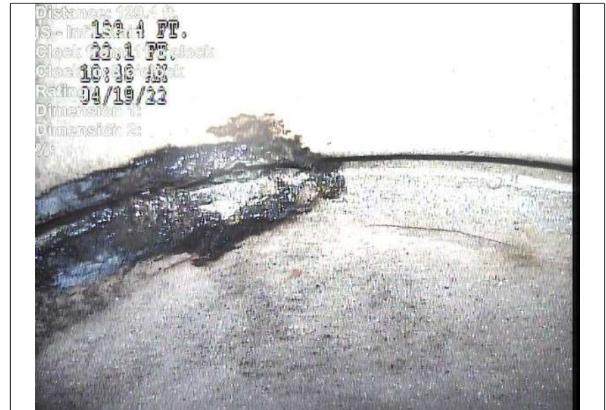
At: 129.4 ft. IS - Infil Stain 11/8 Joint: Yes
