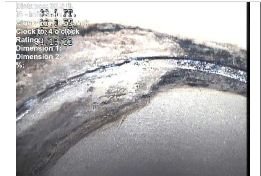
At: 38.5 ft. 8/4 IS - Infil Stain Joint: Yes
