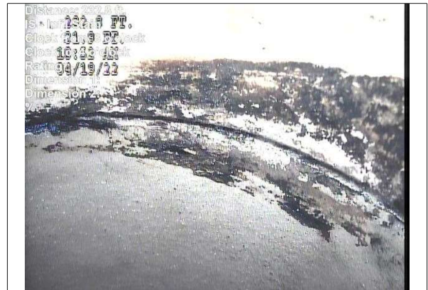
At: 232.8 ft. 8/4 IS - Infil Stain Joint: Yes
