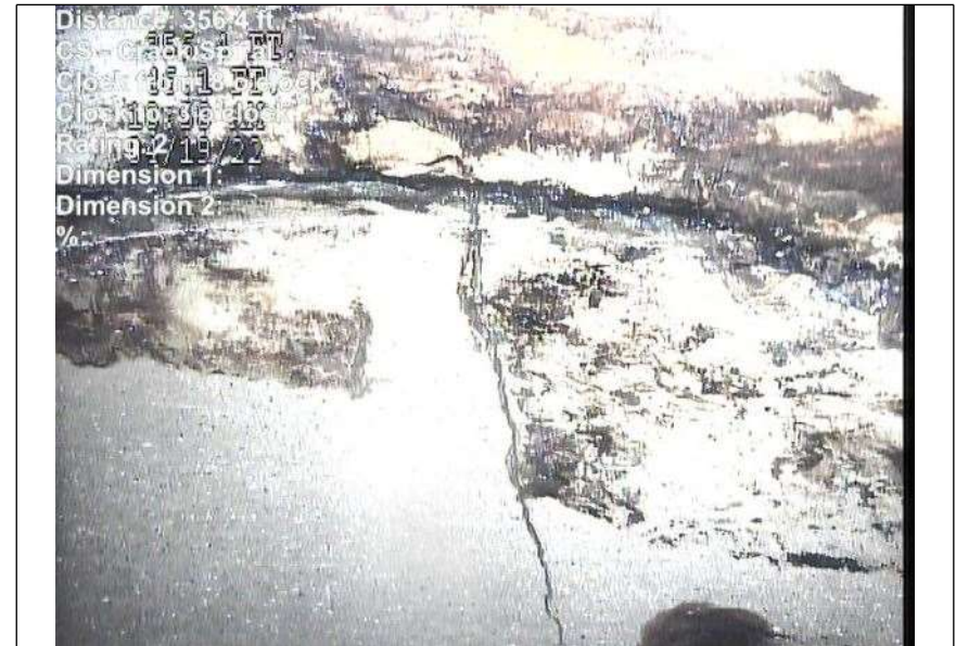
At: 356.4 ft. 8/3 CS - Crack Spiral Joint: Yes
