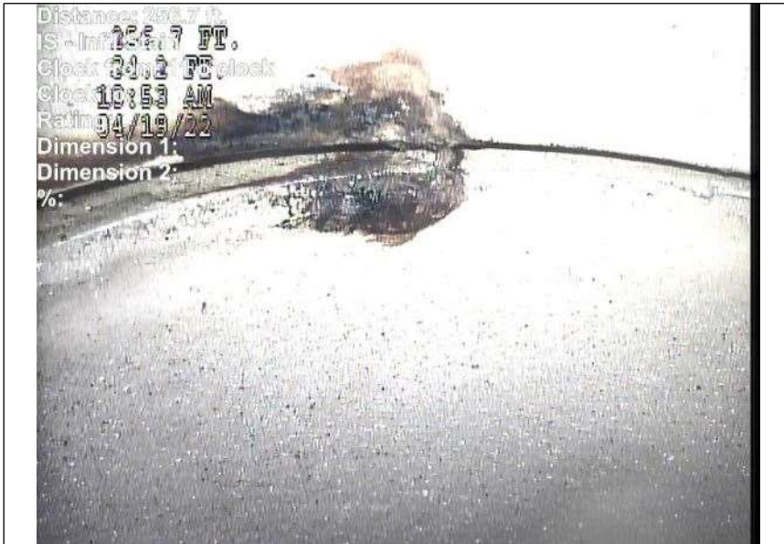
At: 256.7 ft. 11/ IS - Infil Stain Joint: Yes
