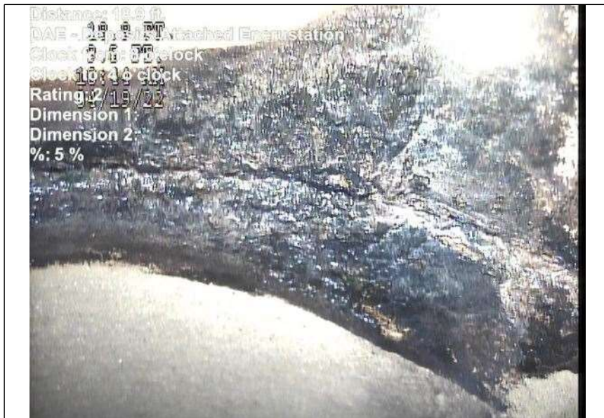
At: 18.9 ft. 8/4 DAE - Deposits Attached Encrustation Joint: Yes 5 %
