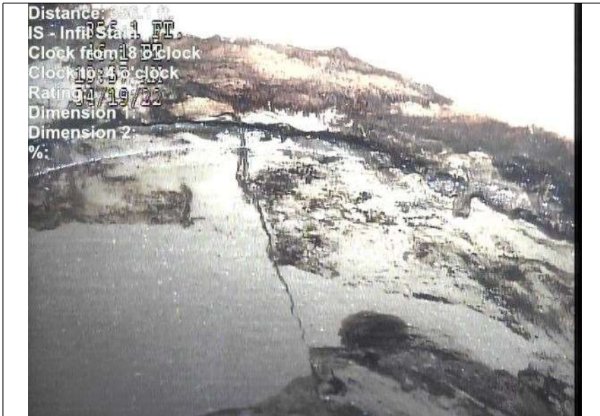
At: 356.1 ft. 8/4 IS - Infil Stain Joint: Yes
