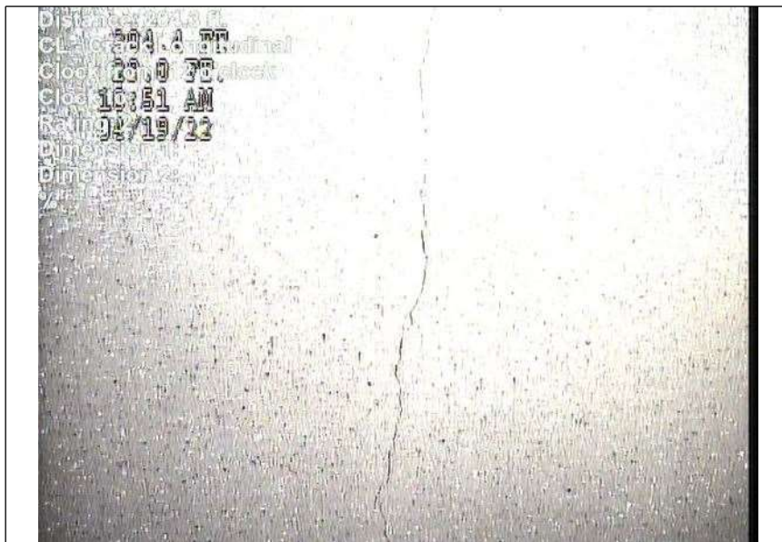
At: 204.3 ft. 12/ CL - Crack Longitudinal Joint: No
