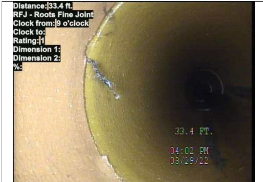
At: 33.4 ft. 9/. RFJ - Roots Fine Joint Joint: Yes
