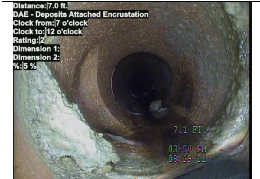
At: 7 ft. 7/5 DAE - Deposits Attached Encrustation Joint: No 5 %
