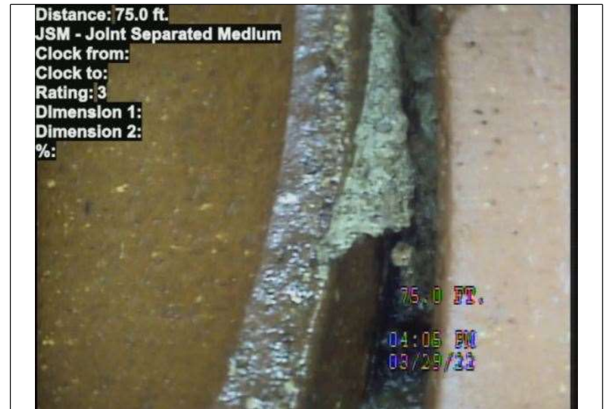
At: 75 ft. JSM - Joint Separated Medium Joint: No
