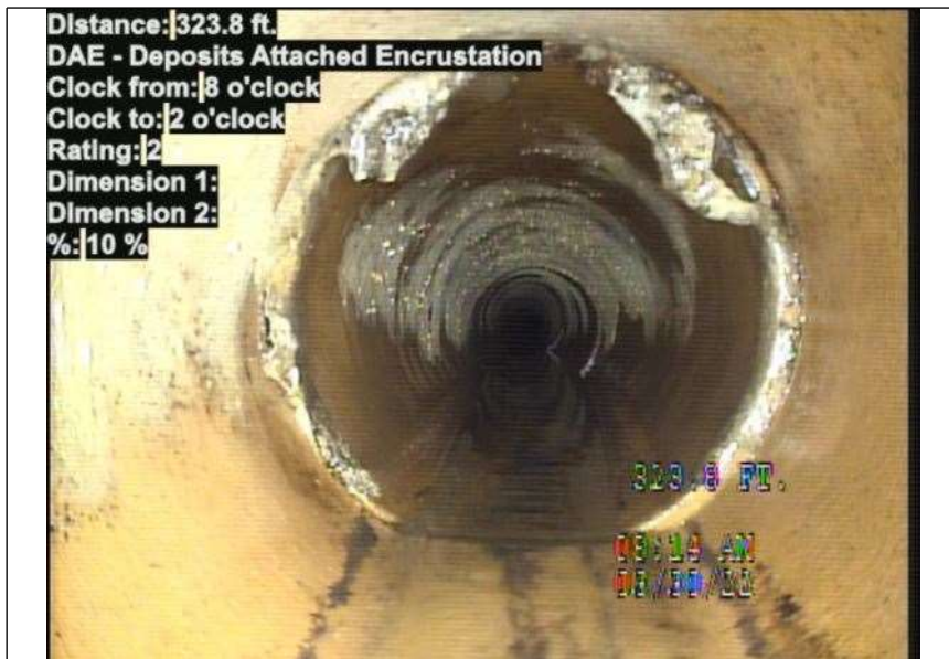
At: 323.8 ft. 8/2 DAE - Deposits Attached Encrustation Joint: No 10 %
