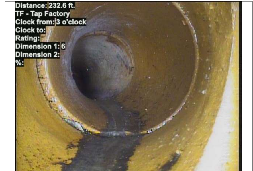
At: 232.6 ft. 3/. TF - Tap Factory
