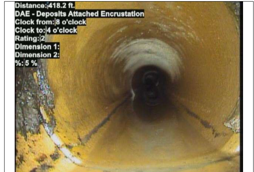
At: 418.2 ft. 8/4 DAE - Deposits Attached Encrustation Joint: No 5 %
