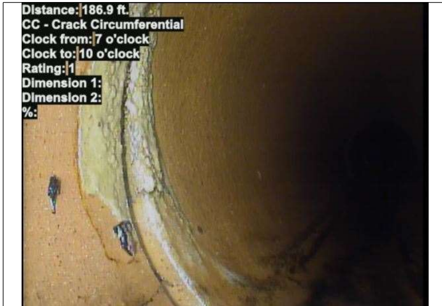
At: 186.9 ft. CC - Crack Circumferential 7/10
