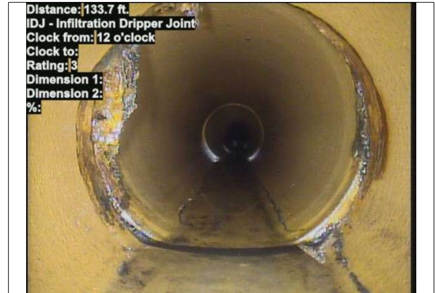
At: 133.7 ft. 12/ IDJ - Infiltration Dripper Joint
