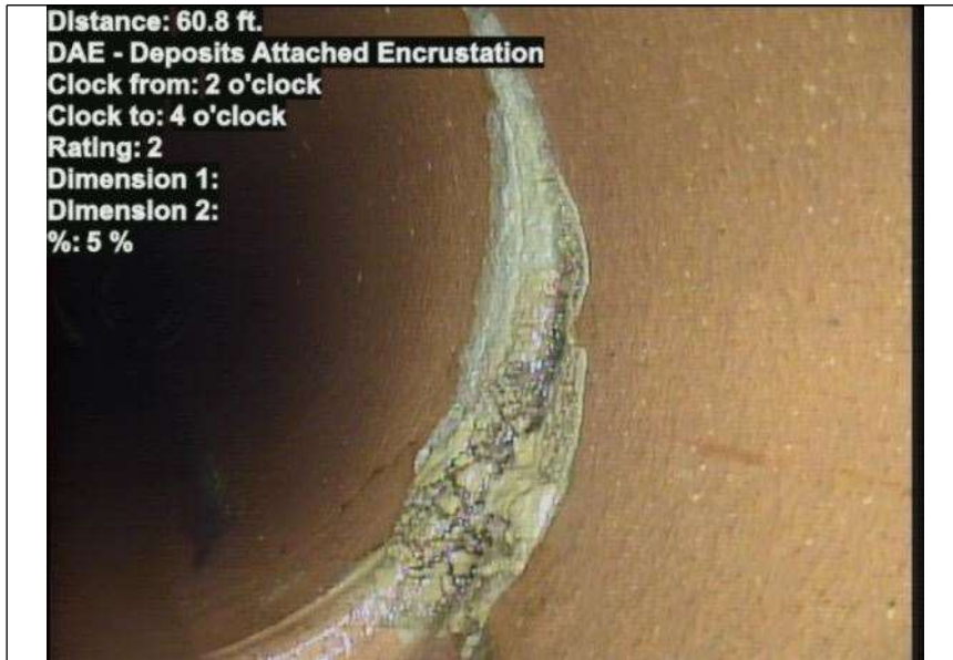
At: 60.8 ft. 2/4 DAE - Deposits Attached Encrustation Joint: No 5 %
