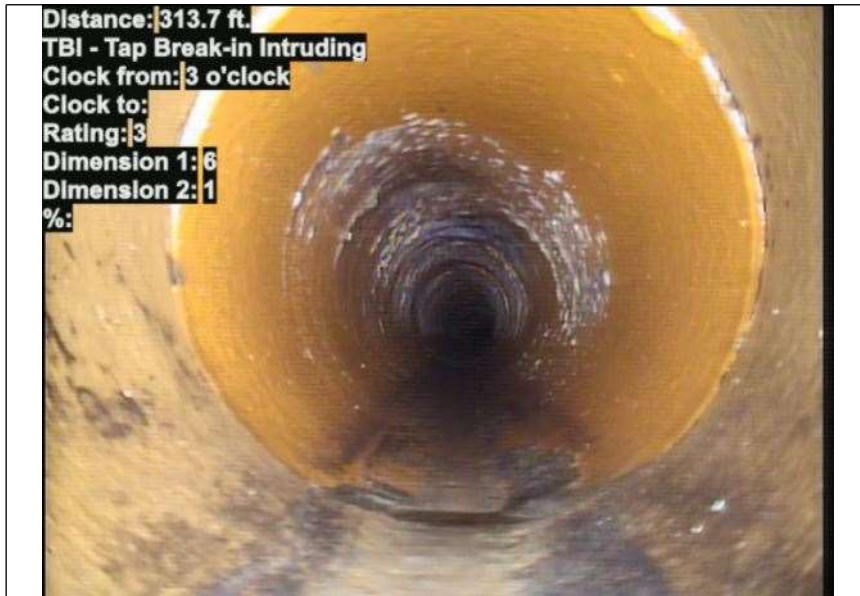
At: 313.7 ft. 3/ TBI - Tap Break-in Intruding Joint: No
