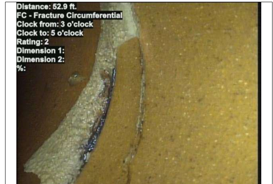
At: 52.9 ft. 3/5 FC - Fracture Circumferential Joint: No
