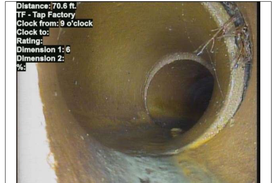
At: 70.6 ft. 9/ TF - Tap Factory Joint: No
