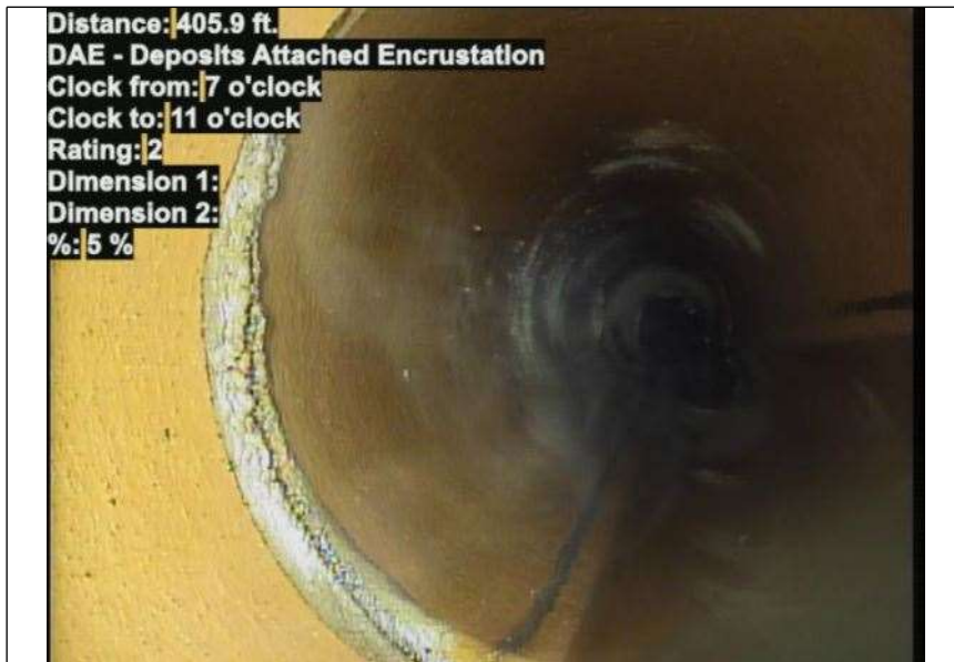
At: 405.9 ft. DAE - Deposits Attached Encrustation 7/11 Joint: No 5 %
