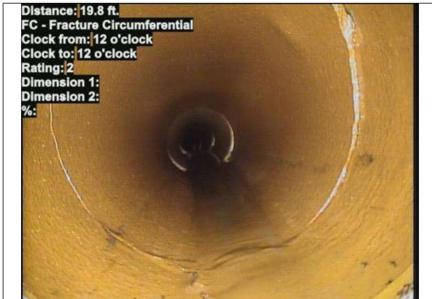
At: 19.8 ft. FC - Fracture Circumferential 12/12 Joint: No
