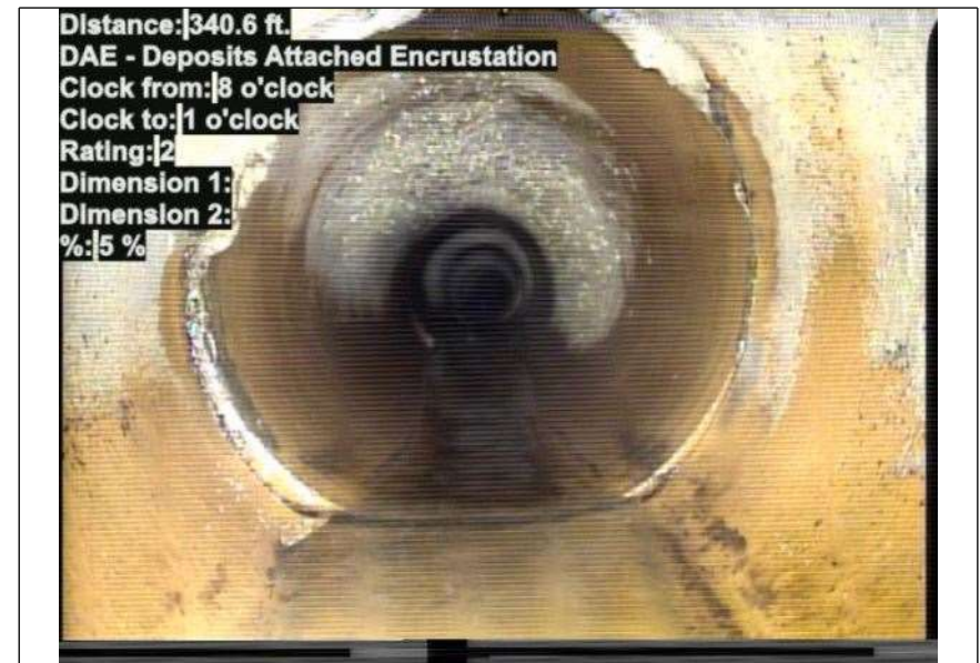
At: 340.6 ft. 8/1 DAE - Deposits Attached Encrustation Joint: No 5 %
