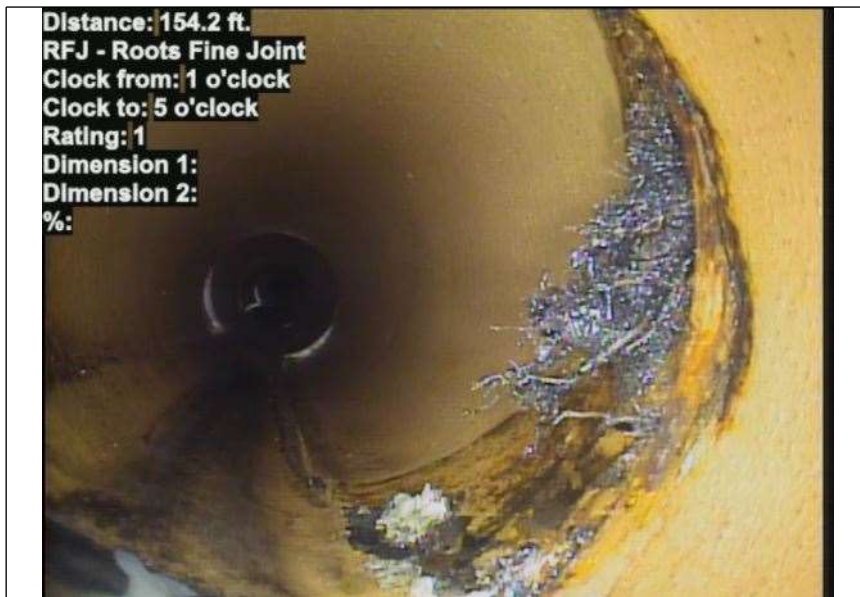
At: 154.2 ft. 1/5 RFJ - Roots Fine Joint
