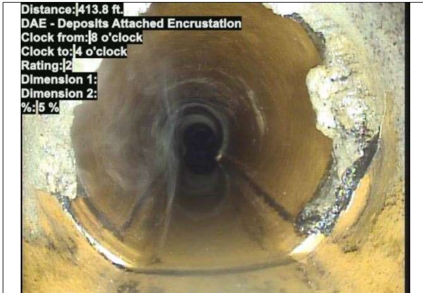
At: 413.8 ft. 8/4 DAE - Deposits Attached Encrustation Joint: No 10 %
