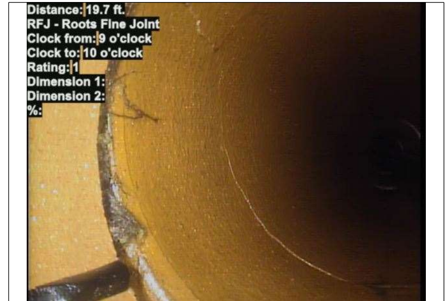
At: 19.7 ft. 9/10 RFJ - Roots Fine Joint Joint: Yes
