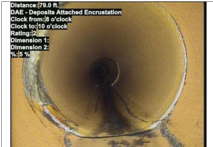
At: 79 ft. 8/10 DAE - Deposits Attached Encrustation Joint: No 5 %
