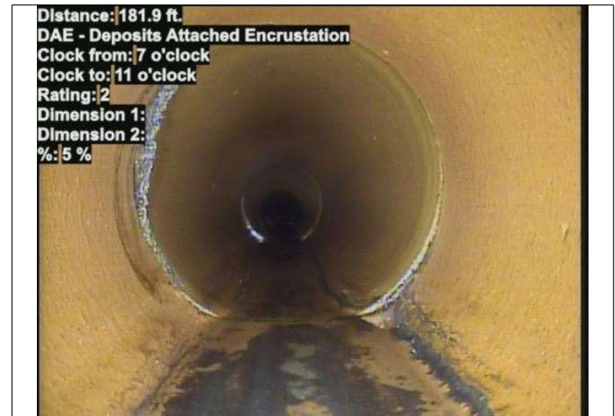
At: 181.9 ft. DAE - Deposits Attached Encrustation 7/11
