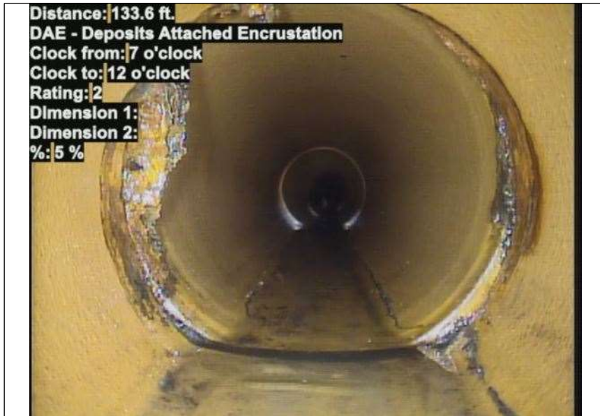
At: 133.6 ft. DAE - Deposits Attached Encrustation 7/12
