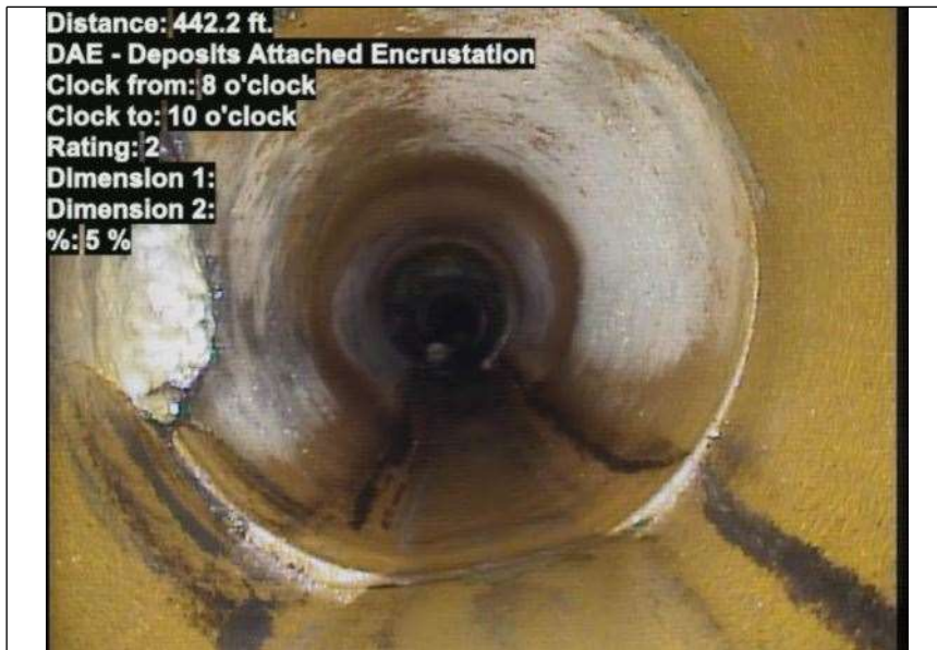
At: 442.2 ft. DAE - Deposits Attached Encrustation 8/10 Joint: No 5 %
