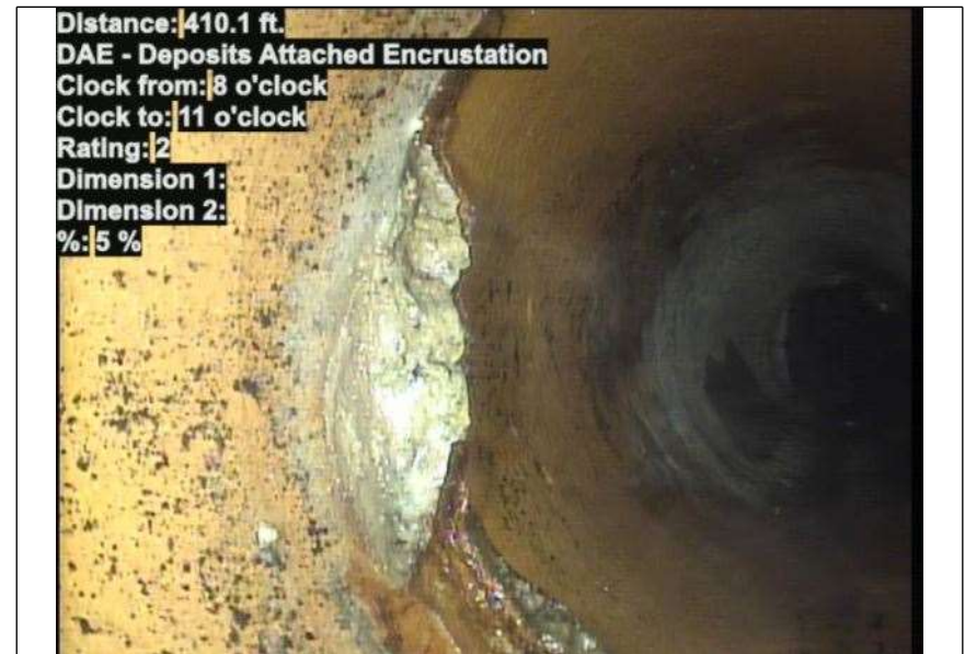
At: 410.1 ft. DAE - Deposits Attached Encrustation 8/11 Joint: No 5 %
