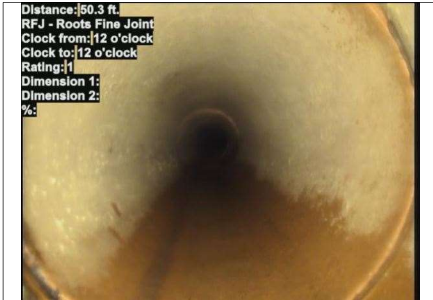
At: 50.3 ft. RFJ - Roots Fine Joint 12/12
