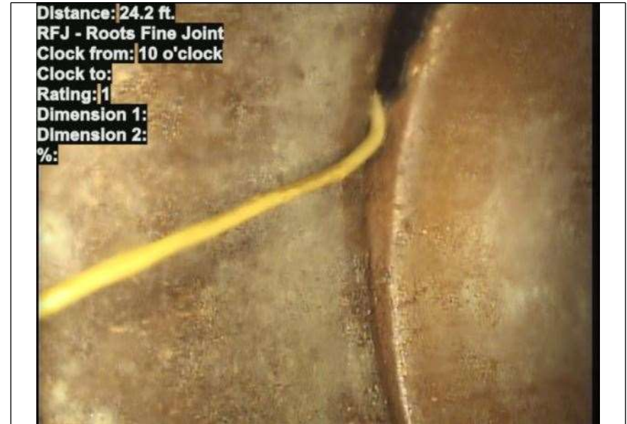
At: 24.2 ft. 10/. RFJ - Roots Fine Joint Joint: Yes
