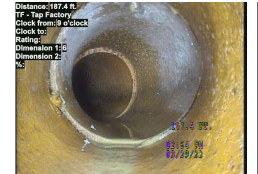
At: 187.4 ft. 9/. TF - Tap Factory
