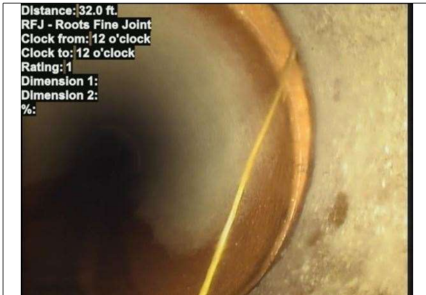
At: 32 ft. 12/12 RFJ - Roots Fine Joint Joint: Yes
