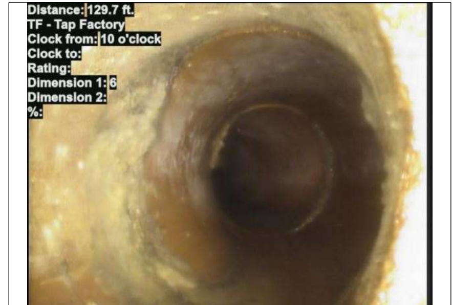
At: 129.7 ft. 10/. TF - Tap Factory
