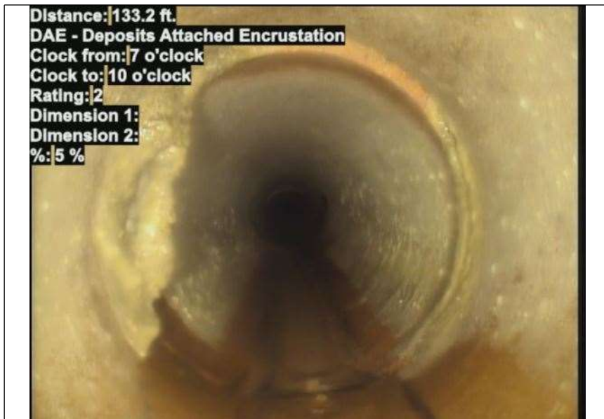
At: 133.2 ft. DAE - Deposits Attached Encrustation 7/10
