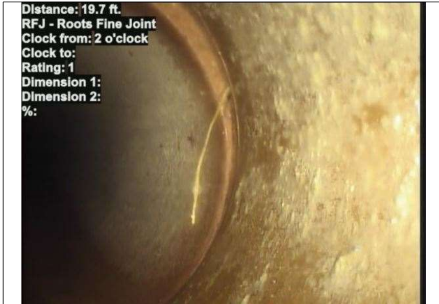
At: 19.7 ft. 2/. RFJ - Roots Fine Joint Joint: Yes
