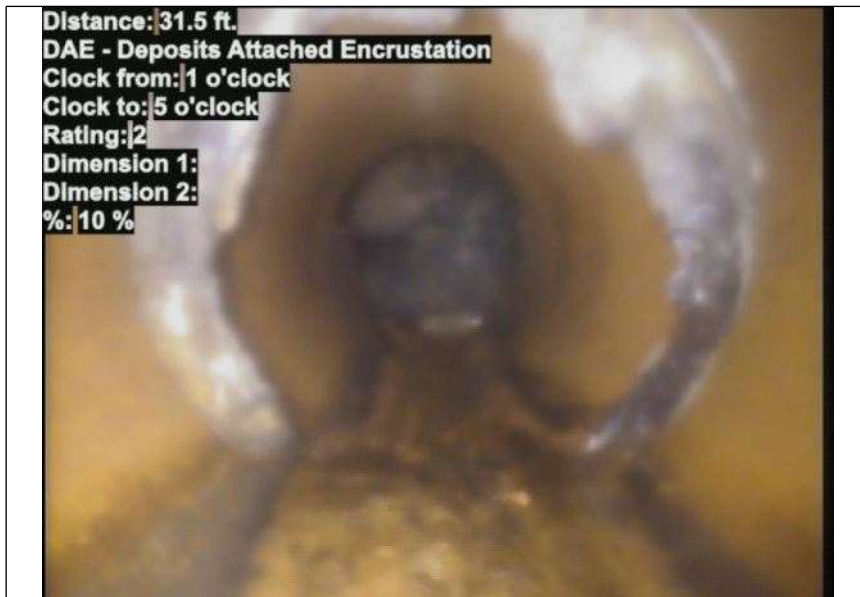
At: 31.5 ft. 1/5 DAE - Deposits Attached Encrustation Joint: No 10 %
