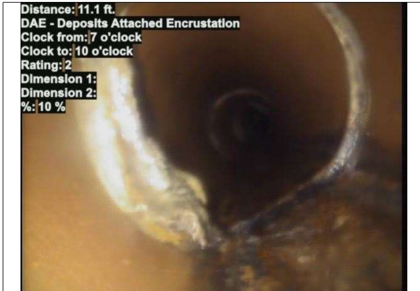
At: 11.1 ft. 7/10 DAE - Deposits Attached Encrustation Joint: No 10 %
