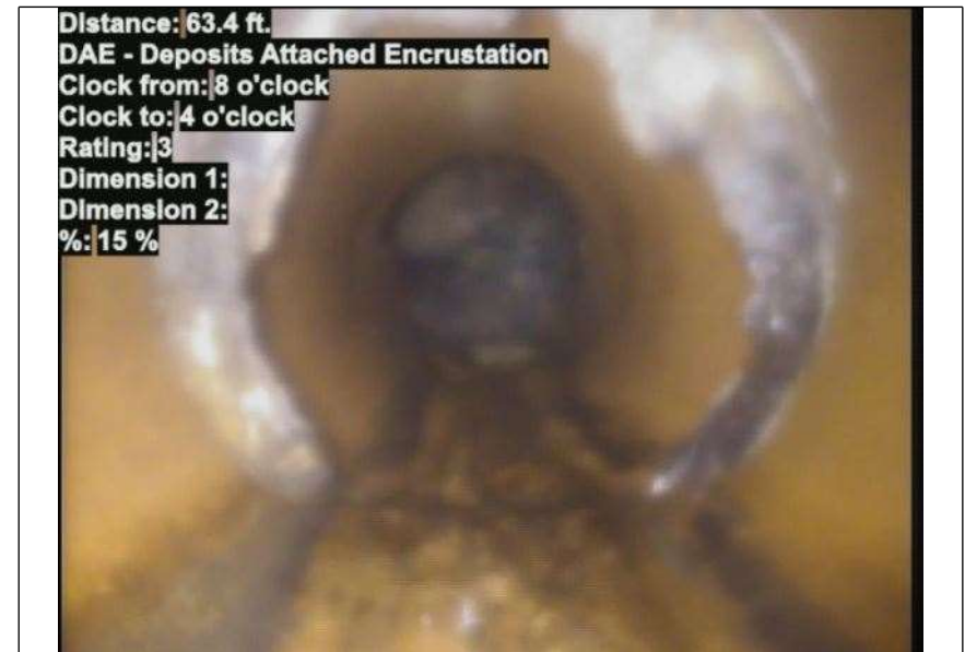
At: 63.4 ft. 8/4 DAE - Deposits Attached Encrustation Joint: No 15 %
