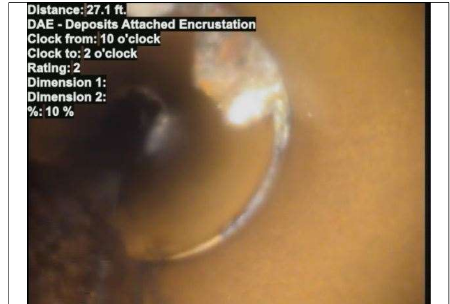
At: 27.1 ft. 10/2 DAE - Deposits Attached Encrustation Joint: No 10 %
