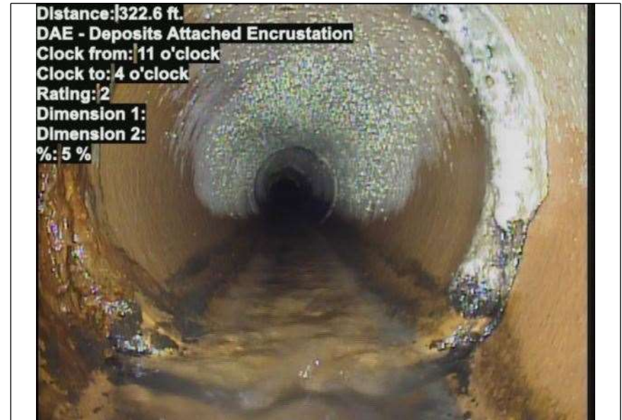
At: 322.6 ft. 11/4 DAE - Deposits Attached Encrustation Joint: No 5 %
