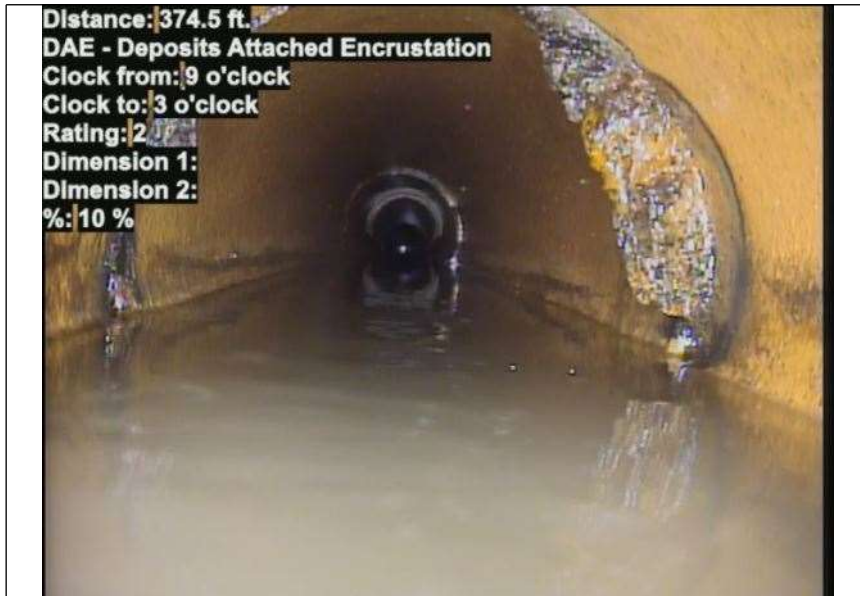
At: 374.5 ft. 9/3 DAE - Deposits Attached Encrustation
