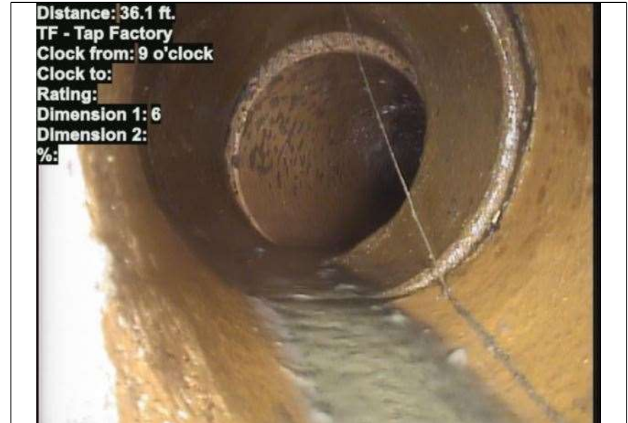
At: 36.1 ft. 9/ TF - Tap Factory Joint: No
