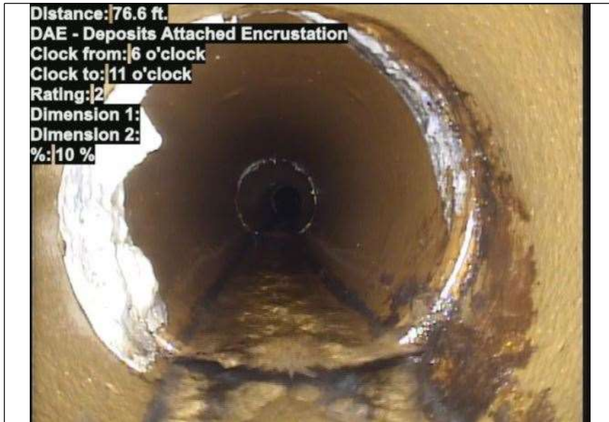
At: 76.6 ft. 6/11 DAE - Deposits Attached Encrustation Joint: No 10 %
