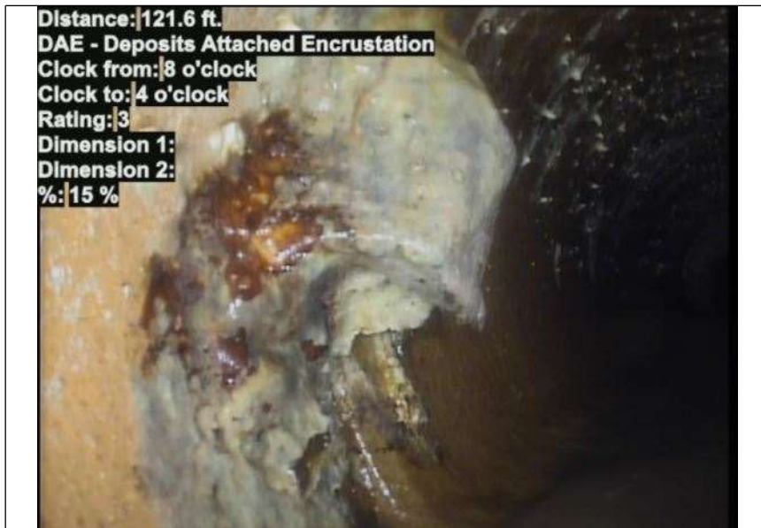
At: 121.6 ft. 8/4 DAE - Deposits Attached Encrustation Joint: No 15 %
