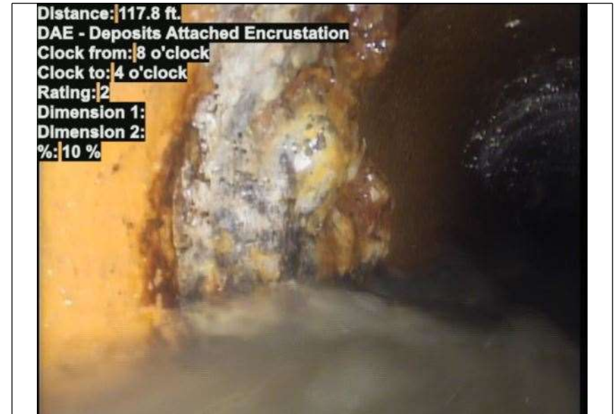
At: 117.8 ft. 8/4 DAE - Deposits Attached Encrustation Joint: No 10 %
