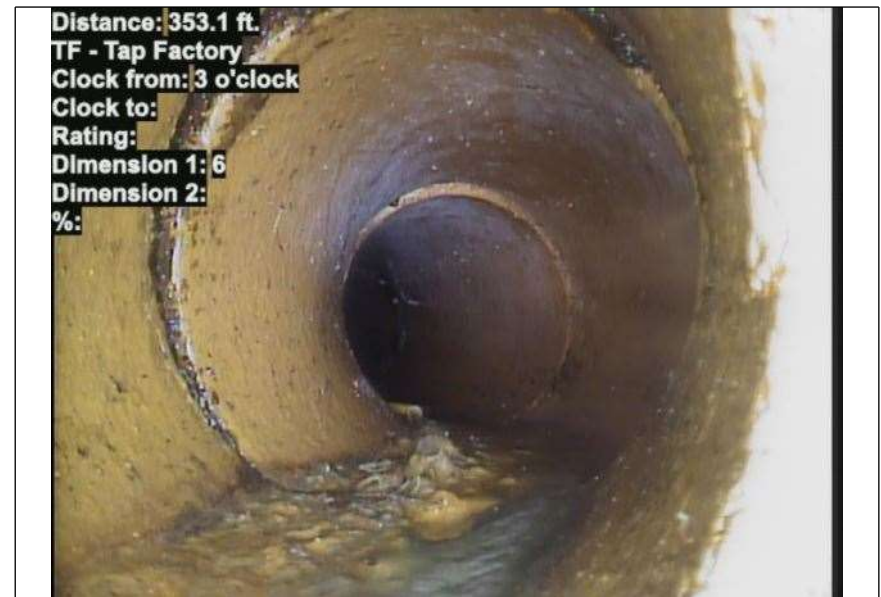
At: 353.1 ft. 3/ TF - Tap Factory Joint: No
