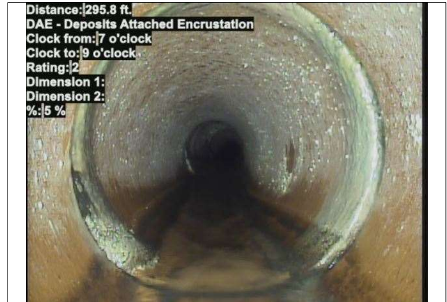
At: 295.8 ft. 7/9 DAE - Deposits Attached Encrustation Joint: No 5 %
