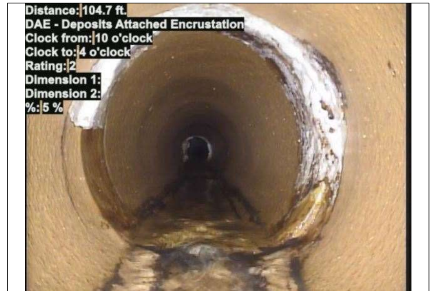
At: 104.7 ft. 10/4 DAE - Deposits Attached Encrustation Joint: No 5 %
