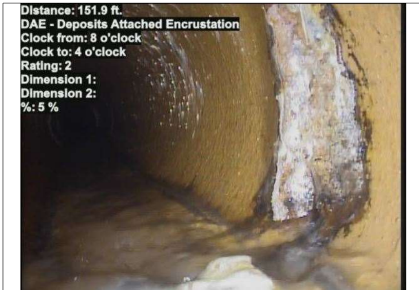
At: 151.9 ft. 8/4 DAE - Deposits Attached Encrustation Joint: No 5 %
