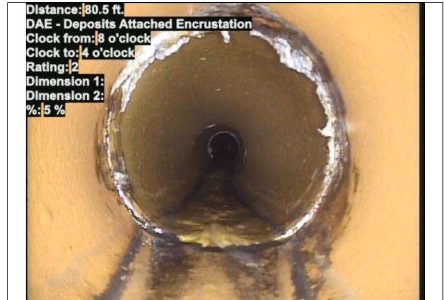
At: 80.5 ft. 8/4 DAE - Deposits Attached Encrustation Joint: No 5 %
