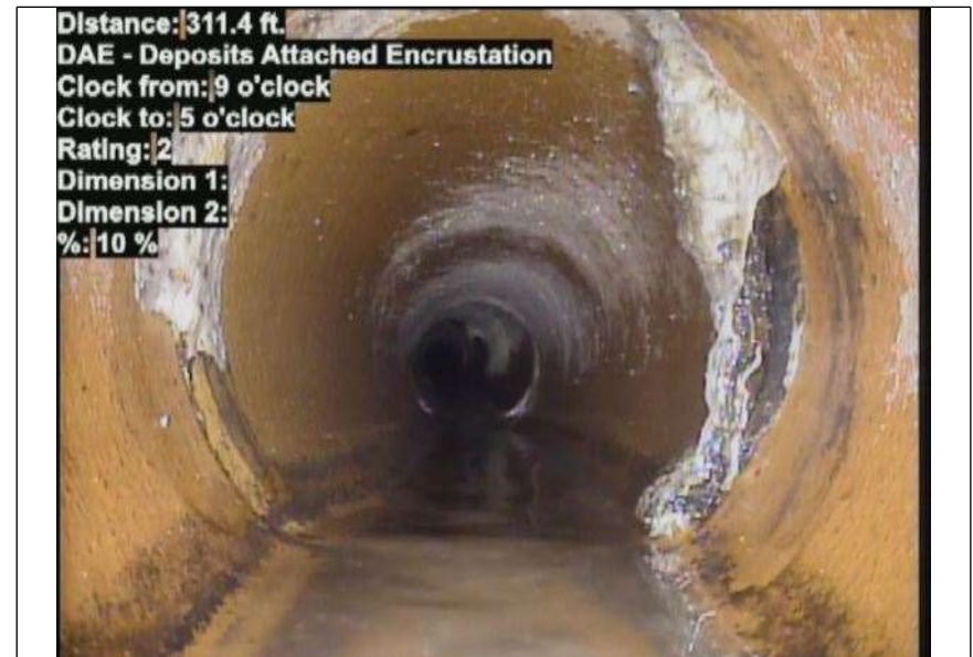
At: 311.4 ft. 9/5 DAE - Deposits Attached Encrustation Joint: No 10 %
