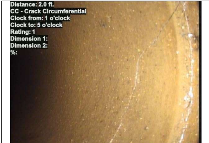
At: 2 ft. 1/5 CC - Crack Circumferential Joint: No
