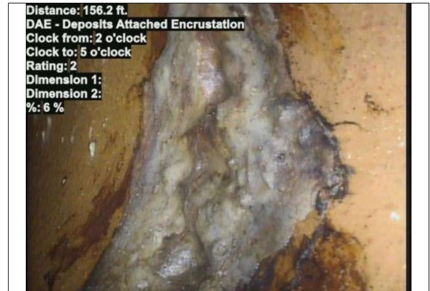
At: 156.2 ft. 2/5 DAE - Deposits Attached Encrustation Joint: No 6 %
