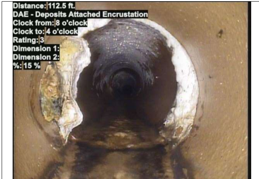
At: 112.5 ft. 8/4 DAE - Deposits Attached Encrustation Joint: No 15 %
