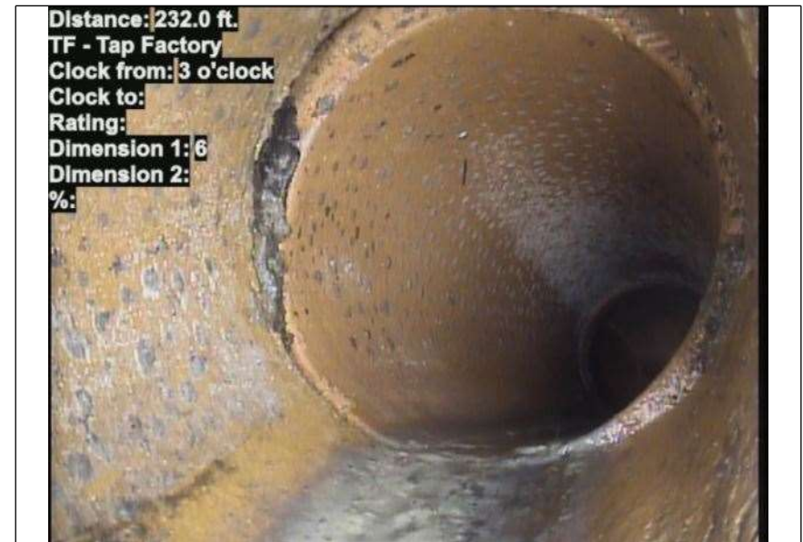
At: 232 ft. 3/. TF - Tap Factory Joint: No
