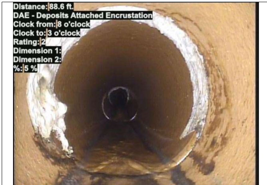
At: 88.6 ft. 8/3 DAE - Deposits Attached Encrustation Joint: No 5 %
