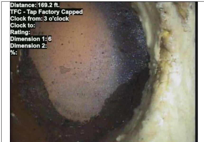
At: 169.2 ft. 3/. TFC - Tap Factory Capped Joint: No
