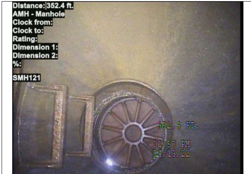
At: 352.4 ft. AMH - Manhole Joint: No SMH121
