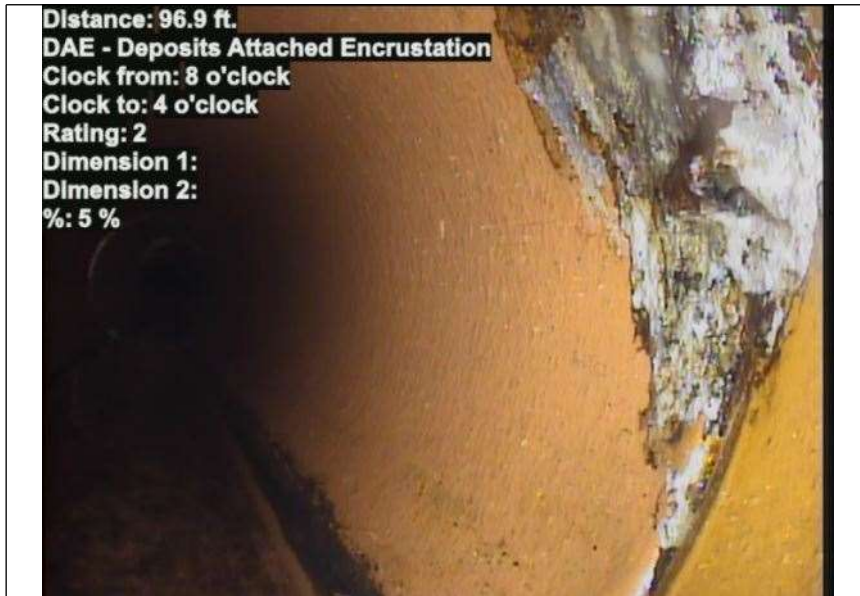
At: 96.9 ft. 8/4 DAE - Deposits Attached Encrustation Joint: No 5 %
