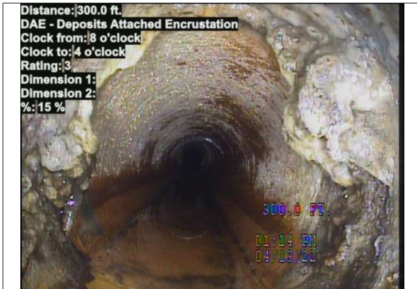
At: 300 ft. 8/4 DAE - Deposits Attached Encrustation Joint: No 15 %
