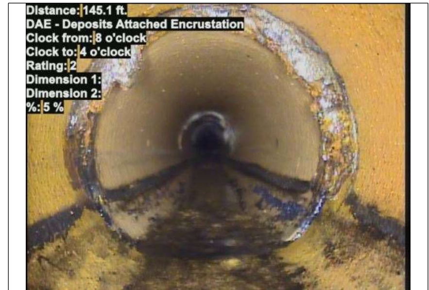
At: 145.1 ft. 8/4 DAE - Deposits Attached Encrustation Joint: No 5 %
