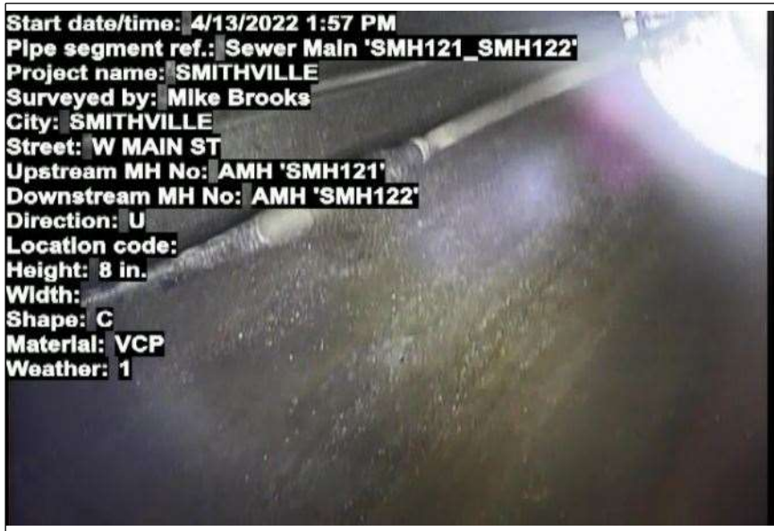
At: 0 ft. AMH - Manhole Joint: No SMH122
