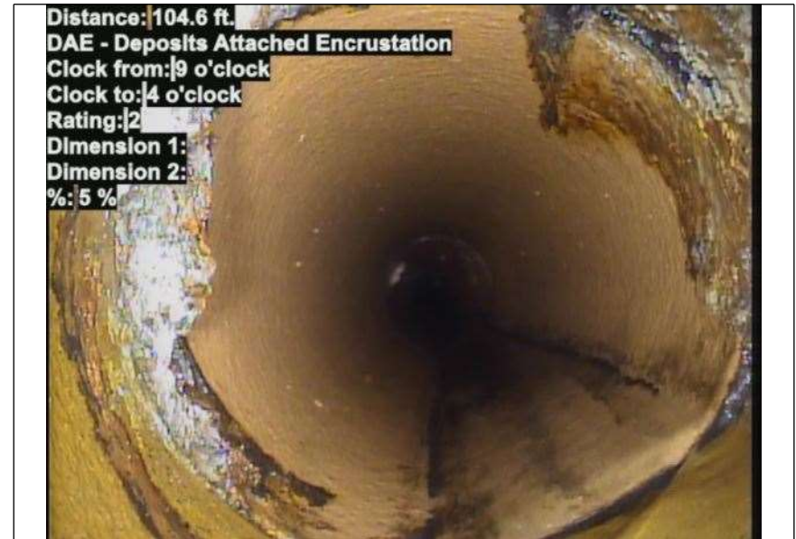
At: 104.6 ft. 9/4 DAE - Deposits Attached Encrustation Joint: No 5 %
