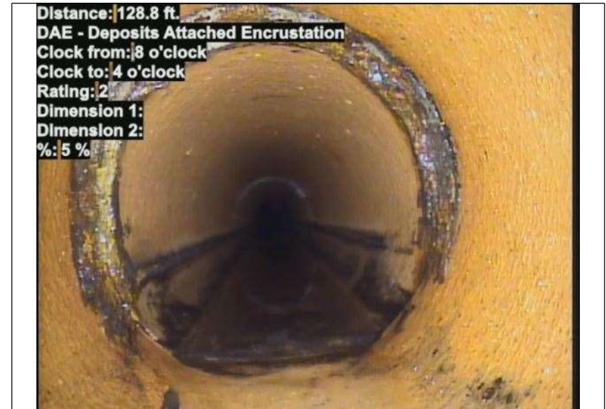
At: 128.8 ft. 8/4 DAE - Deposits Attached Encrustation Joint: No 5 %
