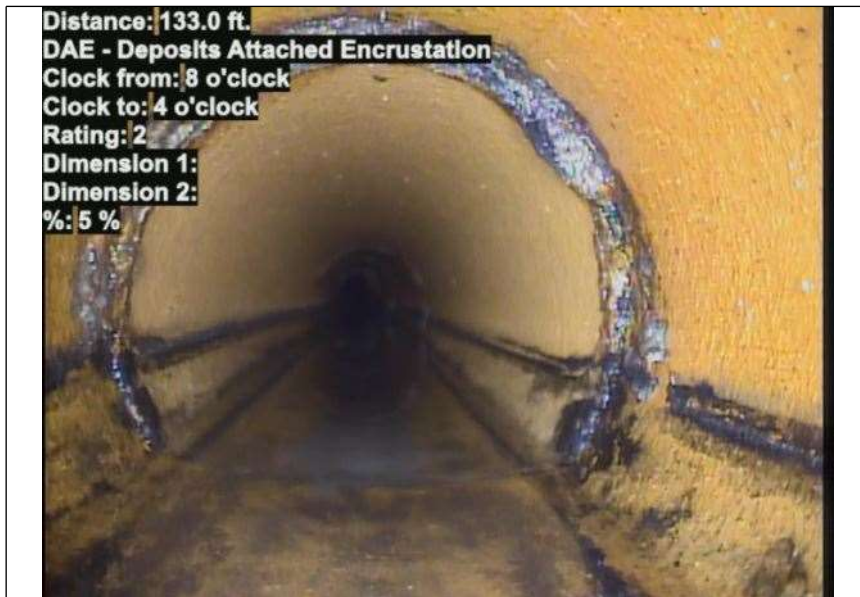
At: 133 ft. 8/4 DAE - Deposits Attached Encrustation Joint: No 5 %
