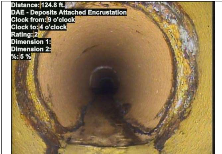
At: 124.8 ft. 9/4 DAE - Deposits Attached Encrustation Joint: No 5 %
