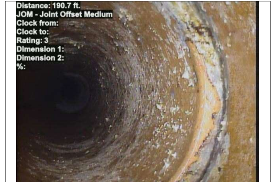
At: 190.7 ft. JOM - Joint Offset Medium Joint: No
