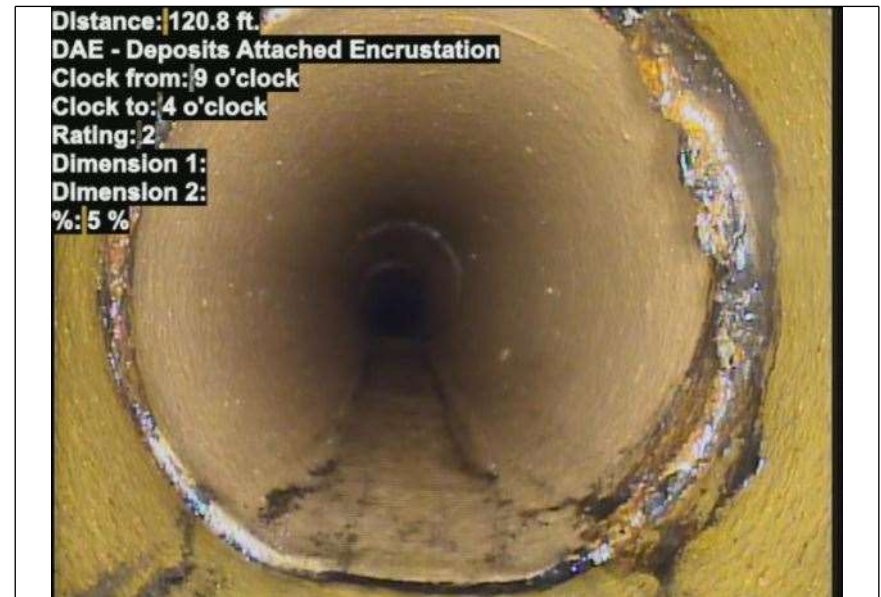
At: 120.8 ft. 9/4 DAE - Deposits Attached Encrustation Joint: No 5 %
