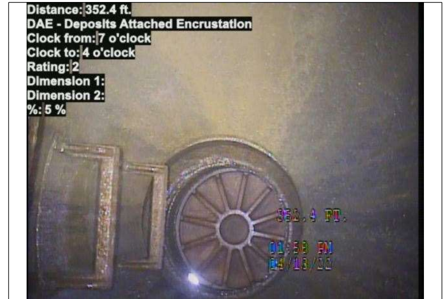
At: 352.4 ft. 7/4 DAE - Deposits Attached Encrustation Joint: No 5 %
