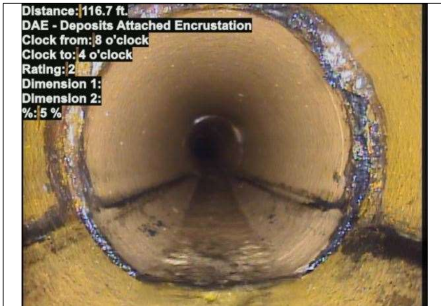
At: 116.7 ft. 8/4 DAE - Deposits Attached Encrustation Joint: No 5 %
