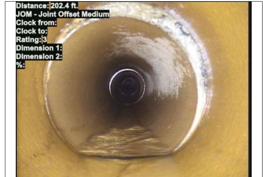
At: 202.4 ft. JOM - Joint Offset Medium Joint: No
