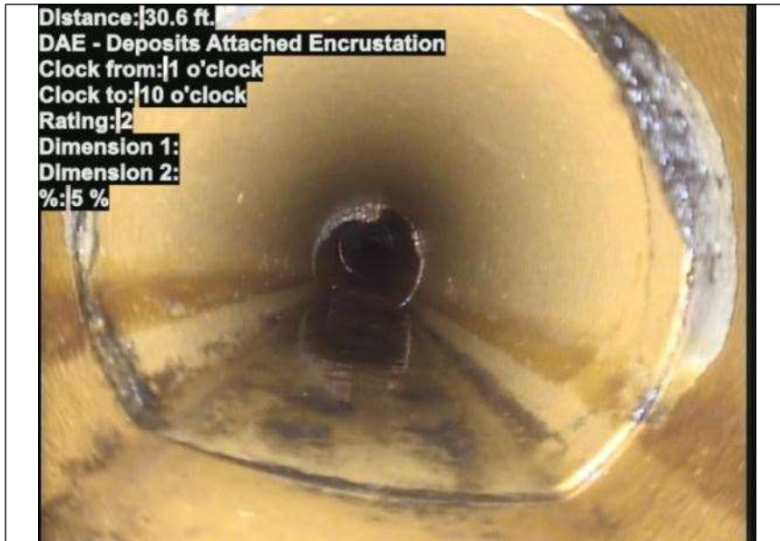
At: 30.6 ft. 1/10 DAE - Deposits Attached Encrustation Joint: No 5 %
