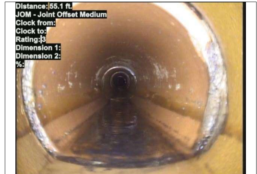
At: 55.1 ft. JOM - Joint Offset Medium Joint: No
