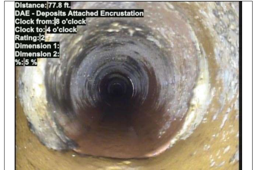
At: 77.8 ft. 8/4 DAE - Deposits Attached Encrustation Joint: No 5 %
