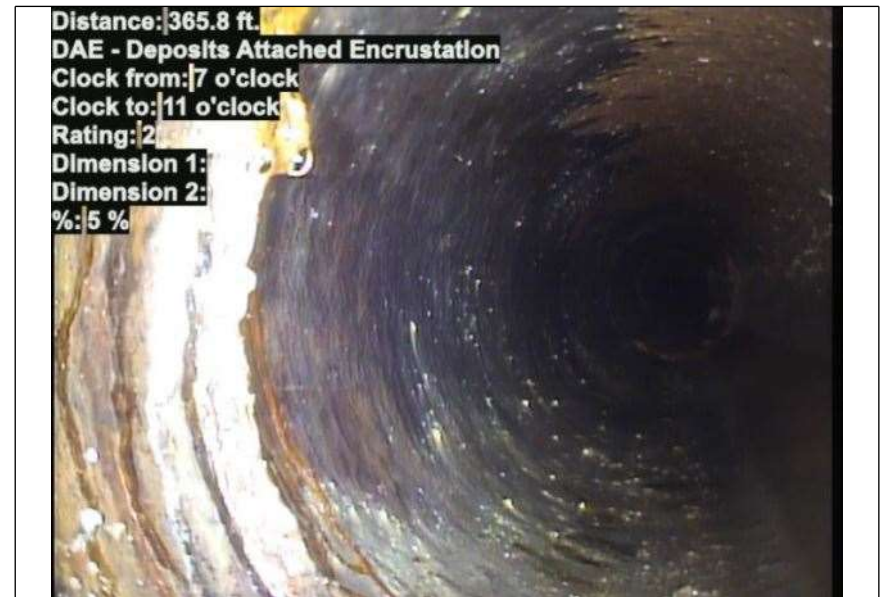
At: 365.8 ft. DAE - Deposits Attached Encrustation 7/11 Joint: No 5 %
