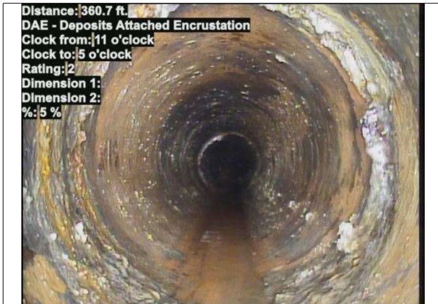
At: 360.7 ft. DAE - Deposits Attached Encrustation 11/5 Joint: No 5 %
