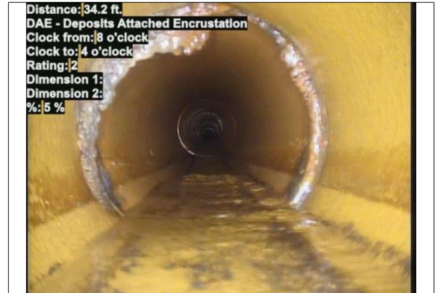
At: 34.2 ft. 8/4 DAE - Deposits Attached Encrustation Joint: No 5 %
