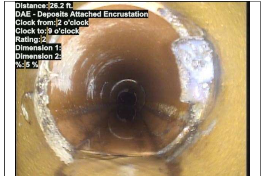
At: 26.2 ft. 2/9 DAE - Deposits Attached Encrustation Joint: No 5 %
