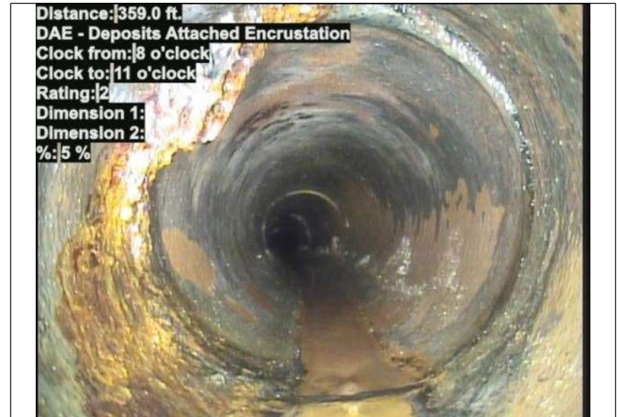
At: 359 ft. 8/11 DAE - Deposits Attached Encrustation Joint: No 5 %
