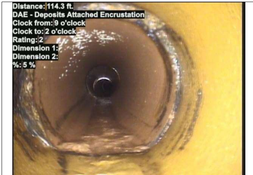
At: 114.3 ft. 9/2 DAE - Deposits Attached Encrustation Joint: No 5 %
