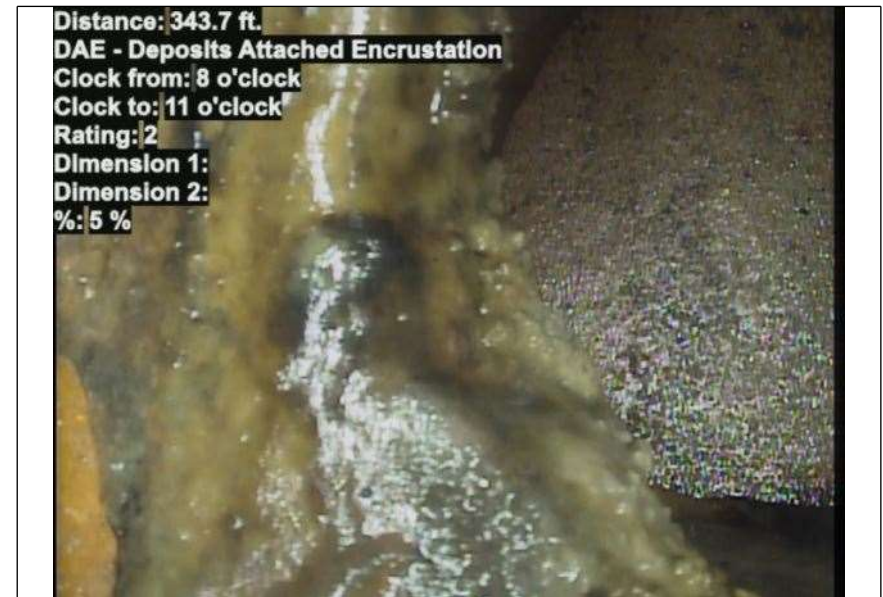
At: 343.7 ft. 8/11 DAE - Deposits Attached Encrustation Joint: No 5 %
