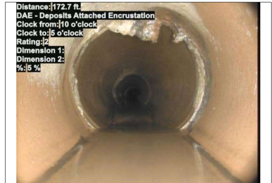
At: 172.7 ft. DAE - Deposits Attached Encrustation 10/5
