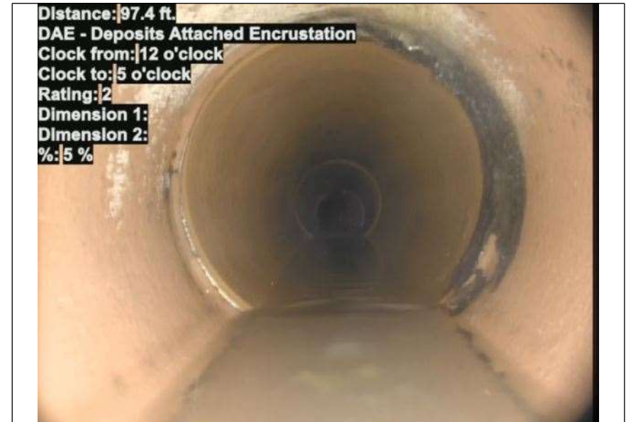
At: 97.4 ft. 12/5 DAE - Deposits Attached Encrustation Joint: No 5 %
