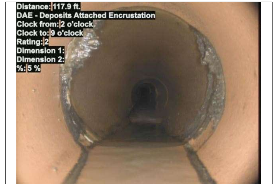
At: 117.9 ft. 2/9 DAE - Deposits Attached Encrustation Joint: No 5 %
