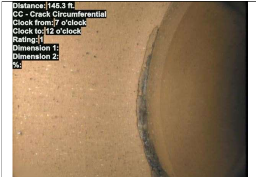
At: 145.3 ft. CC - Crack Circumferential 7/12
