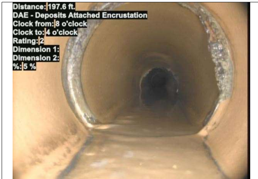
At: 197.6 ft. 8/4 DAE - Deposits Attached Encrustation Joint: No 5 %
