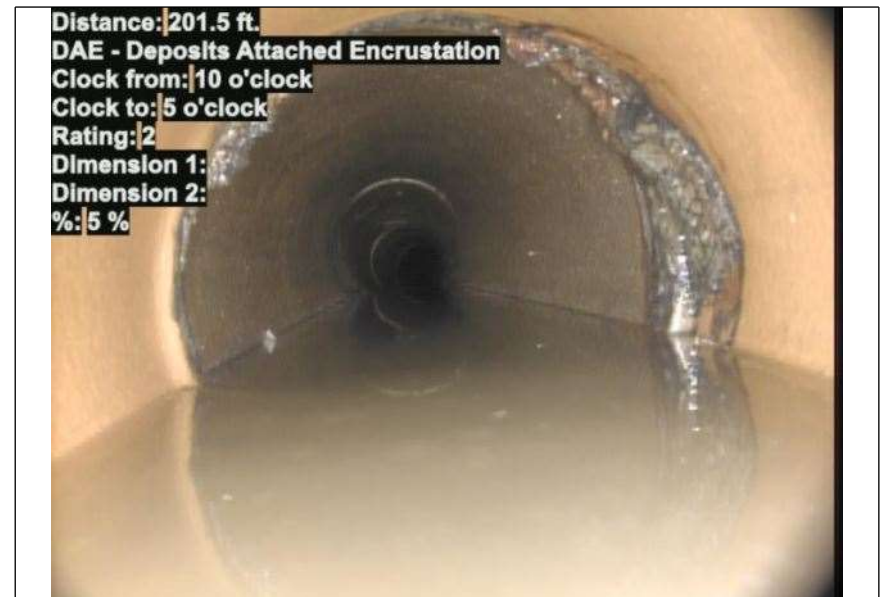
At: 201.5 ft. DAE - Deposits Attached Encrustation 10/5 Joint: No 5 %
