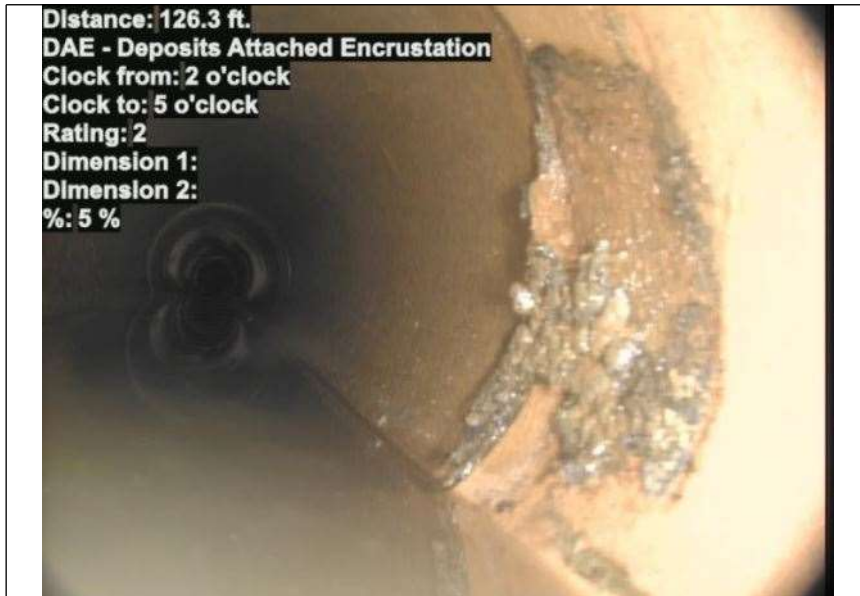
At: 126.3 ft. 2/5 DAE - Deposits Attached Encrustation Joint: No 5 %
