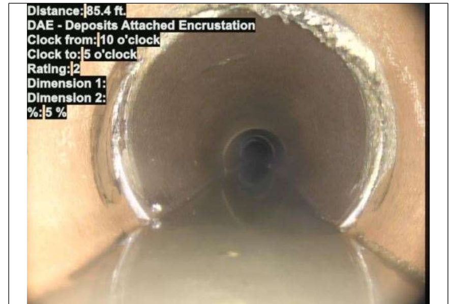
At: 85.4 ft. 10/5 DAE - Deposits Attached Encrustation Joint: No 5 %
