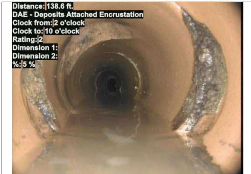
At: 138.6 ft. 2/10 DAE - Deposits Attached Encrustation Joint: No 5 %
