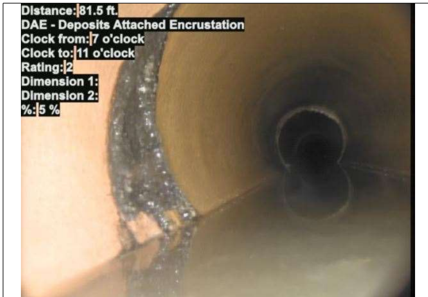
At: 81.5 ft. 7/11 DAE - Deposits Attached Encrustation Joint: No 5 %
