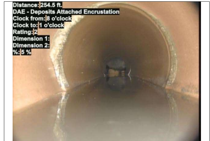
At: 254.5 ft. 8/1 DAE - Deposits Attached Encrustation Joint: No 5 %
