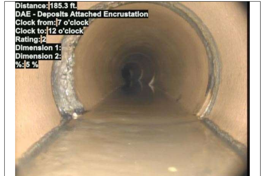
At: 185.3 ft. DAE - Deposits Attached Encrustation 7/12 Joint: No 5 %
