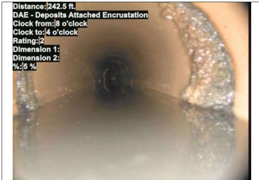
At: 242.5 ft. 8/4 DAE - Deposits Attached Encrustation Joint: No 5 %
