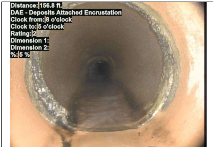
At: 156.8 ft. 8/5 DAE - Deposits Attached Encrustation
