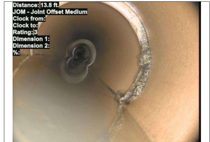
At: 13.8 ft. JOM - Joint Offset Medium Joint: No
