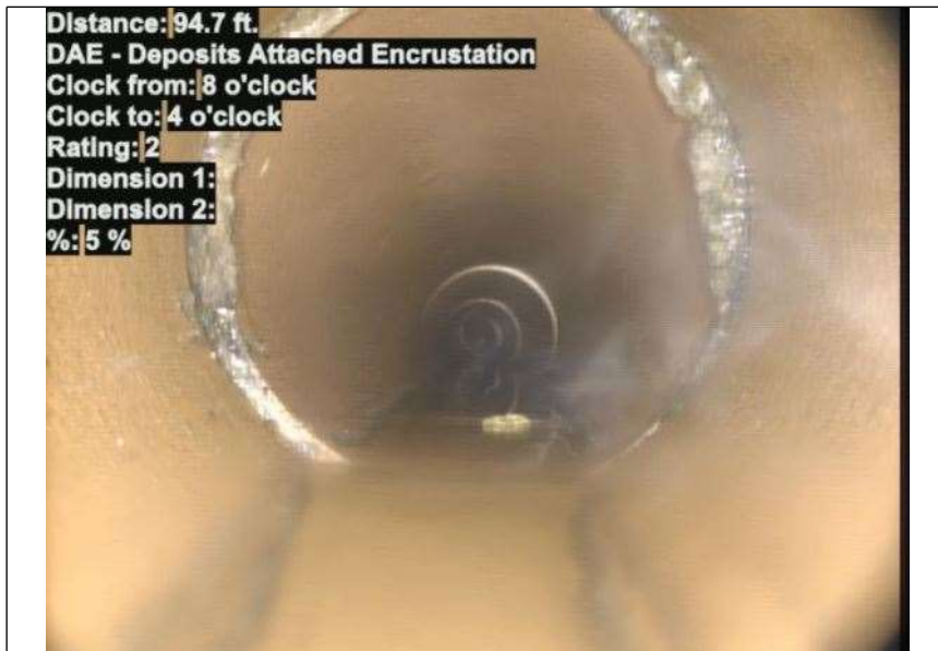
At: 94.7 ft. 8/4 DAE - Deposits Attached Encrustation Joint: No 5 %
