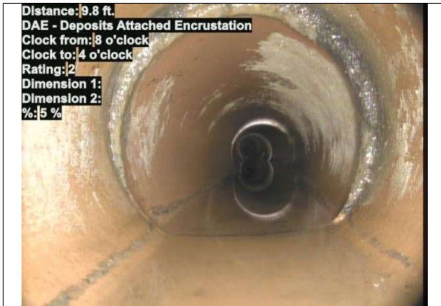
At: 9.8 ft. 8/4 DAE - Deposits Attached Encrustation Joint: No 5 %
