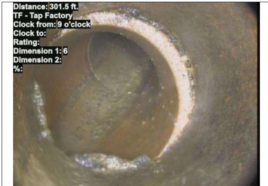
At: 301.5 ft. 9/. TF - Tap Factory Joint: No
