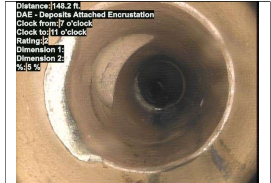
At: 148.2 ft. DAE - Deposits Attached Encrustation 7/11
