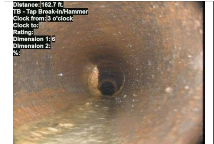
At: 162.7 ft. 3/ TB - Tap Break-in/Hammer
