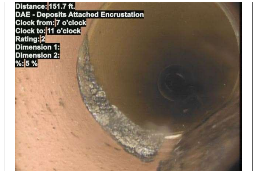
At: 151.7 ft. DAE - Deposits Attached Encrustation 7/11
