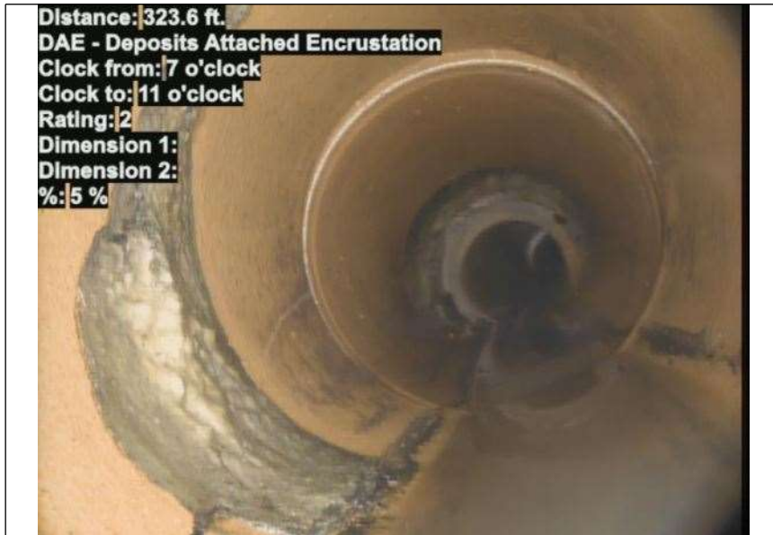
At: 323.6 ft. DAE - Deposits Attached Encrustation 7/11 Joint: No 5 %
