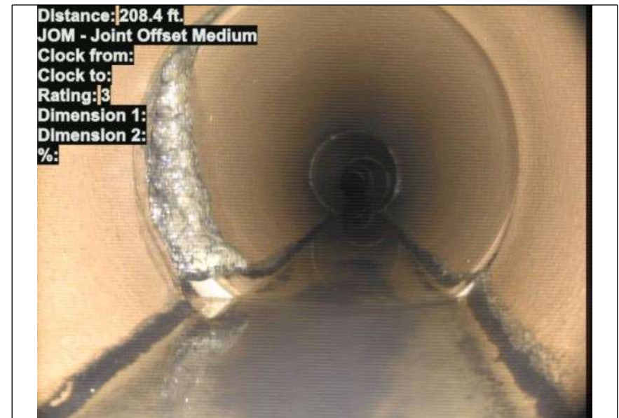
At: 208.4 ft. JOM - Joint Offset Medium Joint: No
