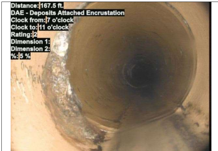
At: 167.5 ft. DAE - Deposits Attached Encrustation 7/11
