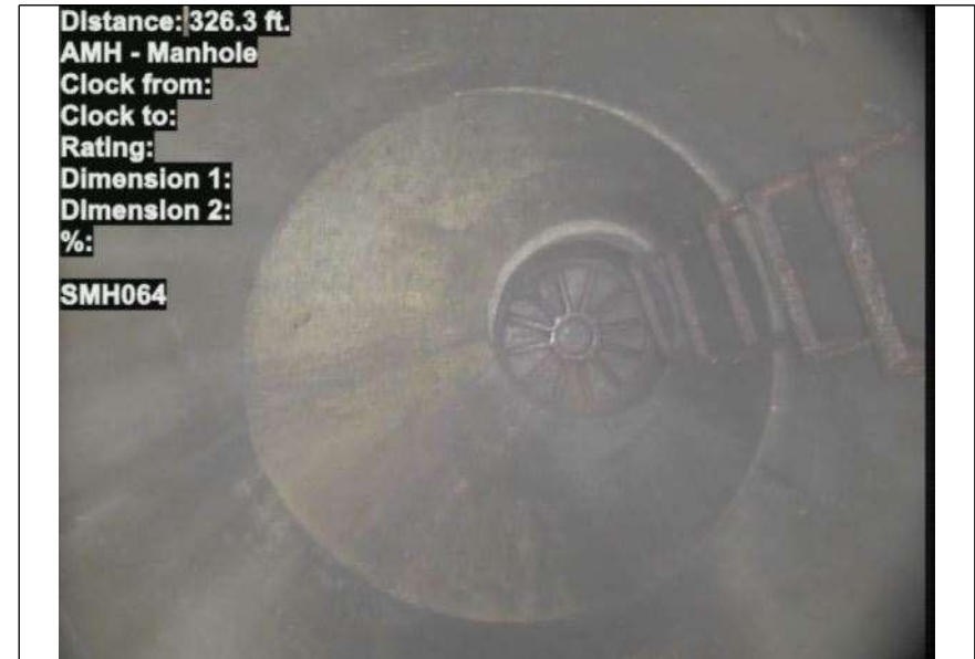
At: 326.3 ft. AMH - Manhole Joint: No SMH064
