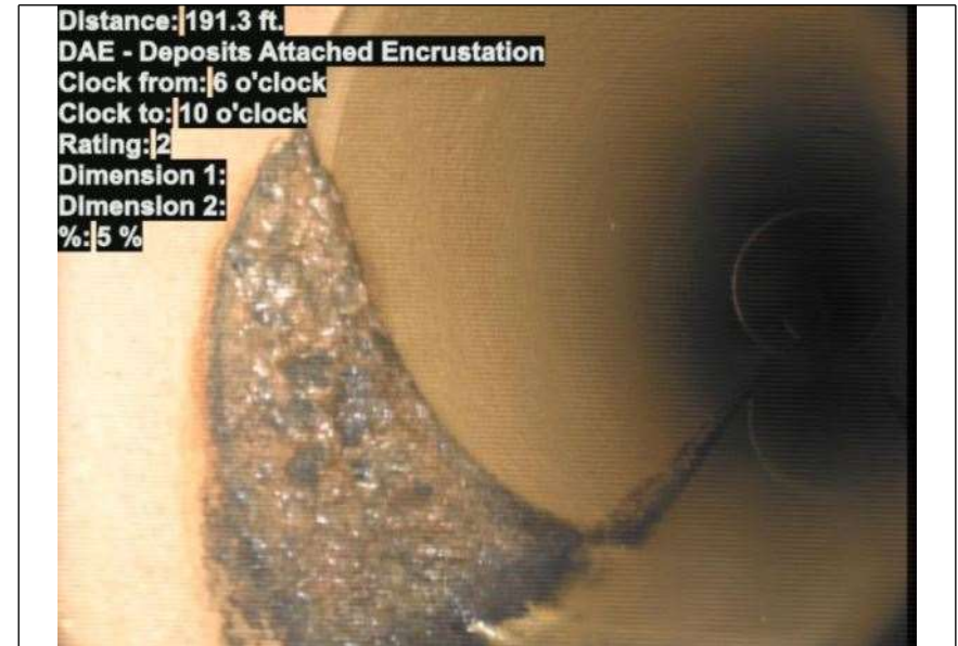
At: 191.3 ft. DAE - Deposits Attached Encrustation 6/10 Joint: No 5 %
