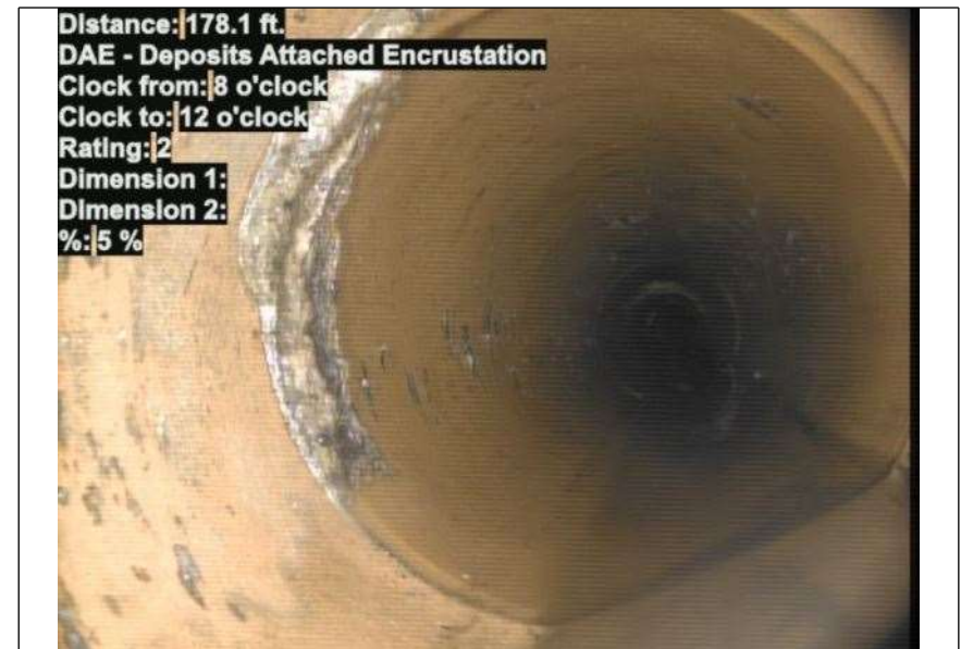
At: 178.1 ft. DAE - Deposits Attached Encrustation 8/12
