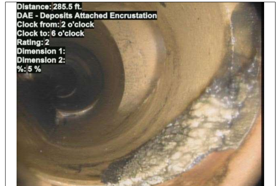
At: 285.5 ft. 2/6 DAE - Deposits Attached Encrustation Joint: No 5 %
