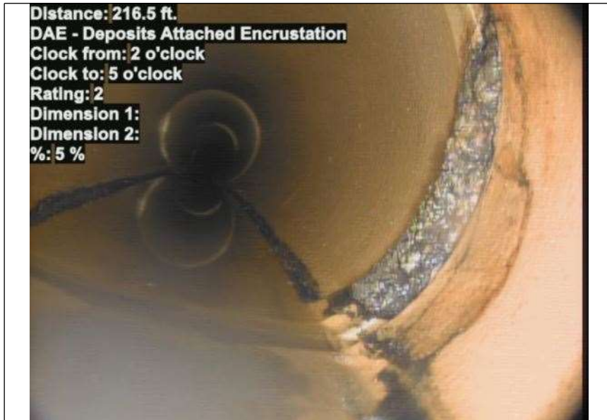
At: 216.5 ft. 2/5 DAE - Deposits Attached Encrustation Joint: No 5 %
