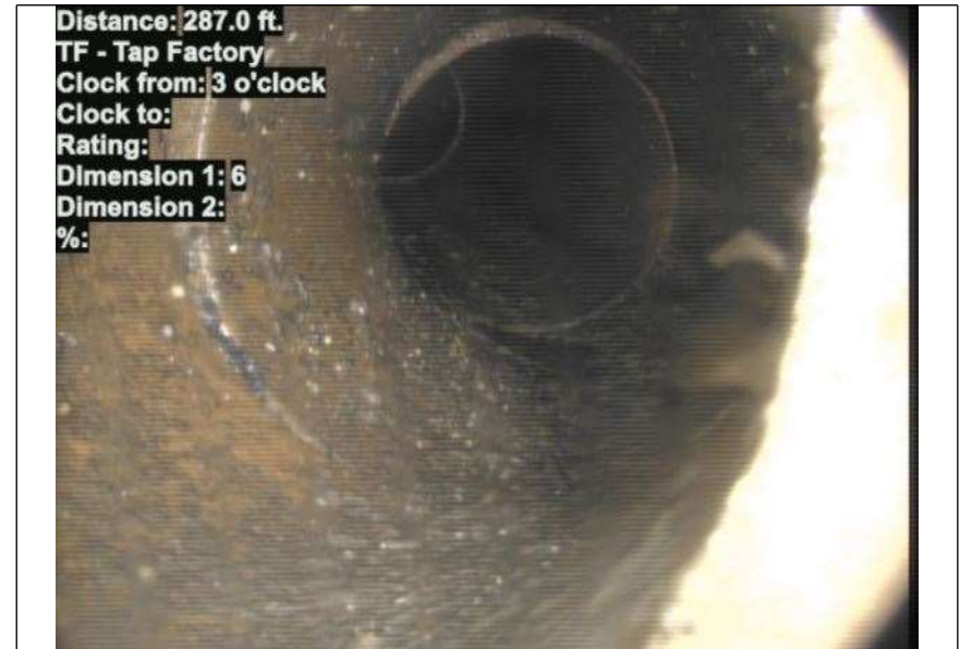
At: 287 ft. 3/. TF - Tap Factory Joint: No
