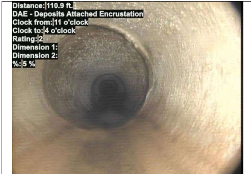
At: 110.9 ft. DAE - Deposits Attached Encrustation 11/4
