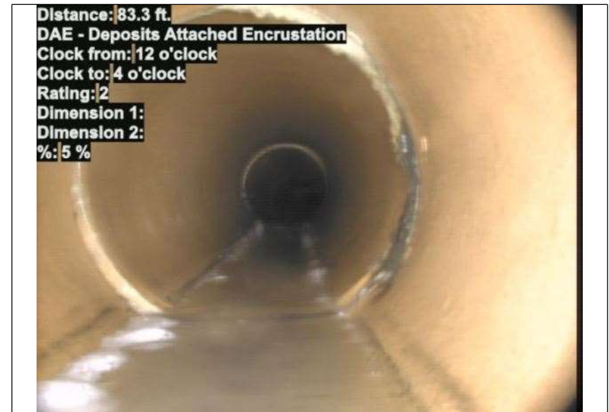
At: 83.3 ft. 12/4 DAE - Deposits Attached Encrustation Joint: No 5 %
