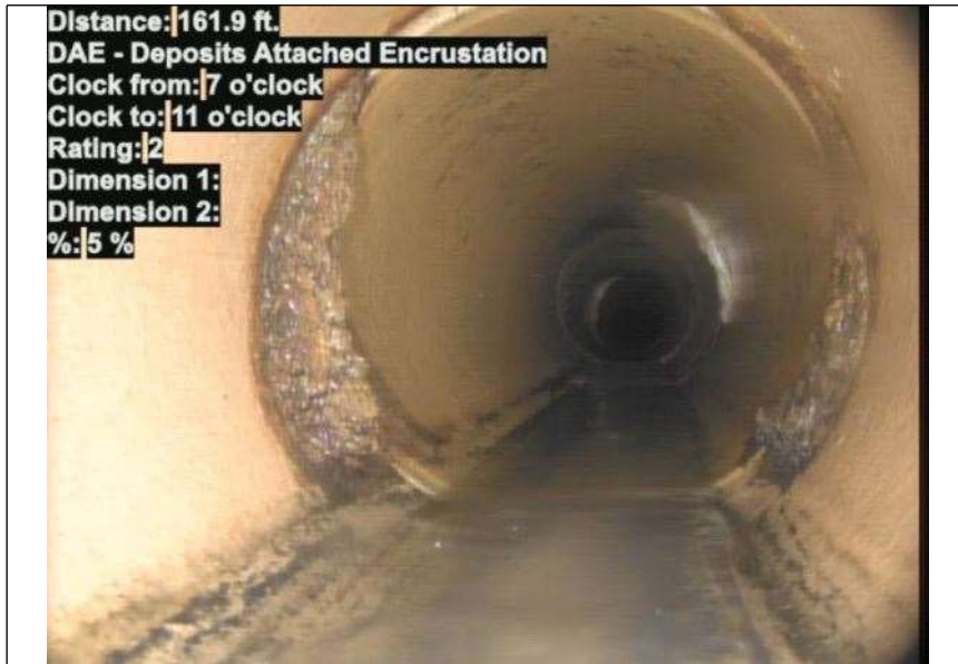
At: 161.9 ft. DAE - Deposits Attached Encrustation 7/11
