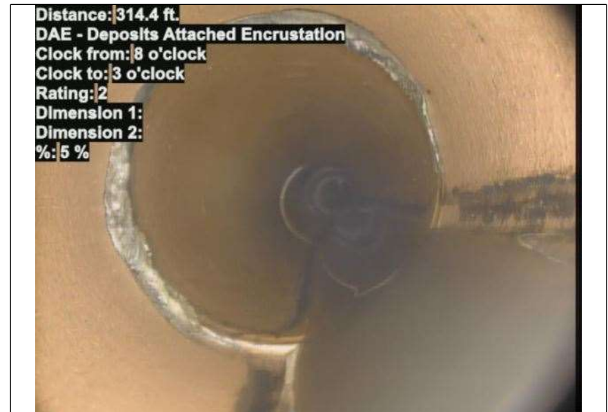
At: 314.4 ft. 8/3 DAE - Deposits Attached Encrustation Joint: No 5 %
