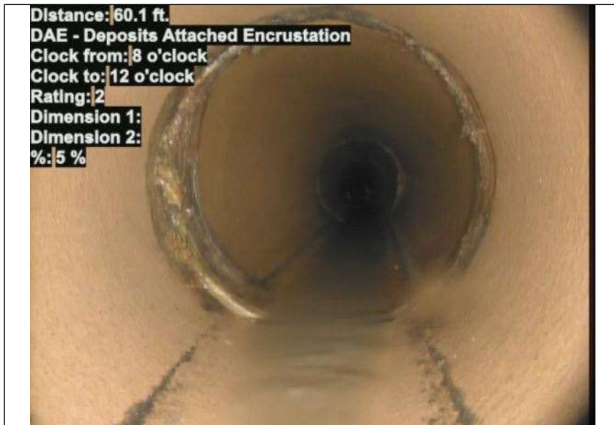
At: 60.1 ft. 8/12 DAE - Deposits Attached Encrustation Joint: No 5 %
