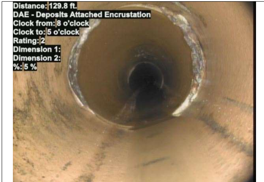
At: 129.8 ft. 8/5 DAE - Deposits Attached Encrustation Joint: No 5 %
