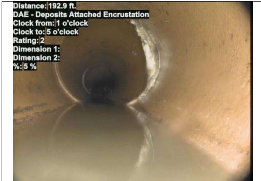
At: 192.9 ft. 1/5 DAE - Deposits Attached Encrustation Joint: No 5 %
