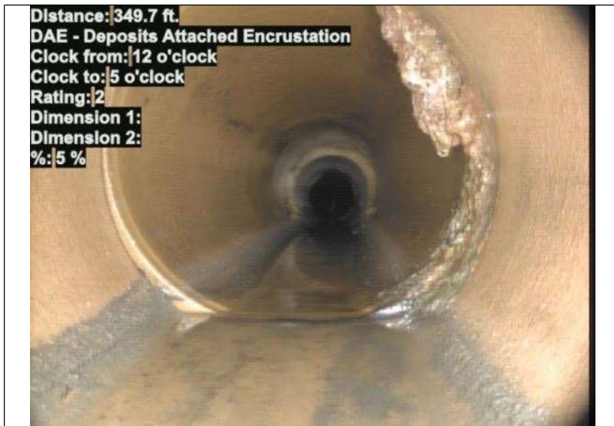
At: 349.7 ft. 12/5 DAE - Deposits Attached Encrustation Joint: Yes 5 %
