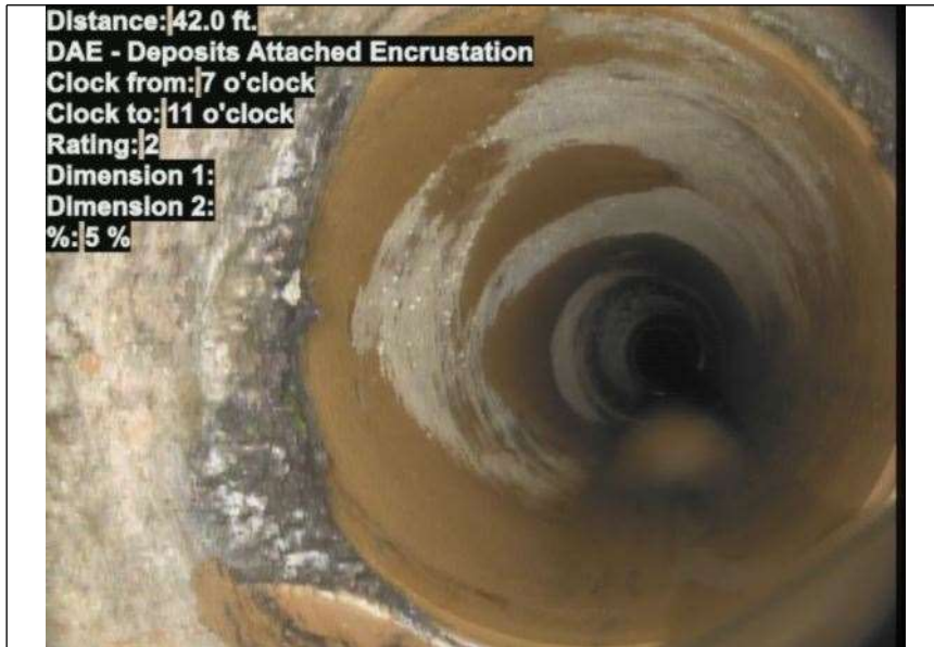
At: 42 ft. 7/11 DAE - Deposits Attached Encrustation Joint: No 5 %
