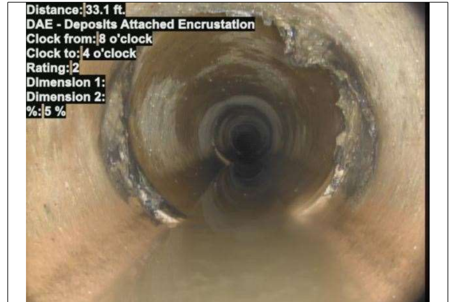
At: 33.1 ft. 8/4 DAE - Deposits Attached Encrustation Joint: No 5 %
