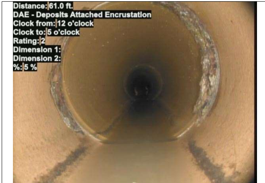
At: 61 ft. 12/5 DAE - Deposits Attached Encrustation Joint: No 5 %
