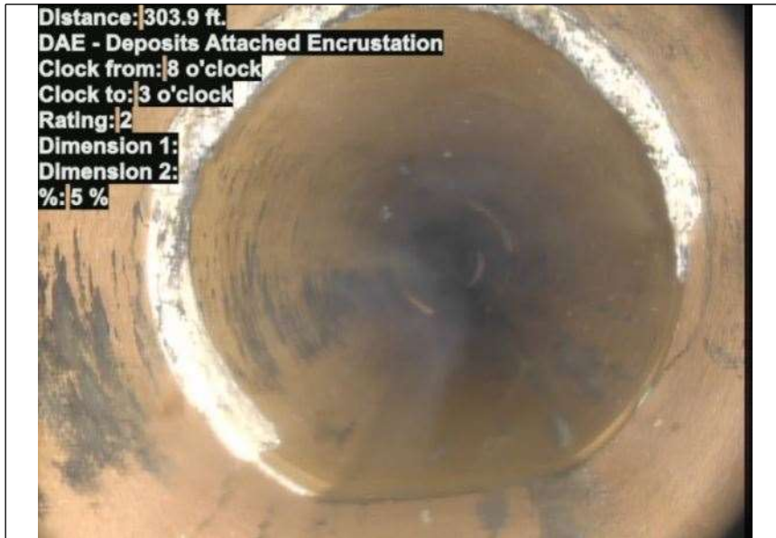
At: 303.9 ft. 8/3 DAE - Deposits Attached Encrustation Joint: No 5 %
