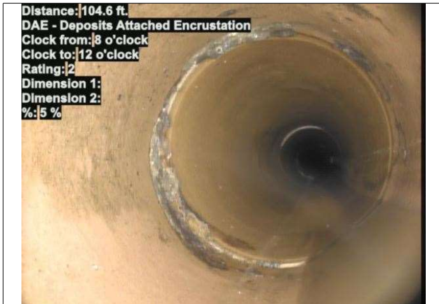
At: 104.6 ft. 8/12 DAE - Deposits Attached Encrustation Joint: No 5 %
