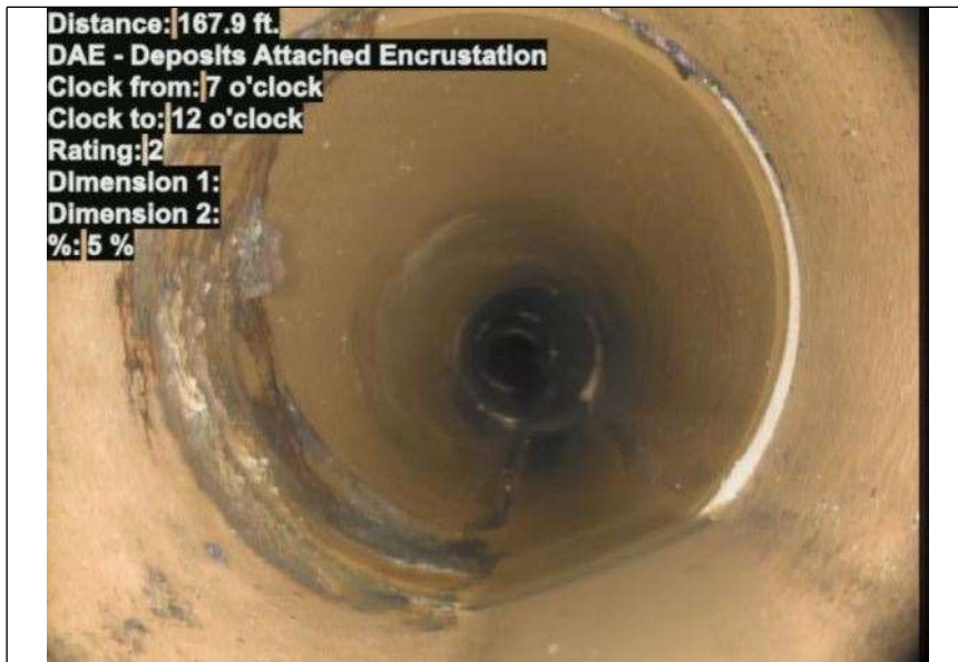
At: 167.9 ft. DAE - Deposits Attached Encrustation 7/12 Joint: No 5 %
