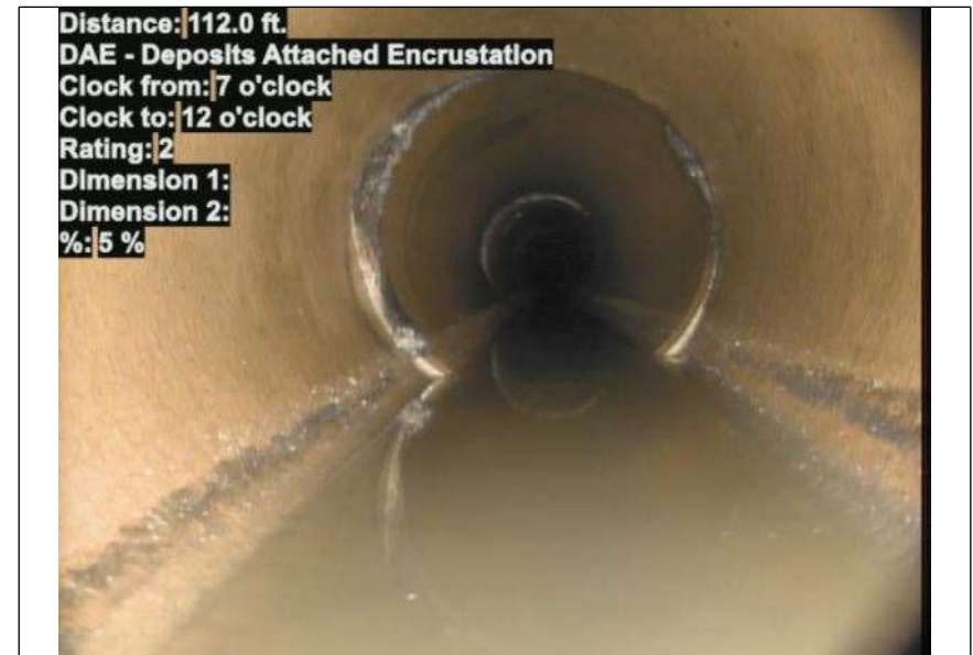
At: 112 ft. 7/12 DAE - Deposits Attached Encrustation Joint: No 5 %
