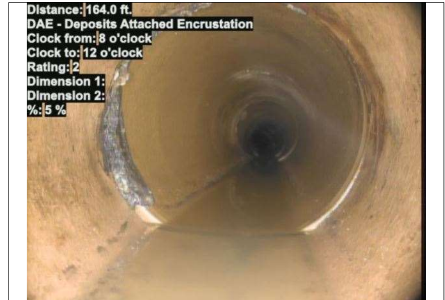
At: 164 ft. 8/12 DAE - Deposits Attached Encrustation Joint: No 5 %
