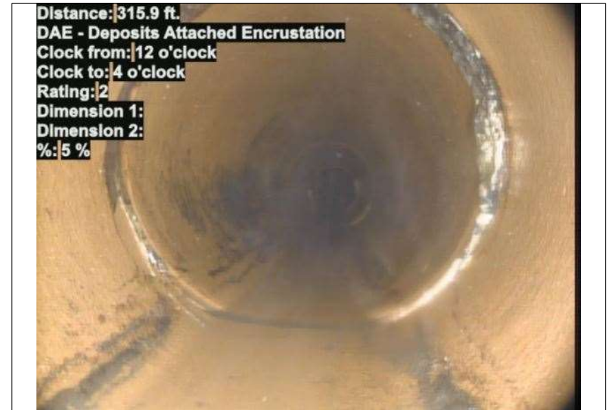
At: 315.9 ft. 12/4 DAE - Deposits Attached Encrustation Joint: No 5 %
