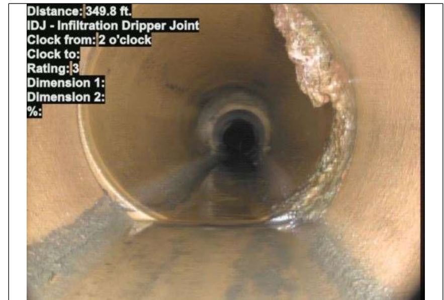
At: 349.8 ft. 2/ IDJ - Infiltration Dripper Joint Joint: Yes
