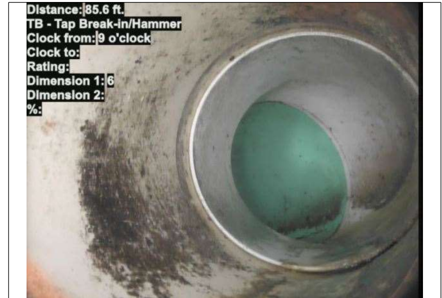
At: 85.6 ft. 9/ TB - Tap Break-in/Hammer Joint: No
