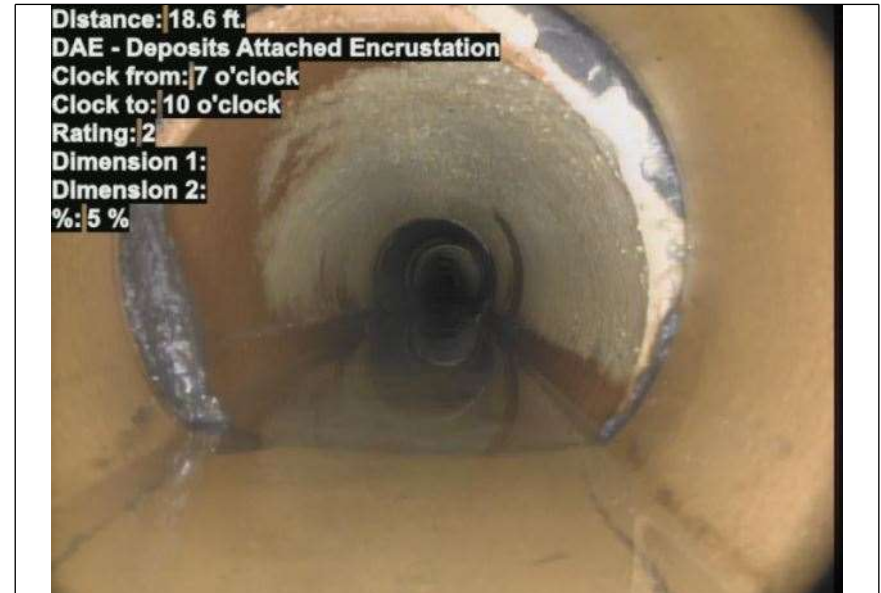
At: 18.6 ft. 7/10 DAE - Deposits Attached Encrustation Joint: No 5 %
