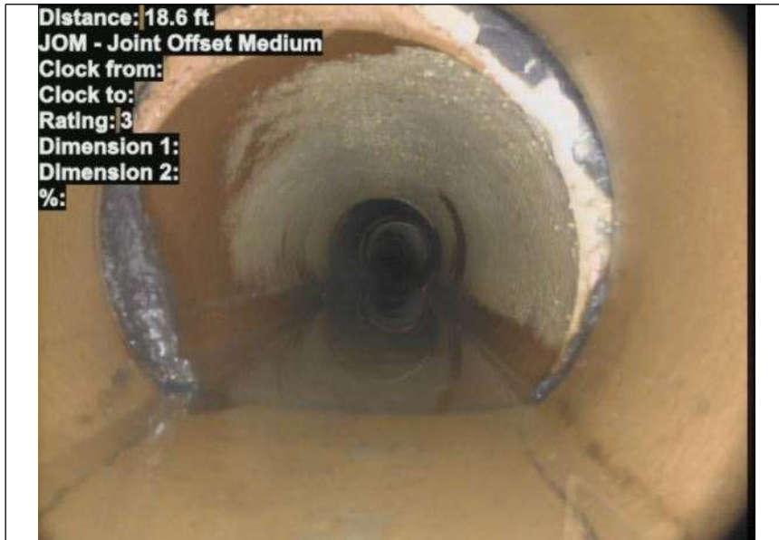
At: 18.6 ft. JOM - Joint Offset Medium Joint: No
