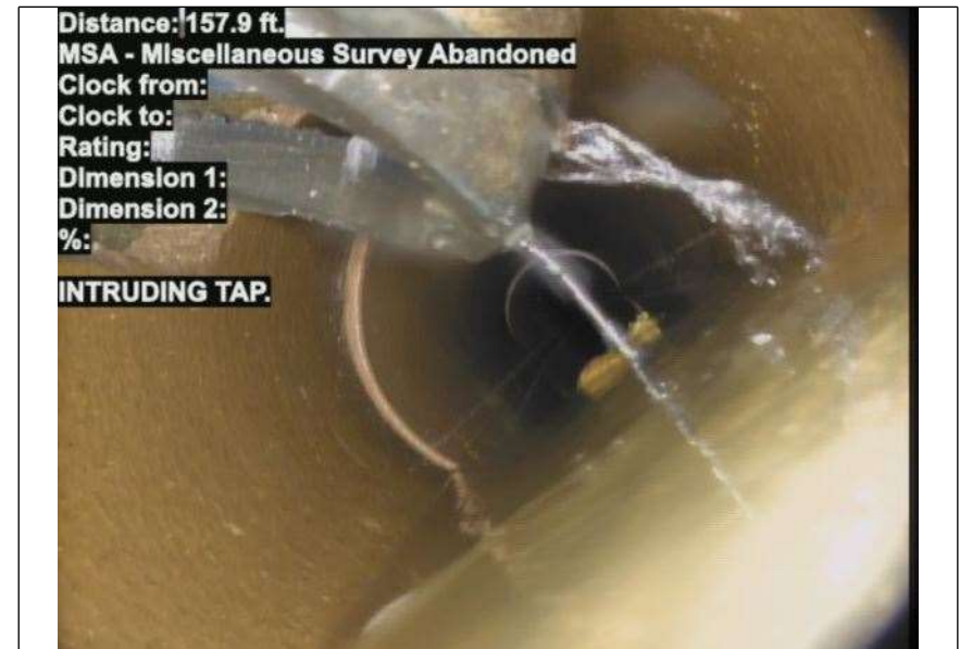
At: 157.9 ft. MSA - Miscellaneous Survey Abandoned Joint: No INTRUDING TAP.
