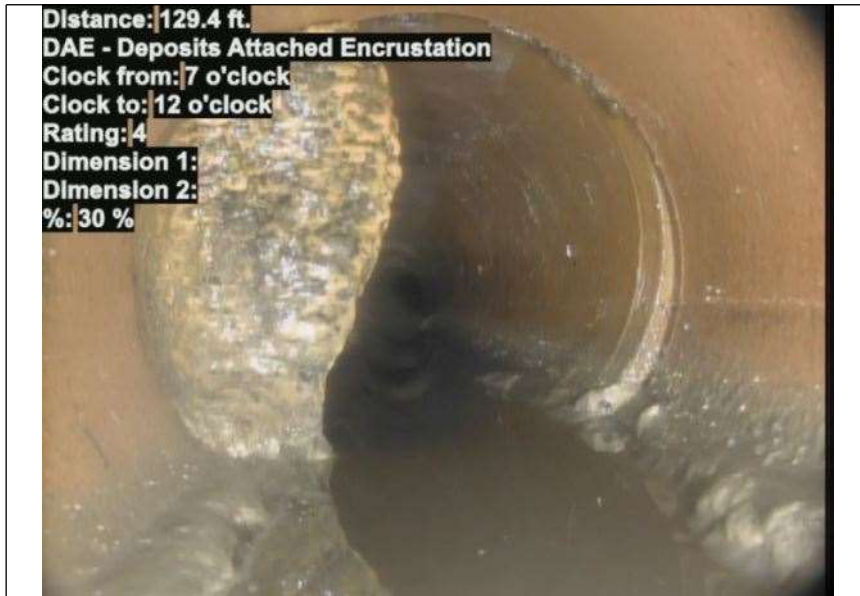
At: 129.4 ft. DAE - Deposits Attached Encrustation 7/12
