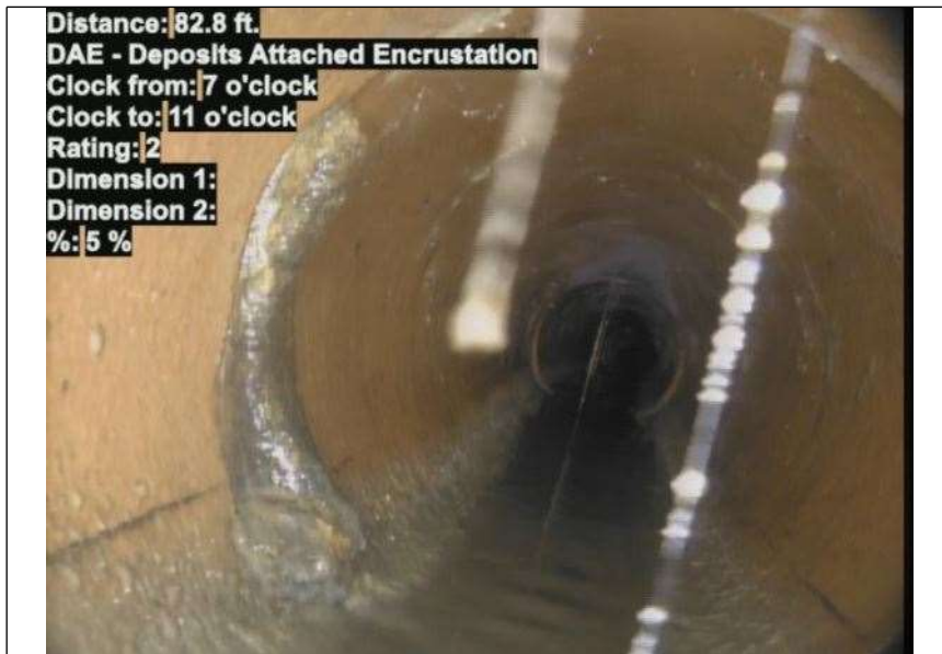
At: 82.8 ft. 7/11 DAE - Deposits Attached Encrustation Joint: No 5 %
