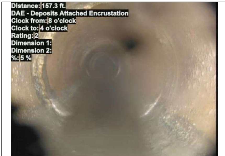
At: 157.3 ft. 8/4 DAE - Deposits Attached Encrustation
