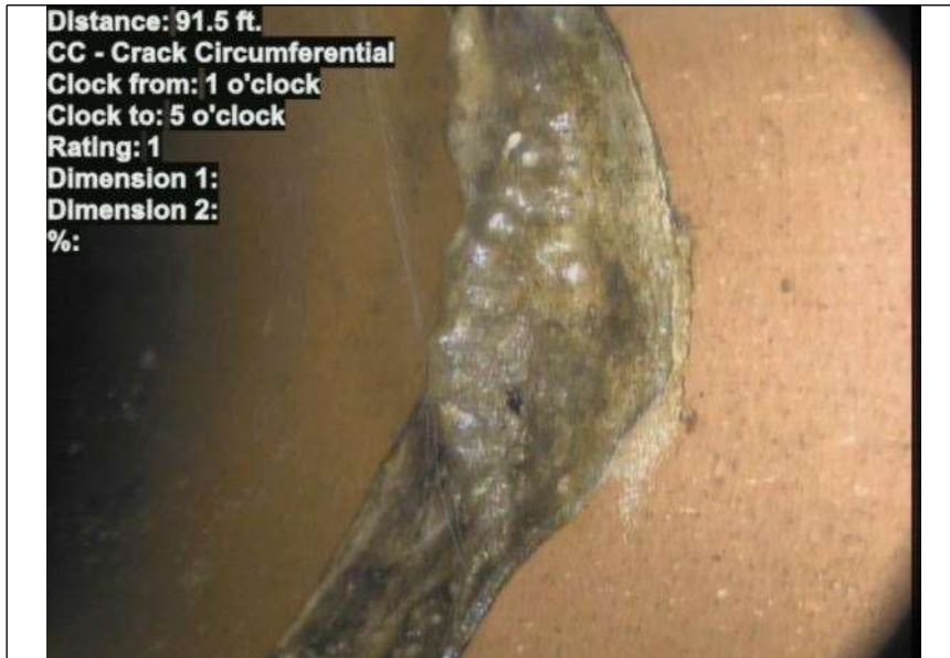
At: 91.5 ft. 1/5 CC - Crack Circumferential Joint: No
