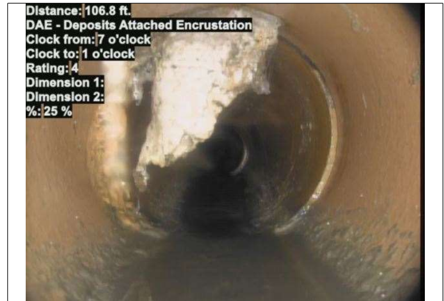
At: 106.8 ft. 7/1 DAE - Deposits Attached Encrustation Joint: No 25 %
