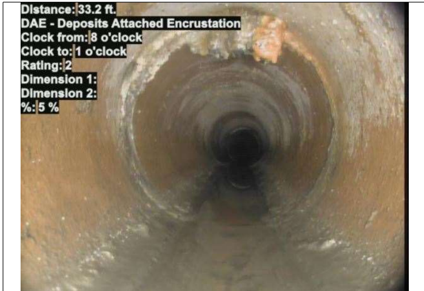
At: 33.2 ft. 8/1 DAE - Deposits Attached Encrustation Joint: No 5 %
