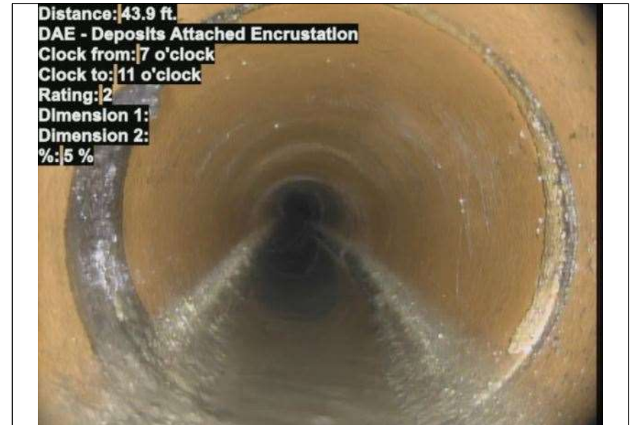
At: 43.9 ft. 7/11 DAE - Deposits Attached Encrustation Joint: No 5 %
