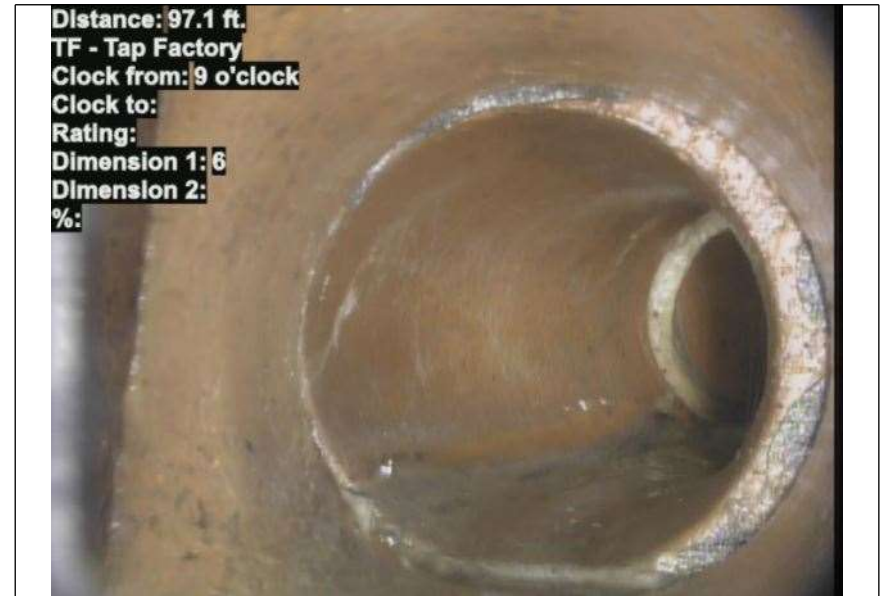
At: 97.1 ft. 9/ TF - Tap Factory Joint: No
