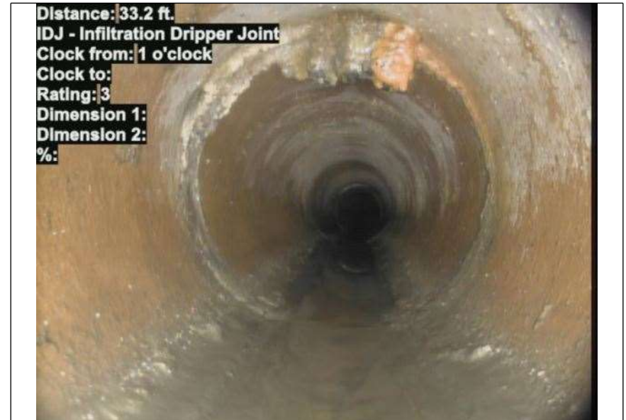
At: 33.2 ft. 1/. IDJ - Infiltration Dripper Joint Joint: Yes
