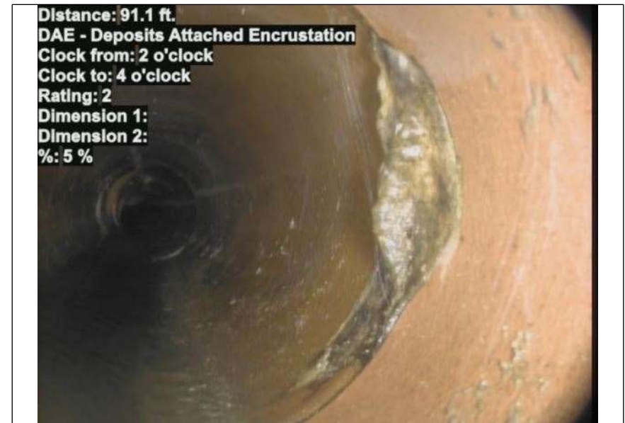
At: 91.1 ft. 2/4 DAE - Deposits Attached Encrustation Joint: No 5 %
