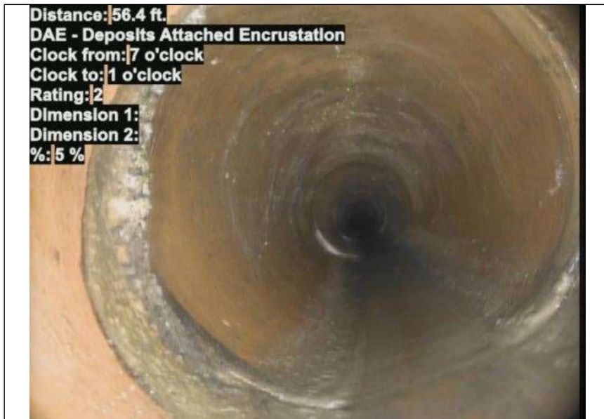
At: 56.4 ft. 7/1 DAE - Deposits Attached Encrustation Joint: No 5 %
