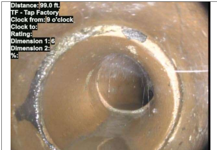
At: 99 ft. 9/ TF - Tap Factory Joint: No
