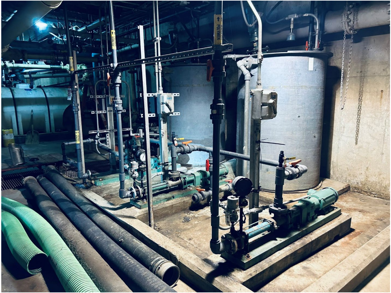
Existing Poly Feed Pumps P17, P18, P19 & Aging Tank. Located in the Basement
