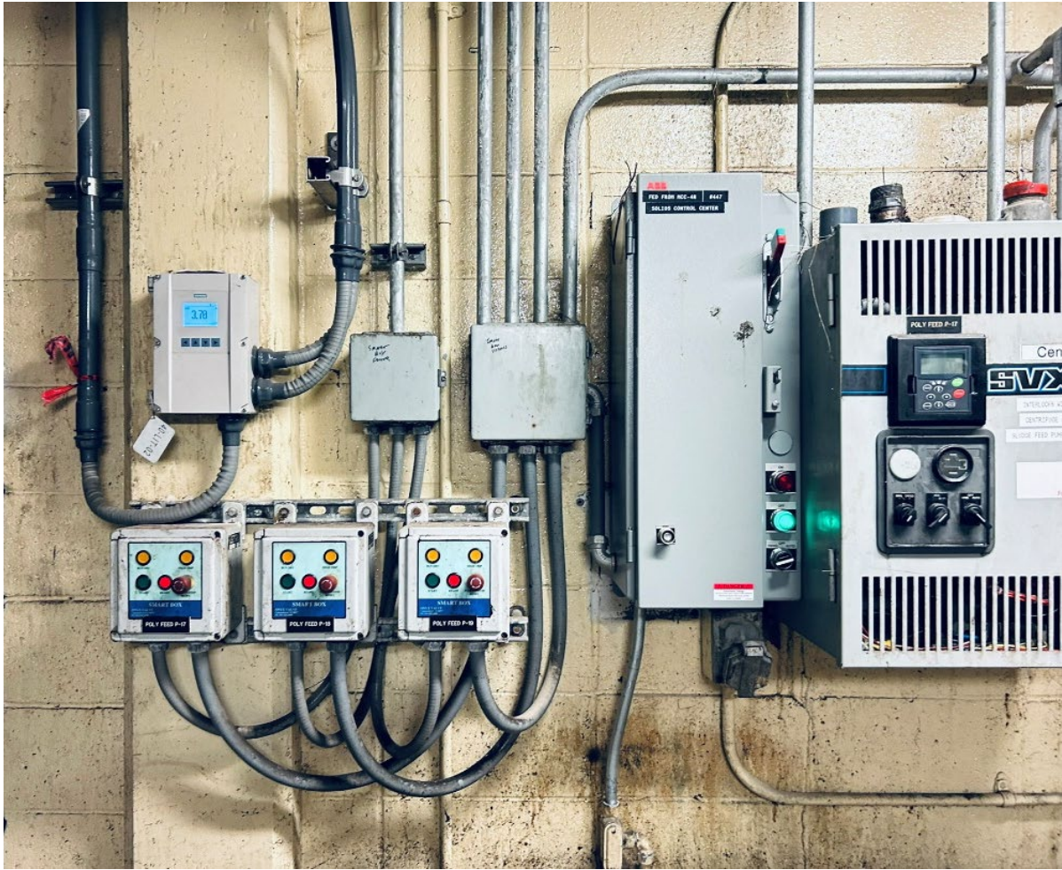
Existing Poly Feed Pumps P17, P18, P19 & Smart Boxes. Located on the 1st Floor Polymer Room
