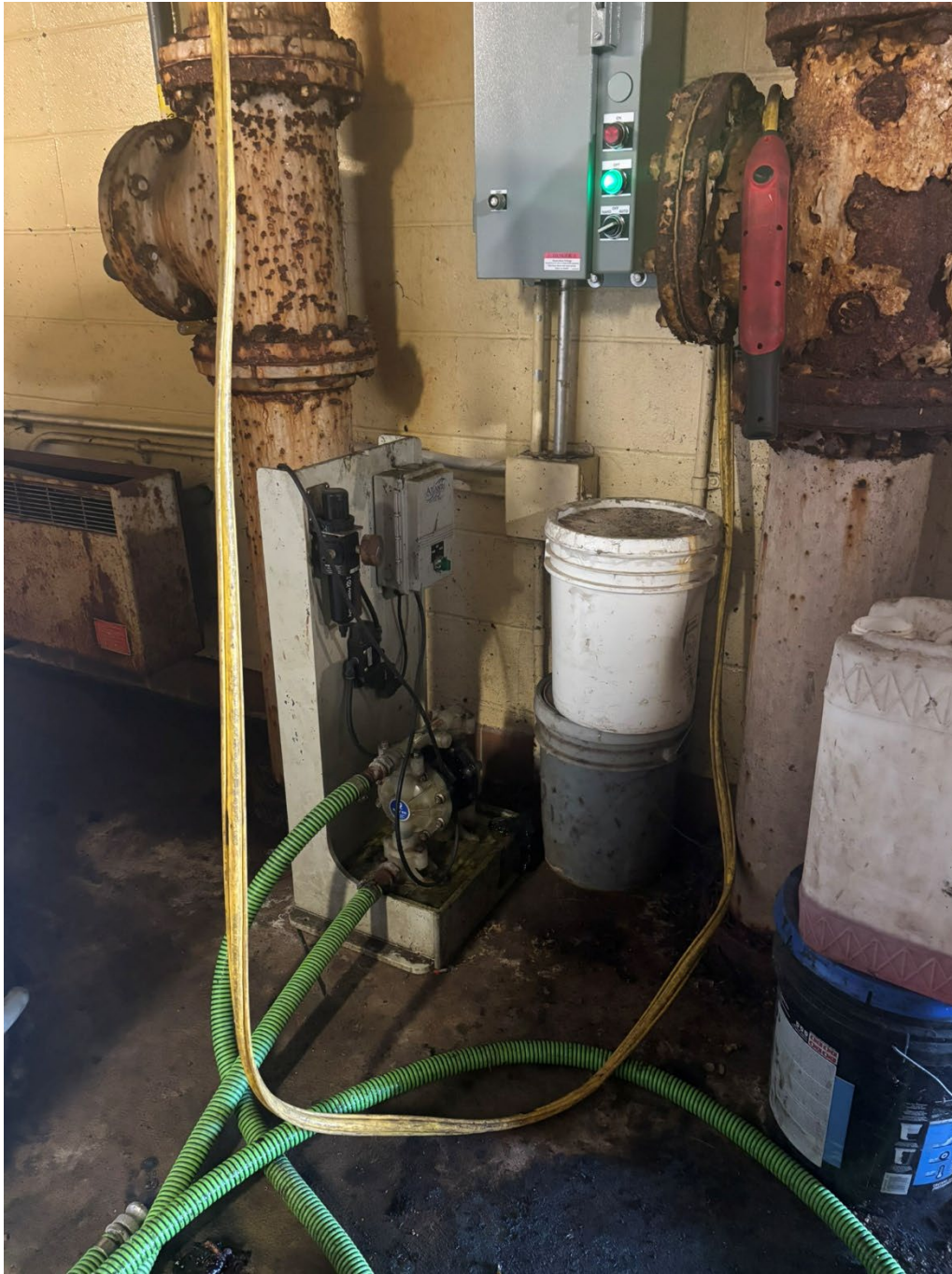
Existing Polymer Tote Transfer Pump. Located on the 1st Floor, Polymer Room
