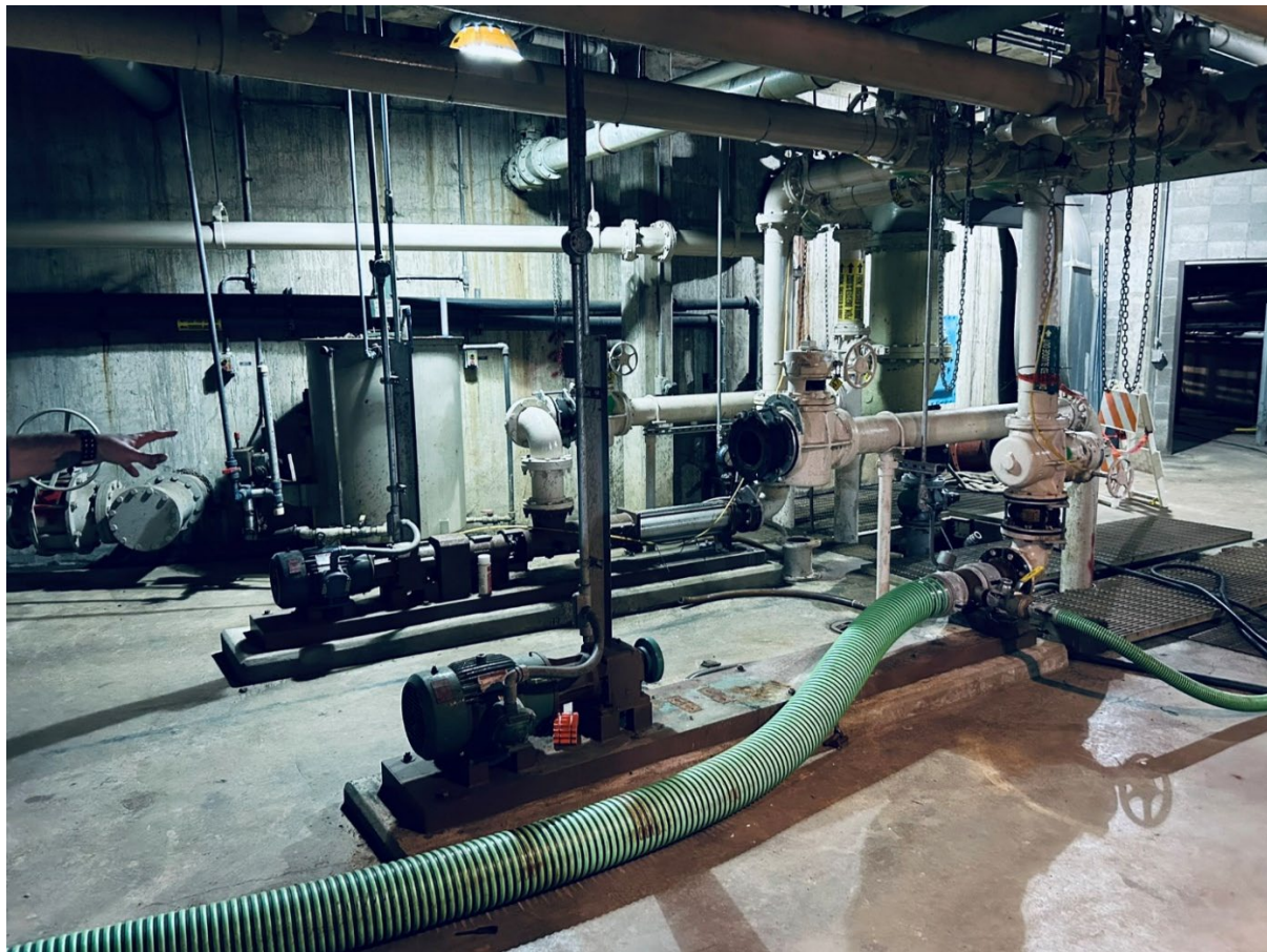
Existing Progressive Cavity Sludge Pumps P11 & P12. Located in the basement.
