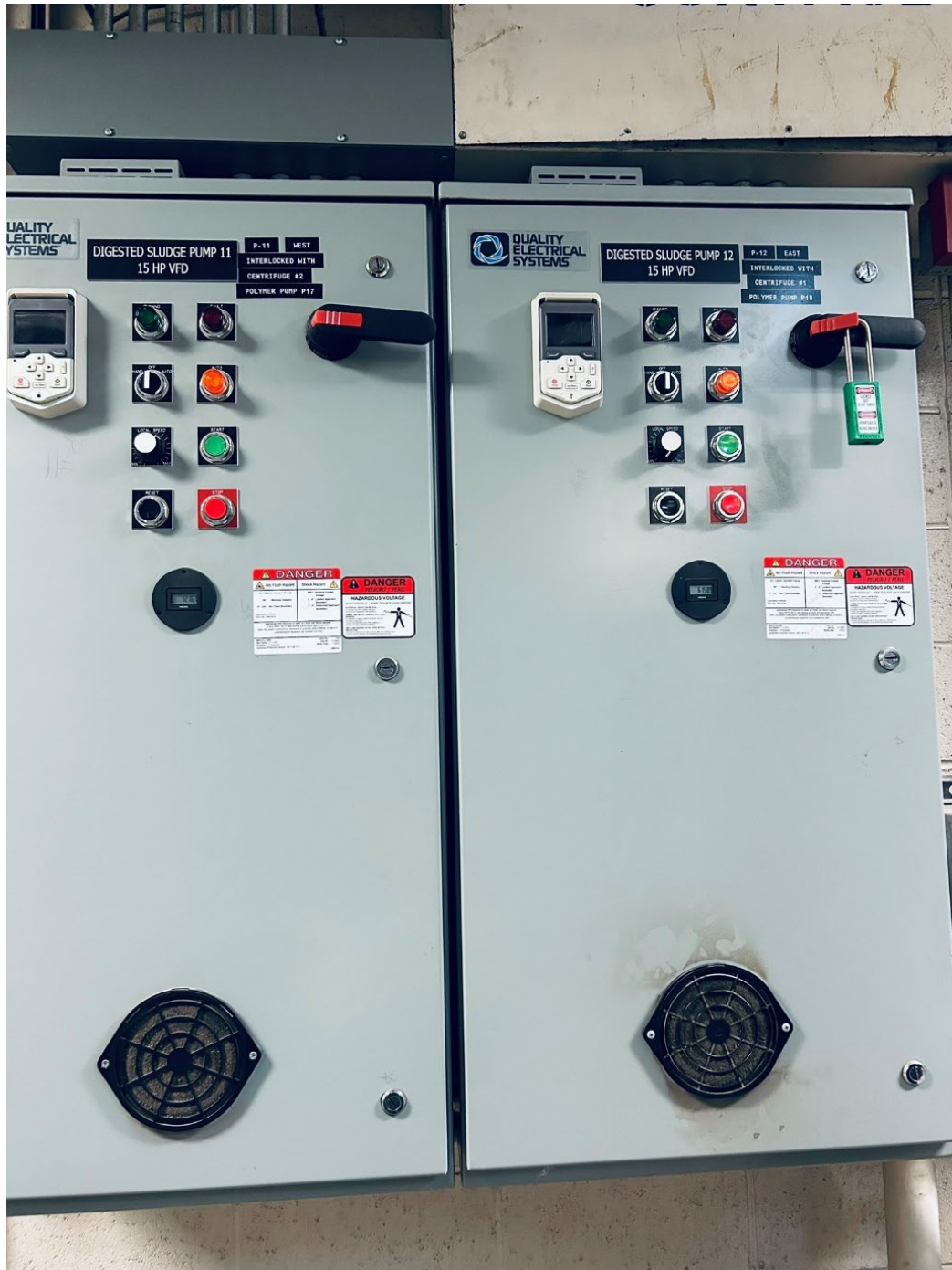
Existing Sludge Pumps P11 & P12 Local Control Panels with ABB 15HP VFDs. Located on the first floor, in the Electrical Room.
