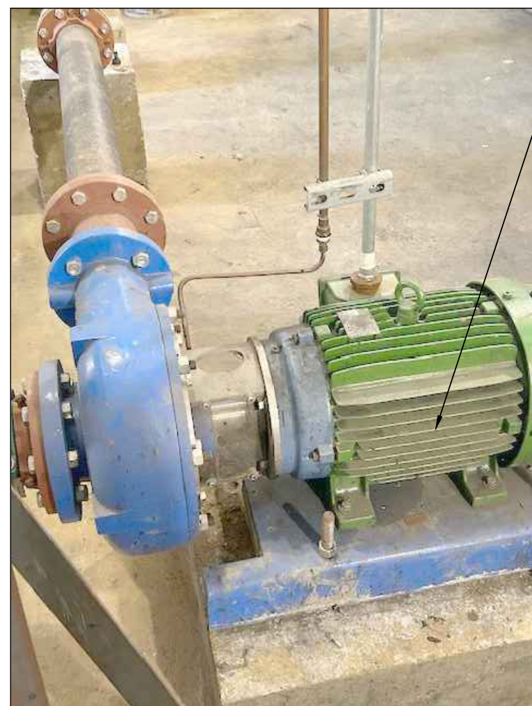
SLUDGE FEED PUMP No. 2 DISC FLOW PUMP TO BE SALVAGED AND TURNED OVER TO THE OWNER
