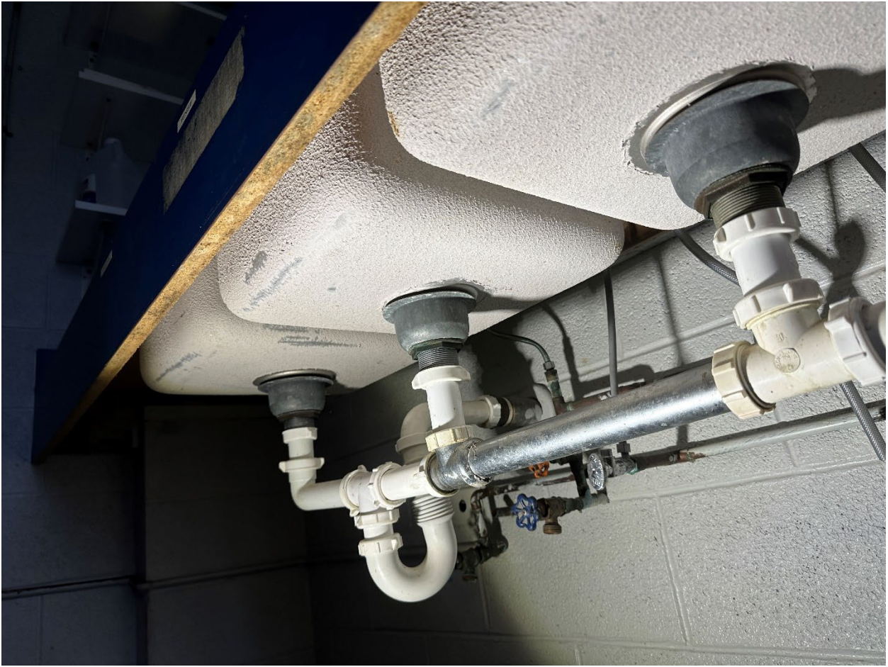
Photo 4 – View of the sink undercoating found on three (3) of the four (4) sinks in the concession stand portion of the L-shaped building.
